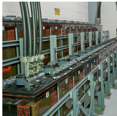
Battery Rack at Nuclear Plant
