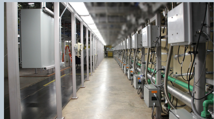
Top: Ground floor view of the HALEU cascade.
