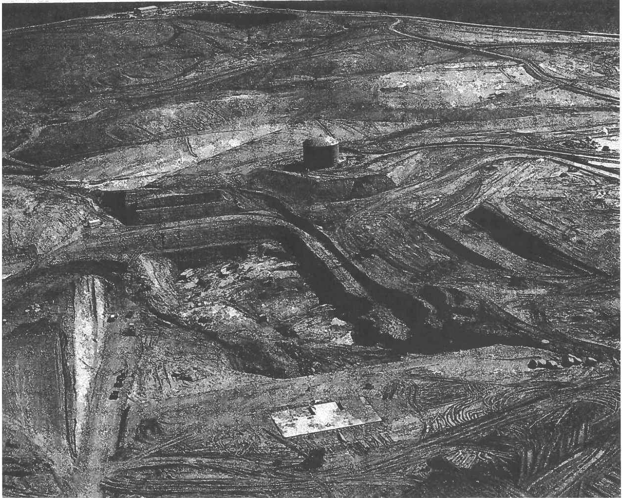
Figure E3.8-6 General Overview Construction Photograph of VCSNS Site During Construction, Showing Excavation and Disturbance, February 1974
