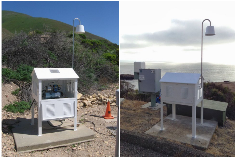
DCPD air sampling station equipment
