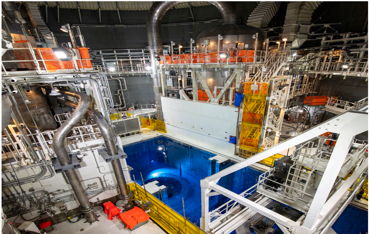
Photo of the Vogtle Unit 3 reactor cavity area. Photo courtesy of Georgia Power Company.
