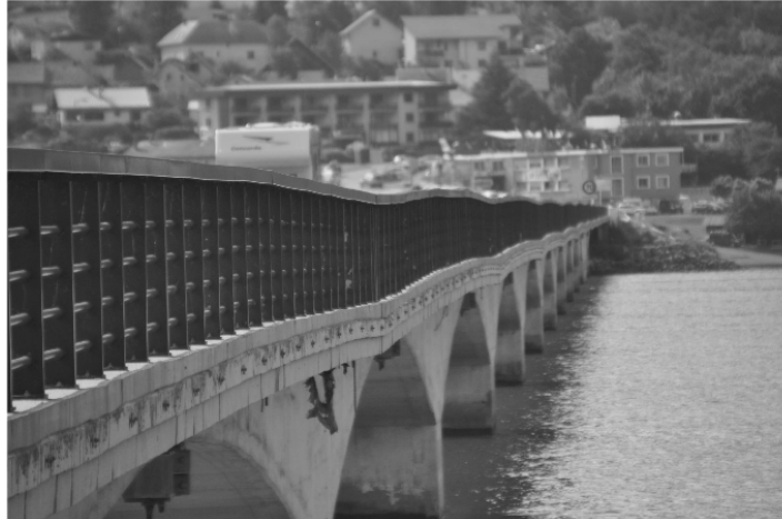
Figure 2-18 Present-day view of the Savines Bridge in France. (Sellin, Barthélémy, Bondonet, & Cauvin, 2015)
