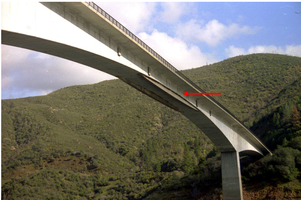
Figure 2-23 Brace installed on Parrotts Ferry Bridge (indicated by arrow) more than 10 years after construction to support the center. (HighestBridges.com, 2009)
