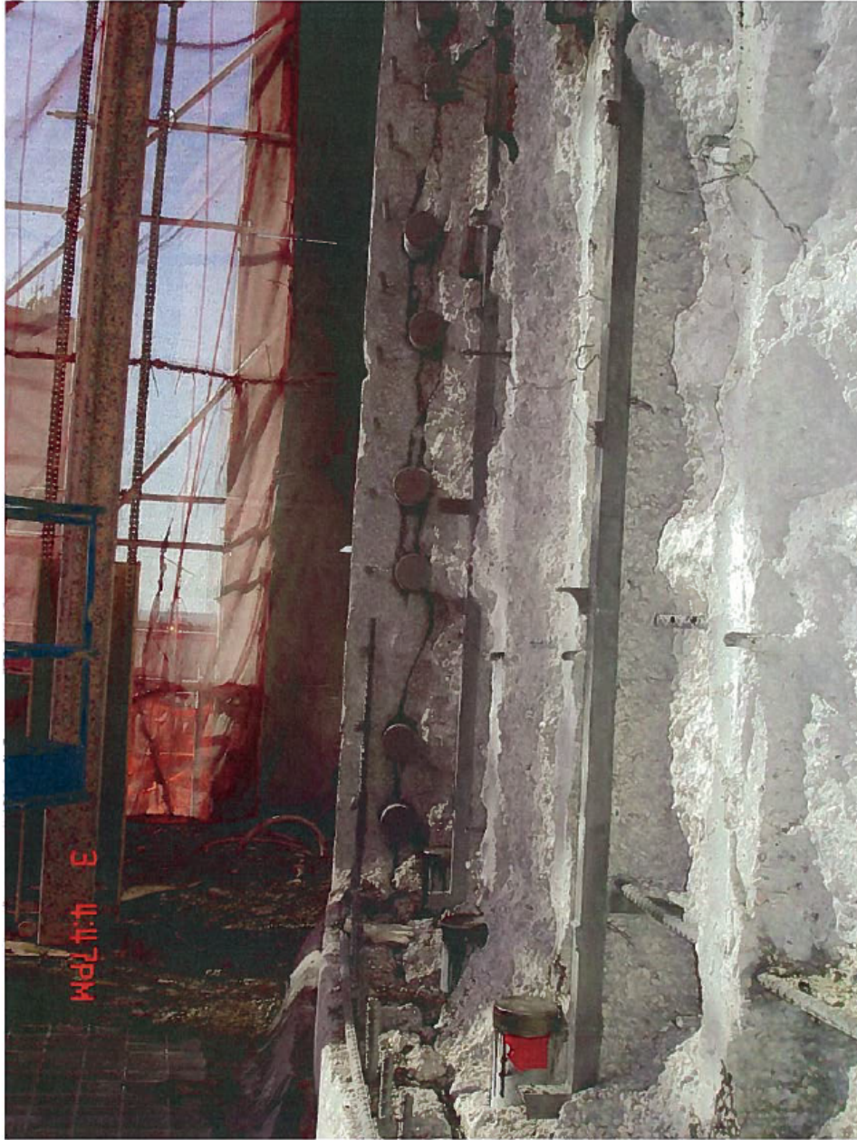
Figure 2-27 Photograph of delamination crack running from horizontal tendon to horizontal tendon, parallel to the wall surface, approximately 10 inches from the exterior surface of the concrete. (US Nuclear Regulatory Commission, 2010)
