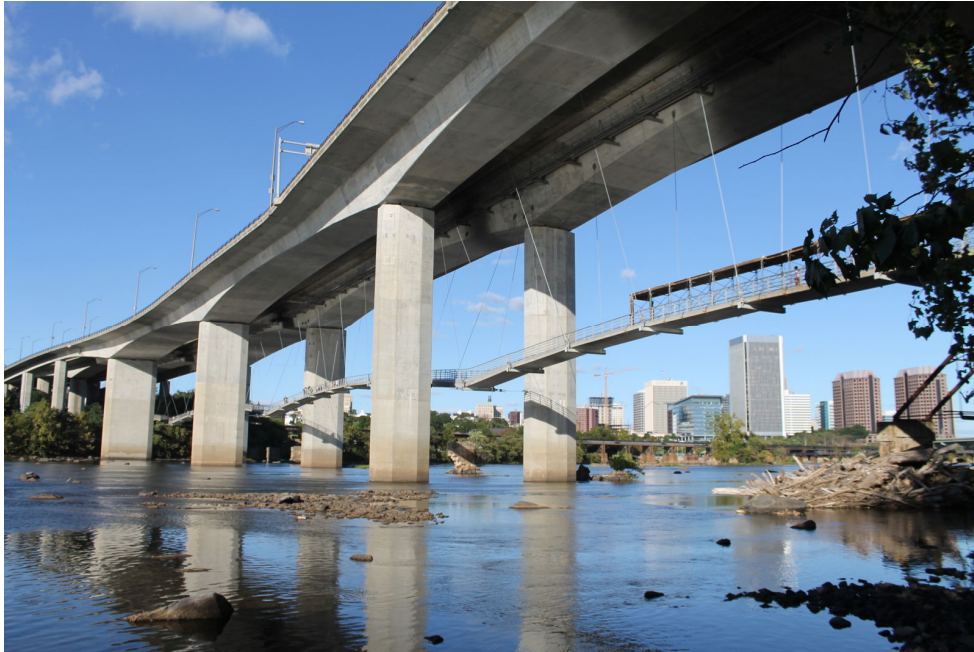
Figure 2-24 Robert E. Lee Memorial Bridge in Richmond, VA. Photograph shows the piers, underside, and pedestrian suspension bridge. (BridgeHunter.com, 2017)
