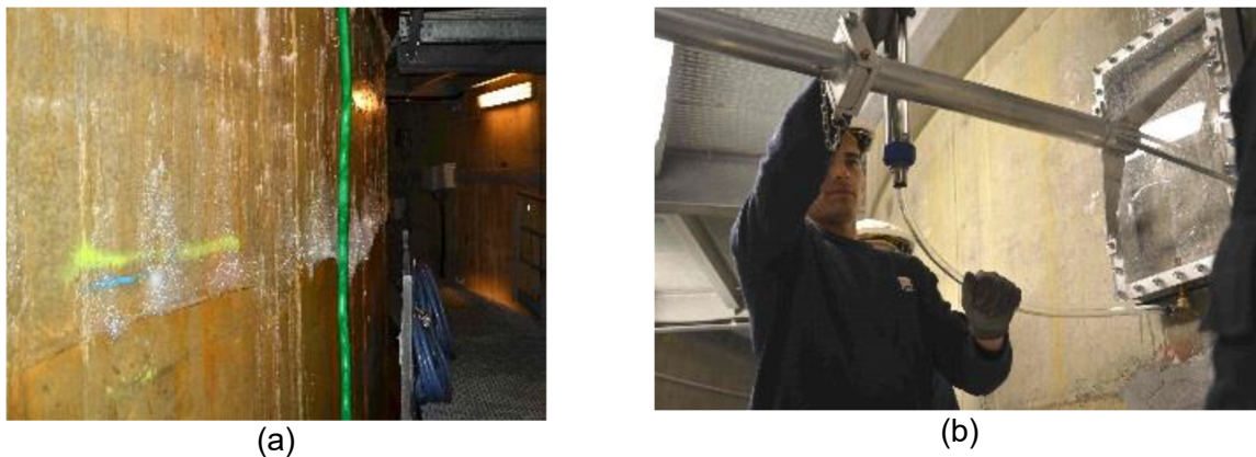
Figure 4-11 (a) Leaking zones revealed by soap bubbling. (b) Flow rate measurement with collecting box and flowmeter. (Henault, et al., 2018)
