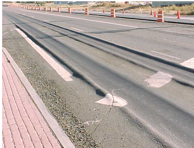
Figure 2-3 Asphalt pavement rutting on a primary highway. (Pavement Tools Consortium, n.d.)
