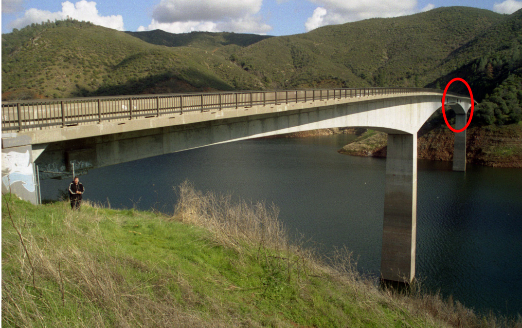
Figure 2-21 Parrotts Ferry Bridge showing deflection at midspan (inside the red circle). (HighestBridges.com, 2009)
