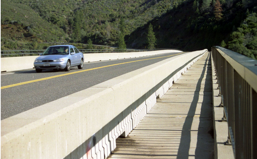
Figure 2-22 Parrotts Ferry Bridge with a nearly 2-foot (61 cm) sag in the center. (HighestBridges.com, 2009)
