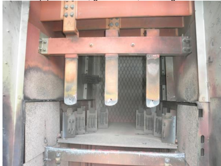
(b) Bus bars (melted metal slugs circled in red)
