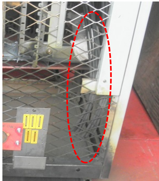
Figure 2.8-8 DP Test 7 Interior Cable Bundle Damage
