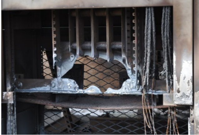
(a) Rear View Shows Plate Damage
