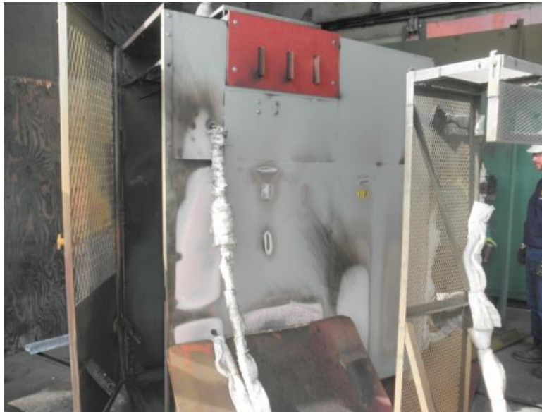
Figure 3.11-4 SWGR Test 9 Exterior Damage
