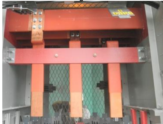
Figure 3.4-2 SWGR Bus Bar and Top Vent Configuration
