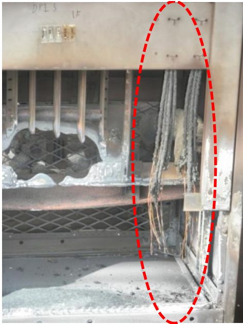
(a) In-situ damage
