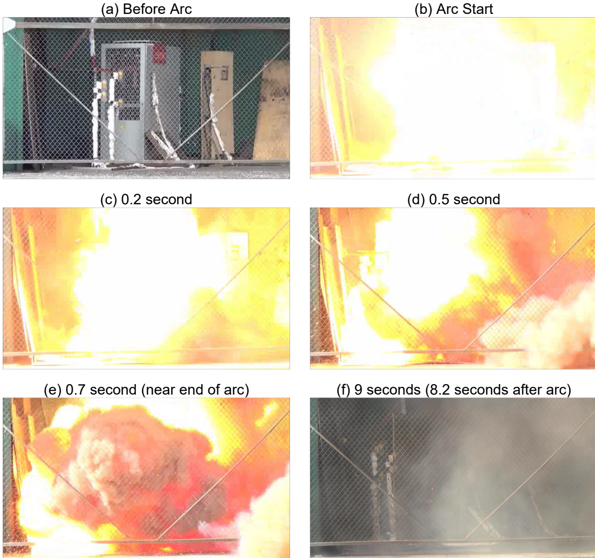
Figure 3.12-1 SWGR Test 10 Arc
