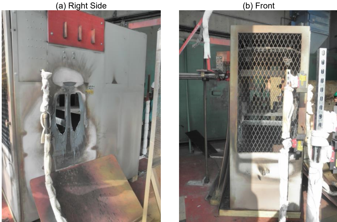
Figure 3.8-4 SWGR Test 7 Exterior Damage
