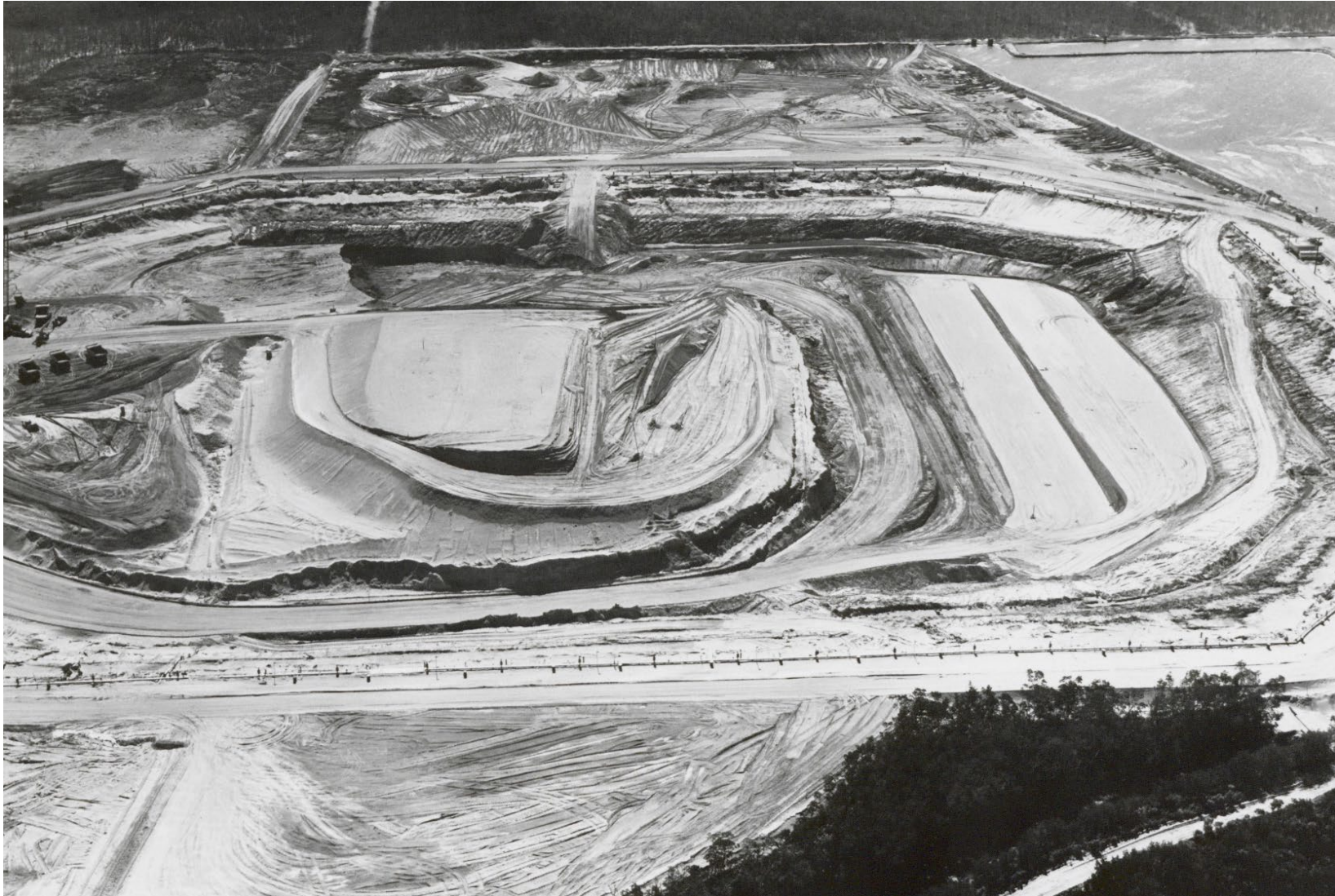
Figure 3.8-6 Construction Photograph of the PSL Site Showing Tree Removal, Excavation, and Mechanical Leveling
