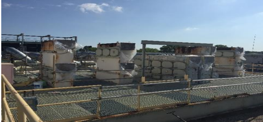
Roof Equipment - Before
