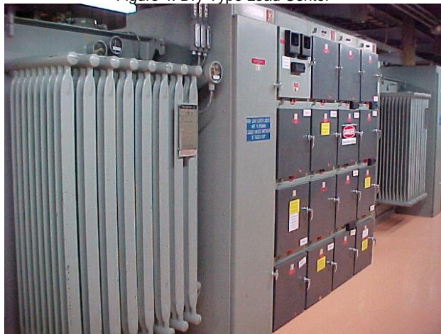
Figure 5: Liquid-Cooled Load Center
