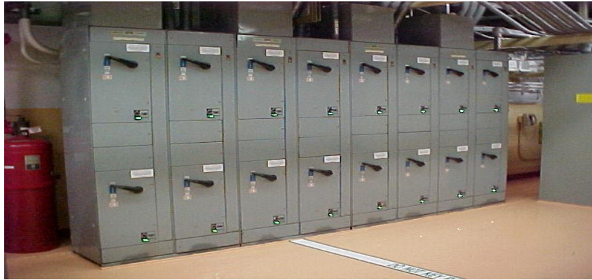
Figure 6: Example of Motor Control Center (MCC)
