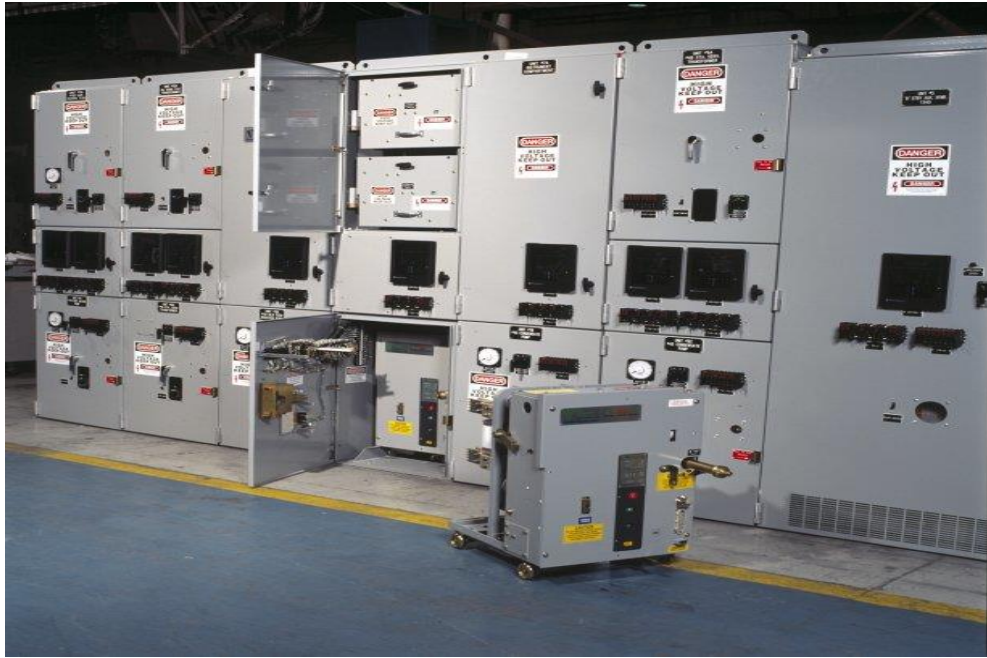
Figure 2: Medium Voltage Switchgear
