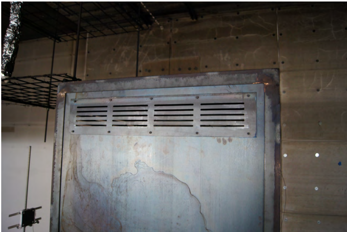
Fig. 20. Photograph of the grill over the large cabinet upper vent. Note that the grill covers approximately three-fourths of the opening area.
