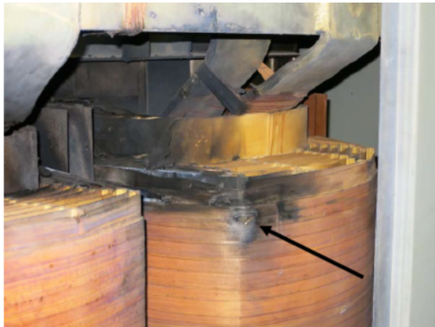
Figure 5-22 Damaged dry transformer
