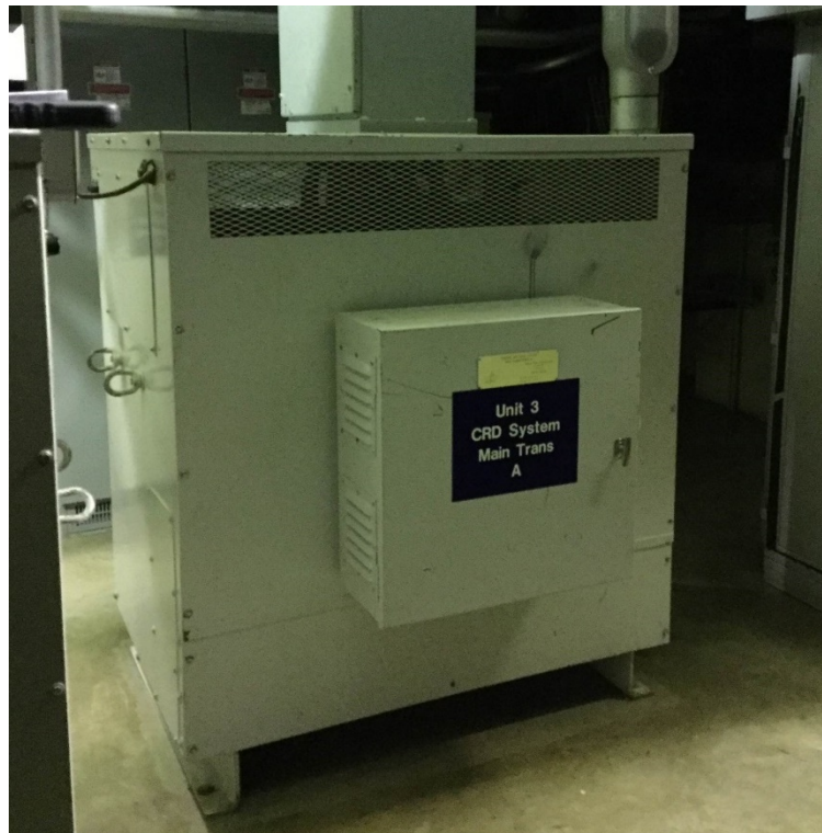
Figure 5-15 Example of typical dry transformer, midrange (375 kVA)
