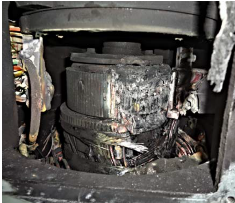
Figure 5-12 40 hp motor fire event-internal impacts
