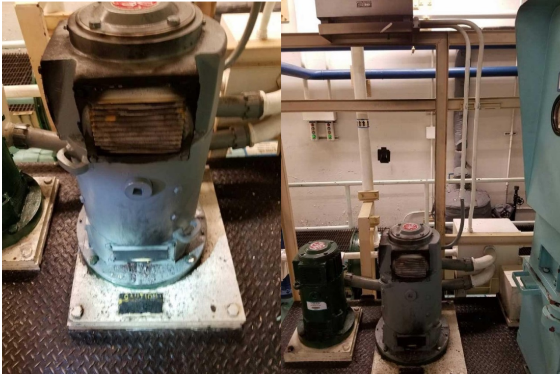
Figure 5-11 40 hp motor fire event-external impacts
