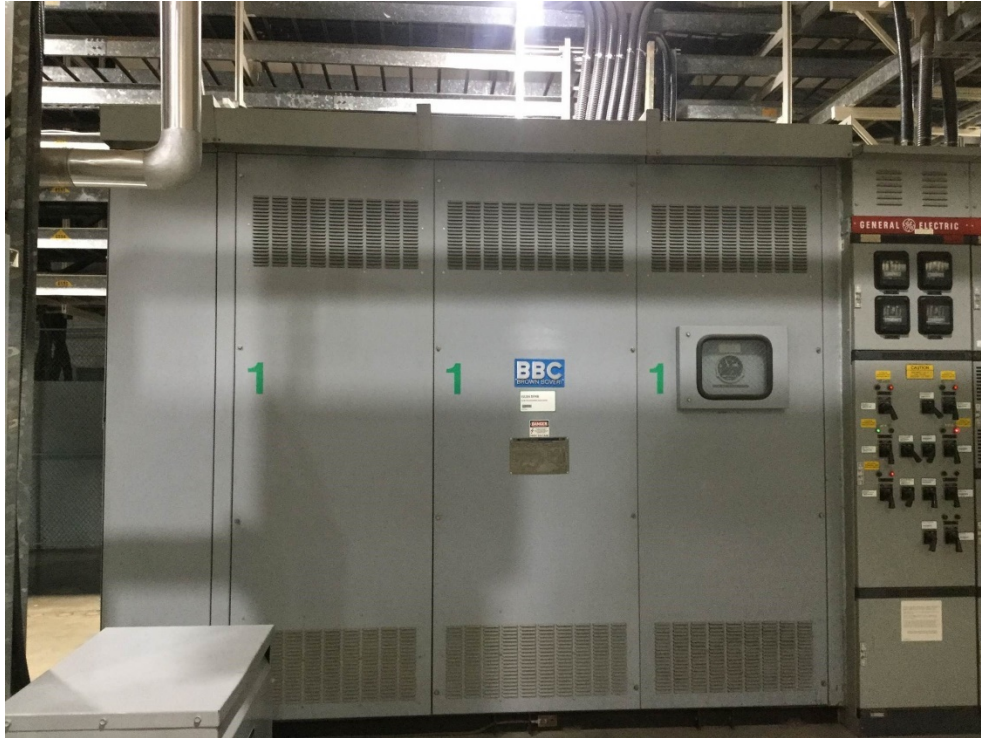
Figure 5-16 Example of typical large dry transformers (2000 kVA)
