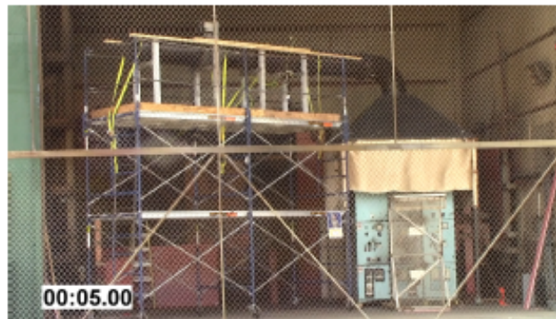
Test #3: 480 V, 35 kA, 8 seconds Copper Bus Bars
