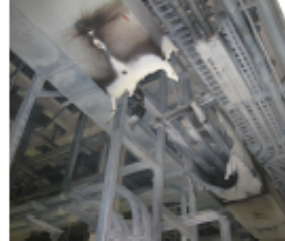
Columbia Bus Duct (OpE) 2009
