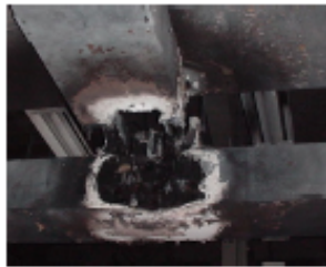
Diablo Canyon Bus Duct (OpE) 2000
