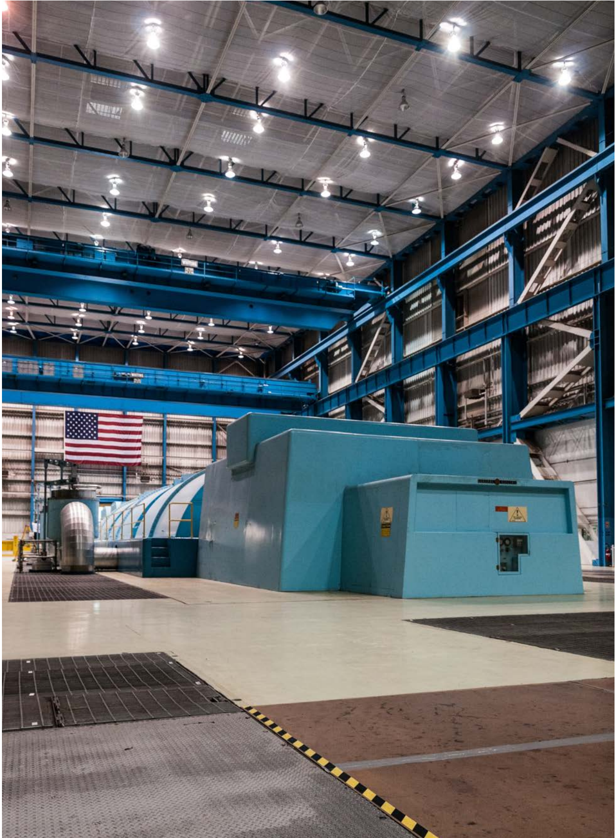
Nuclear power plant generator.
