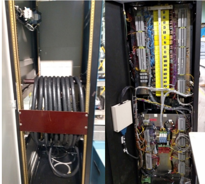
Figure 3-5: CT Testing Configuration and Data Logger
