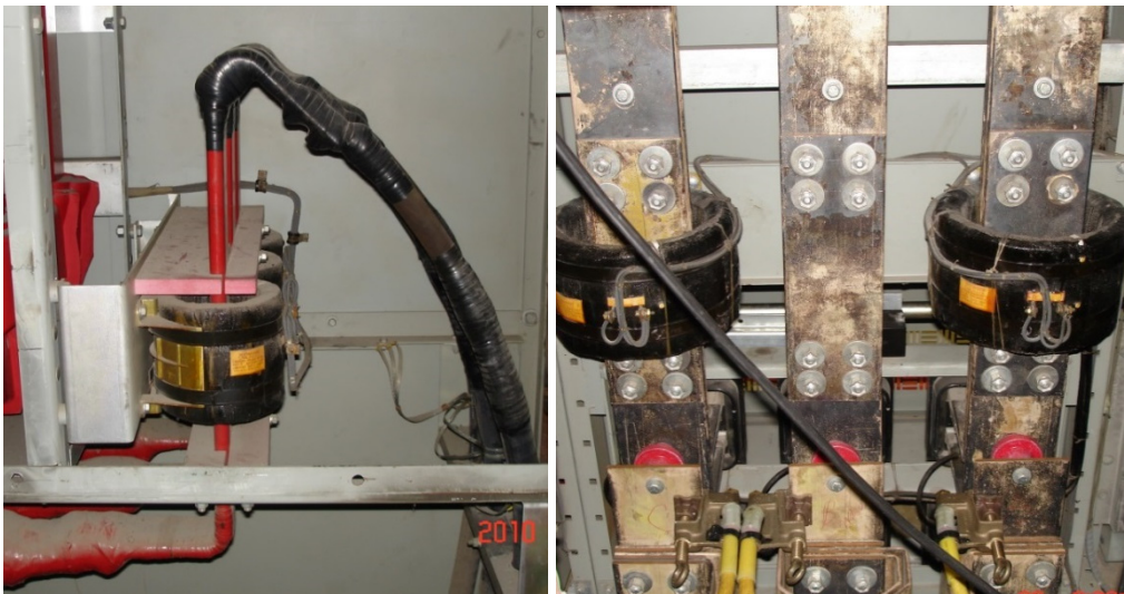
Figure 2-1: Application of Window-Type CTs in Nuclear Power Plants
