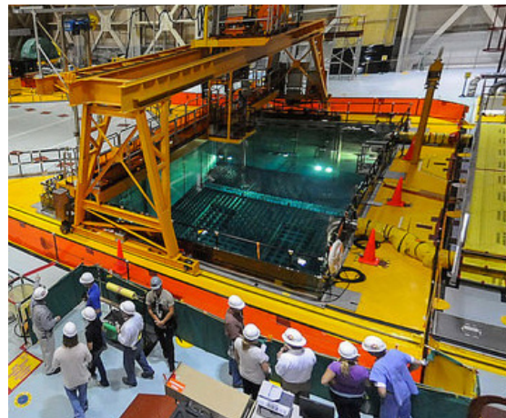
At least 23 feet of water covers the fuel assemblies in the spent fuel pool of Unit 2 at the Brunswick Nuclear Power Plant in Southport, NC. (Courtesy: Matt Born/Wilmington Star-News)
