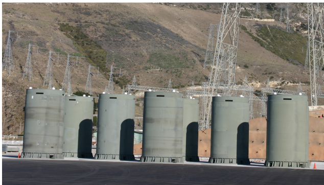
Loaded vertical HI-STORM 100 casks are storing spent fuel at the Diablo Canyon Power Plant in Avila Beach, CA.
