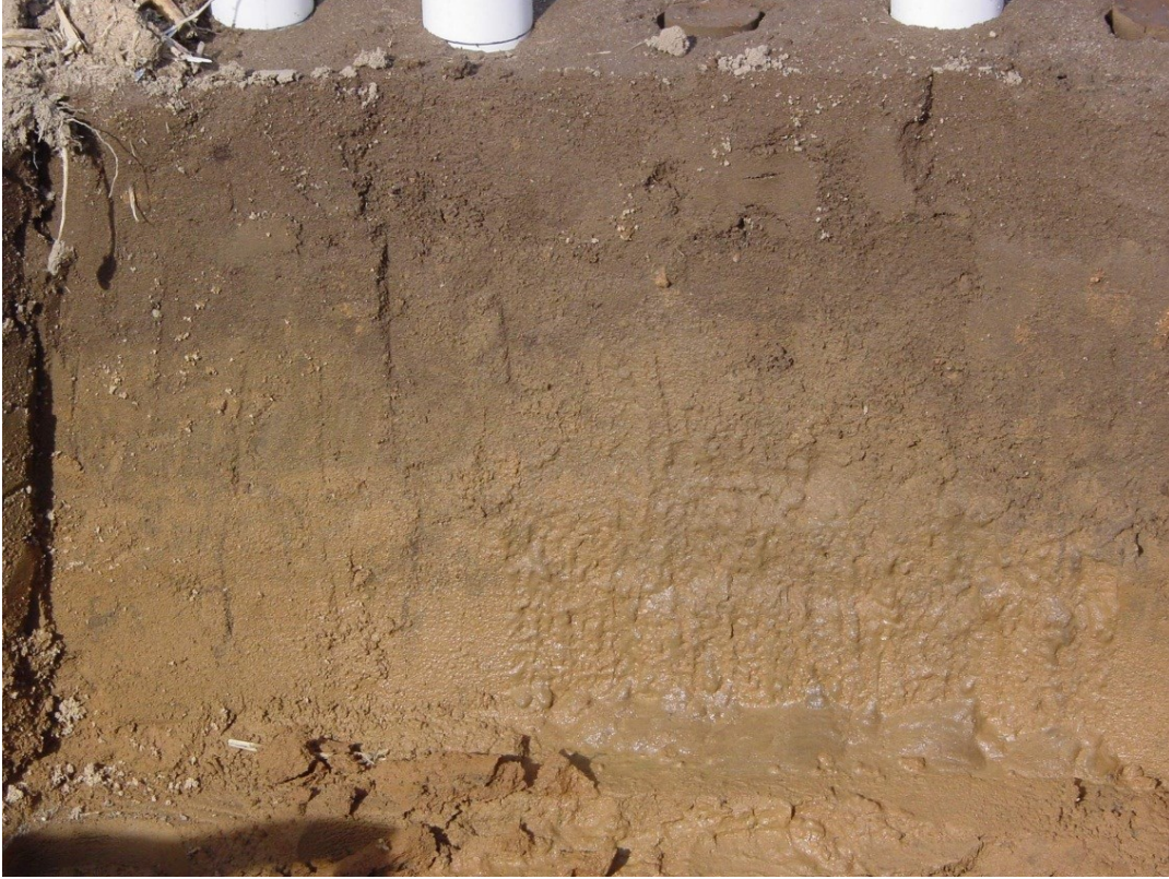
Figure 3-7 Water seepage from the wall above a locally restrictive soil layer near well w50.
