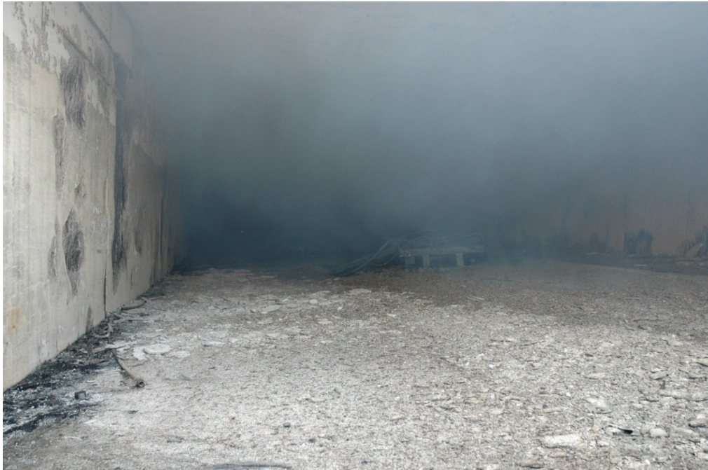
Figure 2.6. Newhall Pass Tunnel Entrance at 10/13/2007 7:58 a.m. (photo from MAIT Report, CHP 2007, reprinted with permission.)
