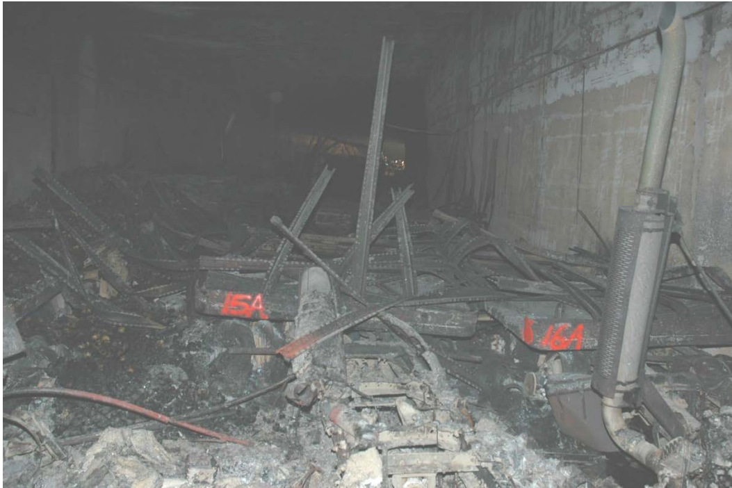
Figure 2.7. Vehicles Near Middle of Tunnel, View Toward Tunnel Entrance (photo from MAIT Report, CHP 2007, reprinted with permission.)
