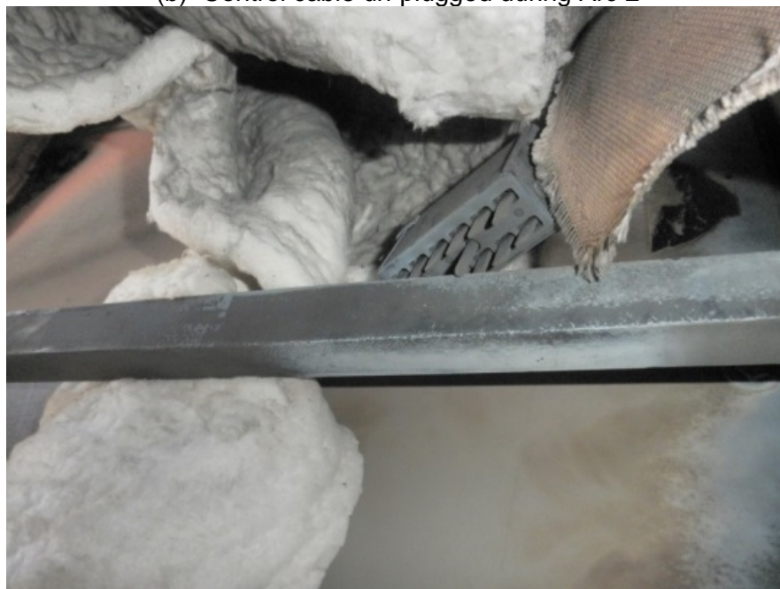
Figure 5.7-5. SWGR Test 6 Breaker Opened in Arc 2
