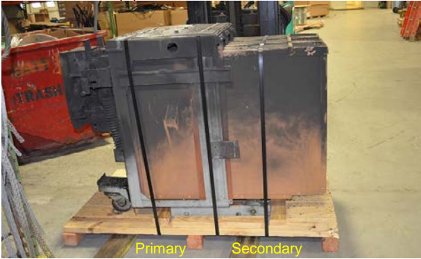
Figure 4.7-7. SWGR Test 1 Breaker Damage
