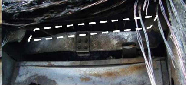
(b) Cabinet 7 Horizontal Bus Bars
