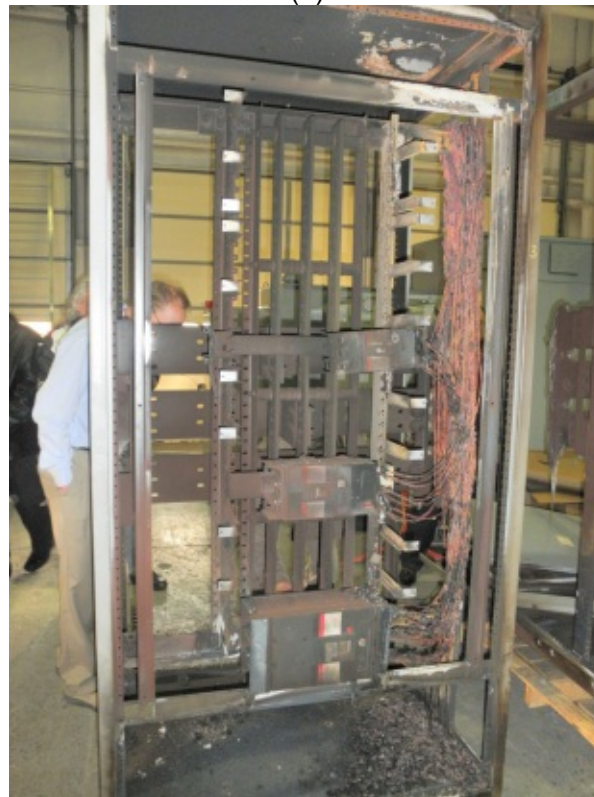
Figure 2.10-5. DP Test 3 Interior Damage
