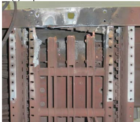
Figure 2.12-6. DP Test 5 Bus Bar Damage at Arc Location
