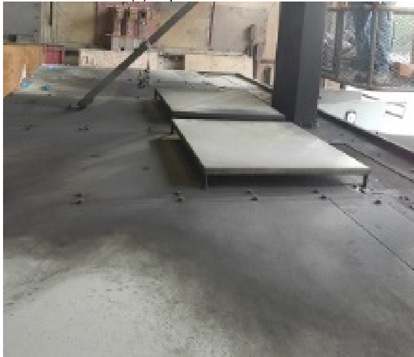
Figure 4.7-3. SWGR Test 1 Exterior Damage, continued
