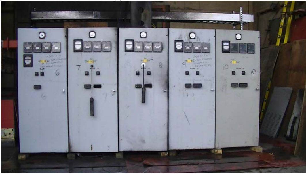
(b) Top of Cabinets (from Cabinet 8 side)
