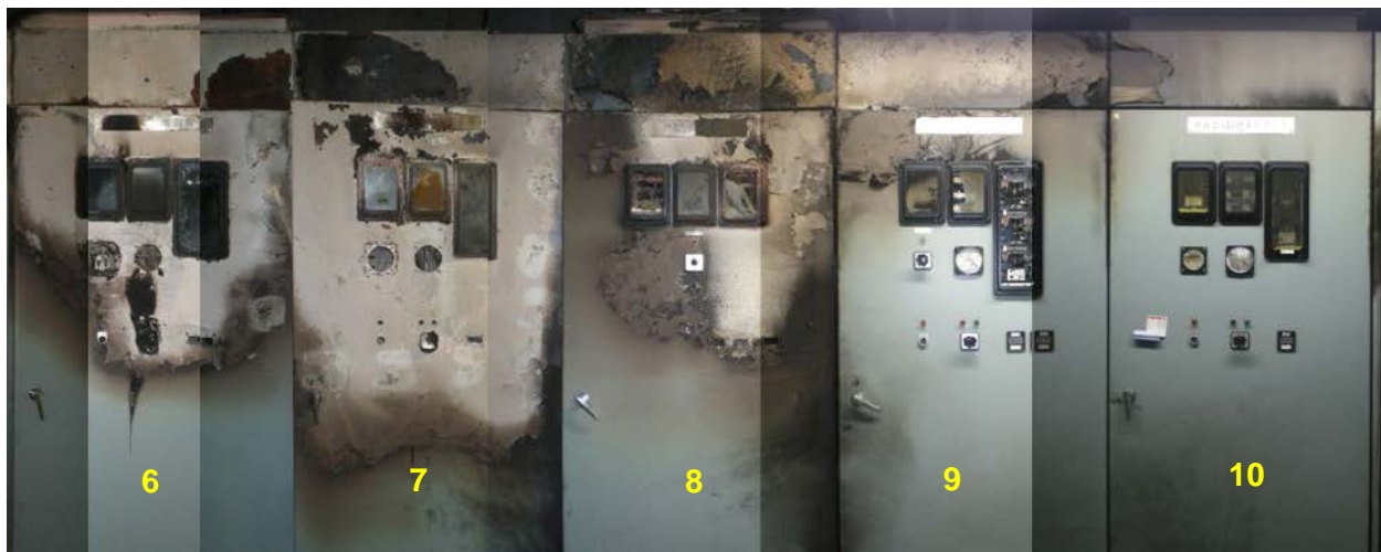
Figure 1.2-1. Damage in Onagawa HEAF Event
