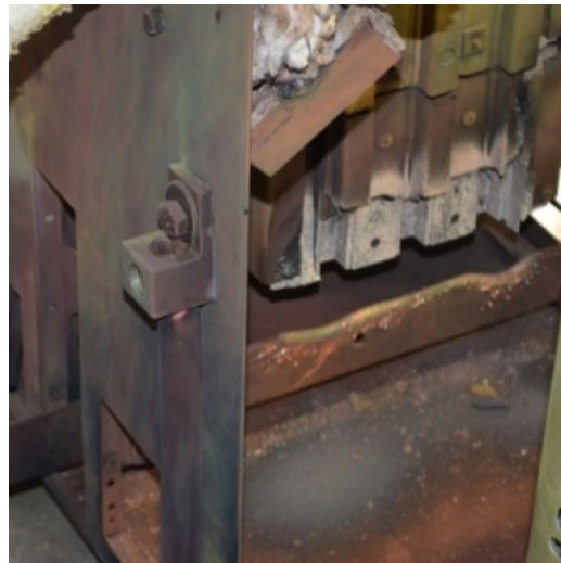
(c) lower bus bar damage
