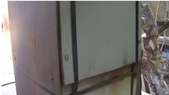
Figure 3.9-3. MCC Test 3 Exterior Damage.
