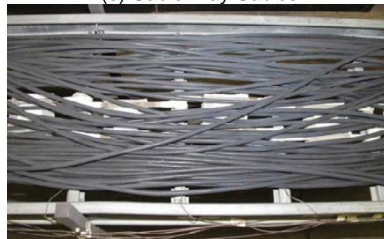
Figure 5.7-6. SWGR Test 6 Cabinet Exterior Damage
