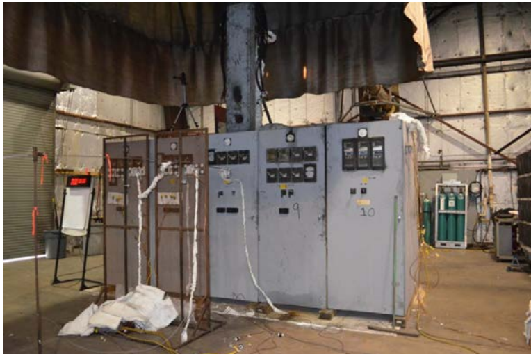
Figure 6.3-1. SwRI 5-Cabinet RFAS Test Setup
