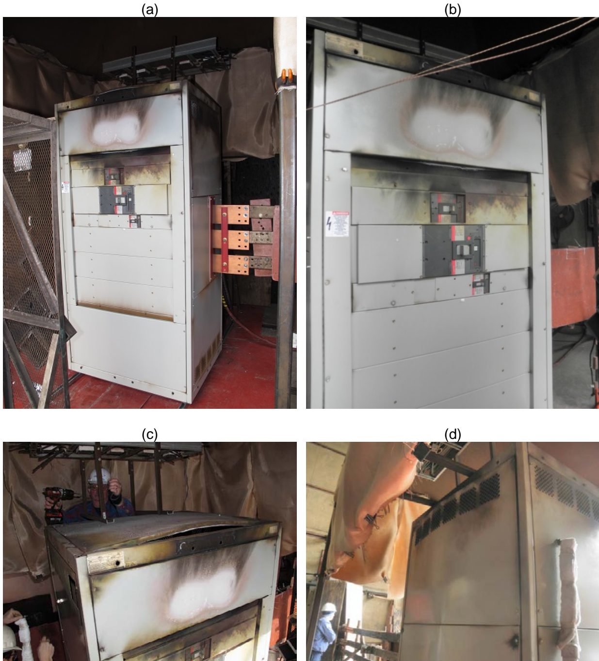
Figure 2.11-4. DP Test 4 Exterior Cabinet Damage
