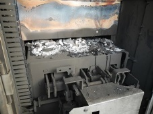
(a) Cabinet 8 breaker with insulator debris
