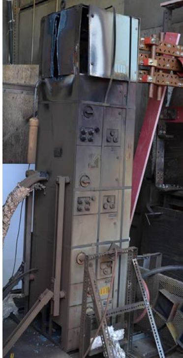
(a) Exterior damage
