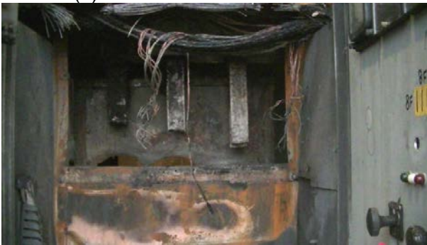
(a) Cabinet 7 Vertical Bus Bars
