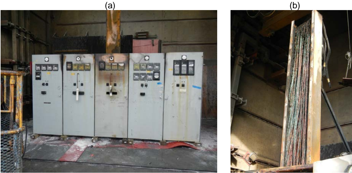
Figure 4.9-1. SWGR Test 2 Exterior Damage
