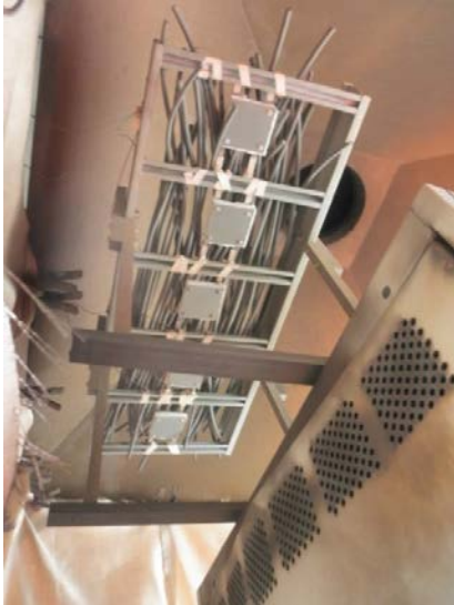
Figure 2.11-5. DP Test 4 External Cable Tray Damage
