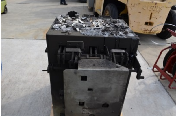
(b) Cabinet 8 breaker with insulator debris
