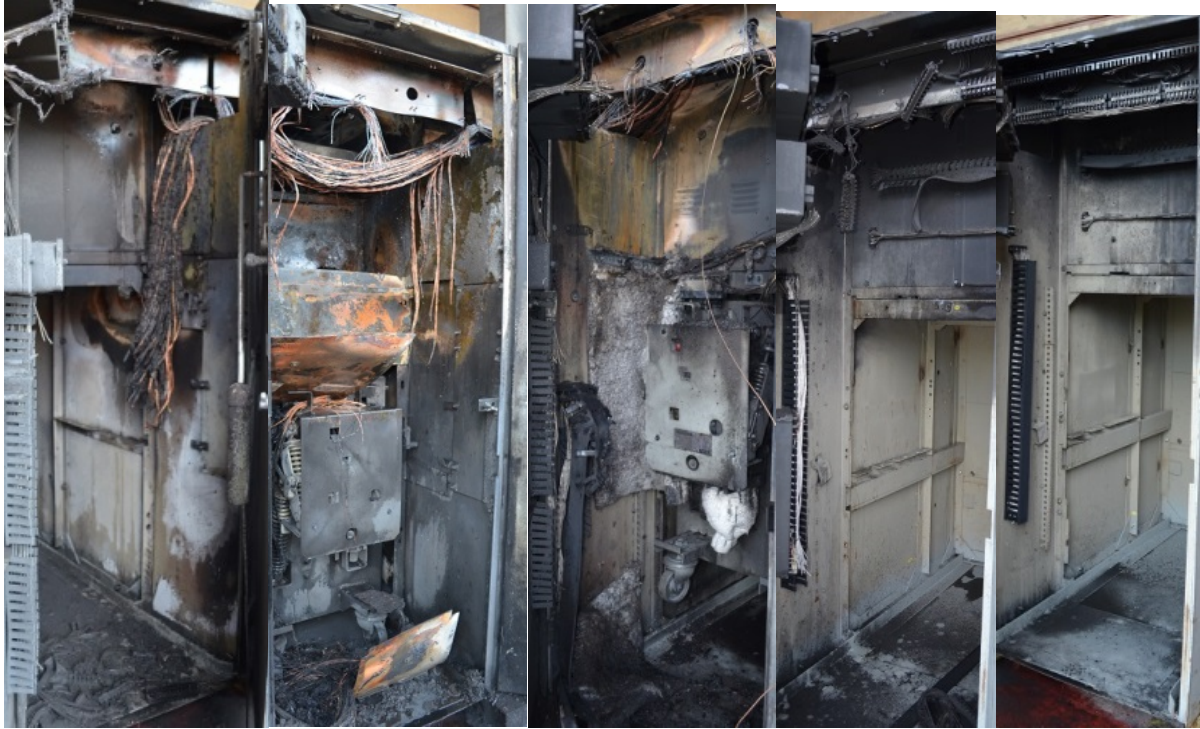
Figure 5.5-4. SWGR Test 4 Interior Damage
