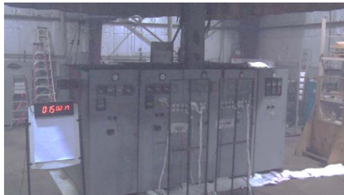
Figure 6.9-4. Test 1 Exterior Cabinet Damage
