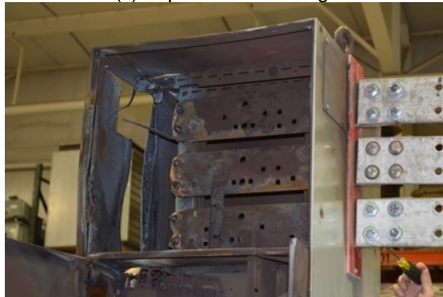
Figure 3.8-4. MCC Test 2 Exterior Damage
