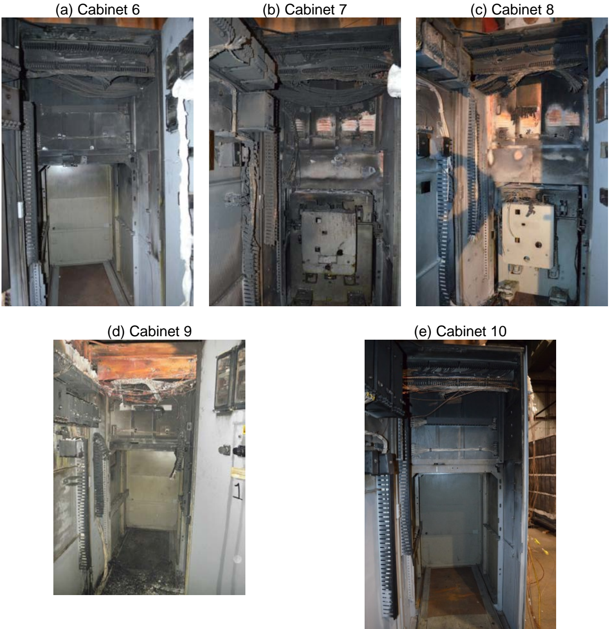
Figure 6.10-3. Test 2 Interior Cabinet Damage
