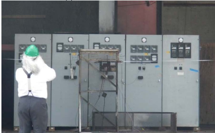
Figure 4.7-3. SWGR Test 1 Exterior Damage
