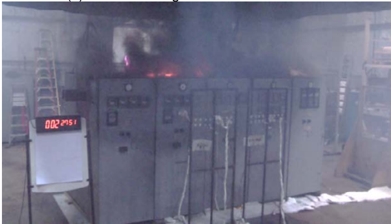
(b) 5 minutes after RFAS1. Note the low maximum temperature- there is residual heat, but no fire
