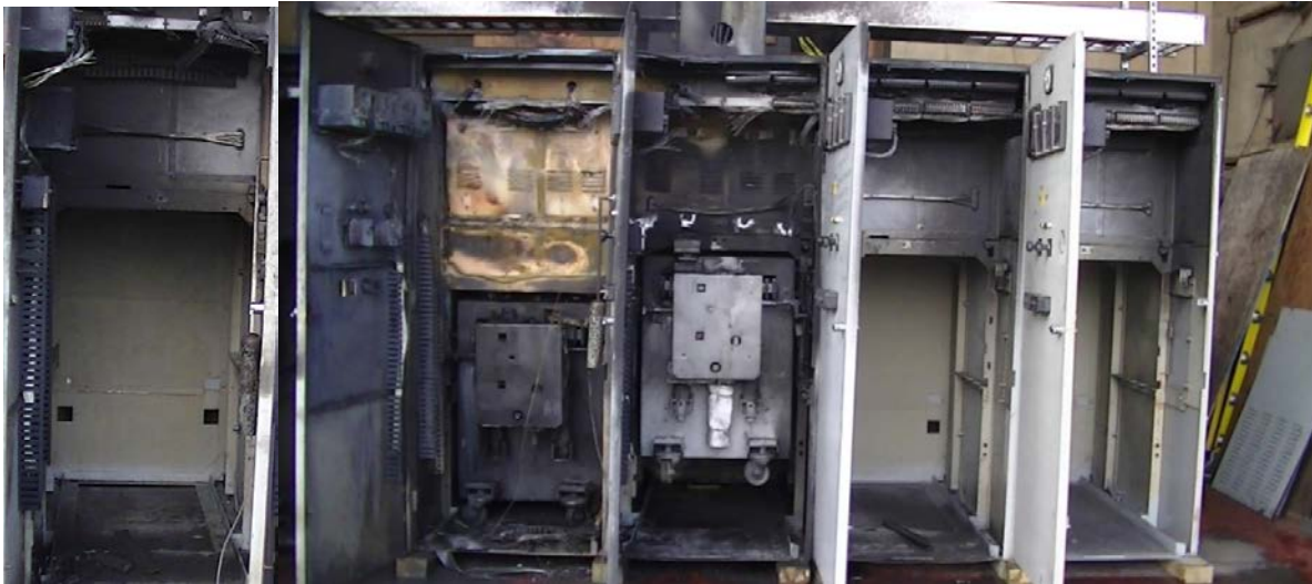
Figure 5.6-4. SWGR Test 5 Interior Damage
