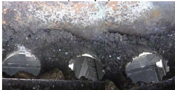
(b) Cabinet 7 Insulators 1, 2 and 3 (destroyed)
