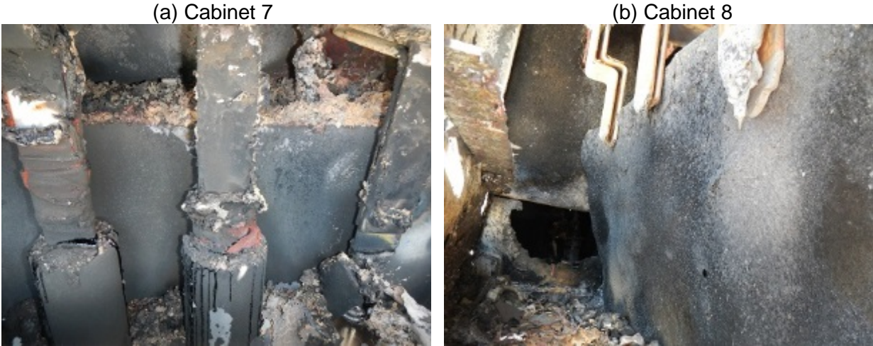
Figure 4.10-6. SWGR Test 3 Insulator and Bus Bar Damage
