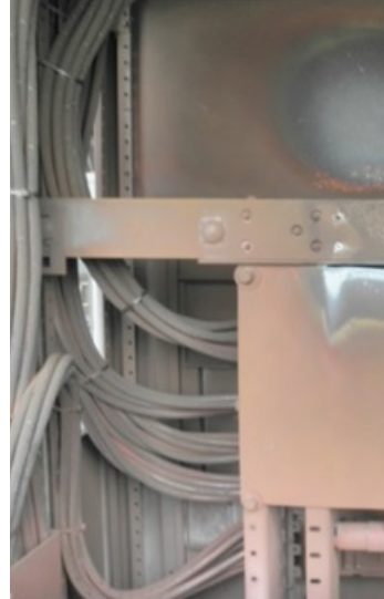
Figure 2.11-6. DP Test 4 Interior Cable Damage
