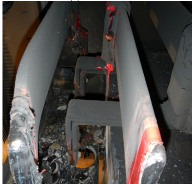
Figure 4.7-6. SWGR Test 1 Insulator and Bus Bar Damage
