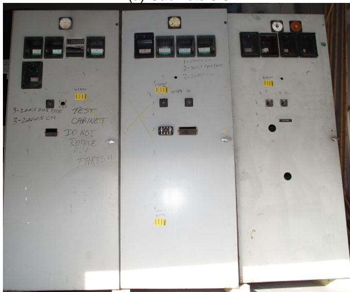
(b) Side of Cabinet 8
