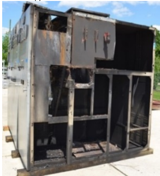
Figure 4.10-5. SWGR Test 3 Interior Damage, Detailed
