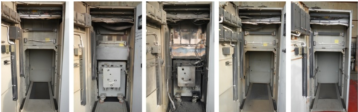
Figure 4.7-4. SWGR Test 1 Interior Damage
