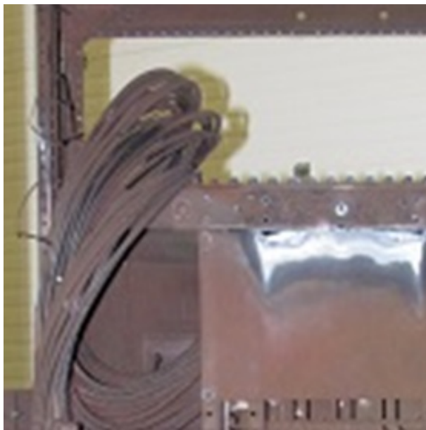
Figure 2.13-5. DP Test 6 Interior Cable Damage
