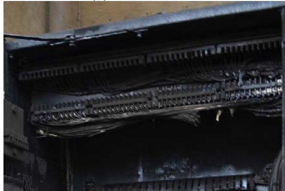
(c) Cabinet 7 Cables
