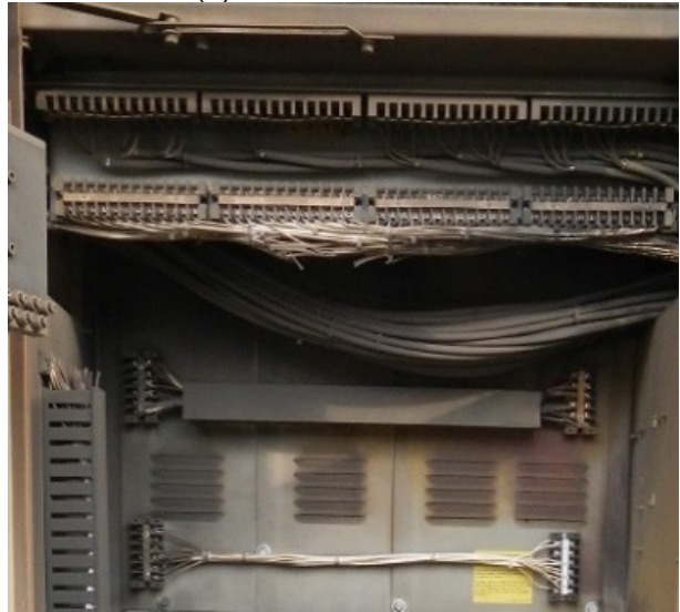
(b) Cabinet 7 Cables
