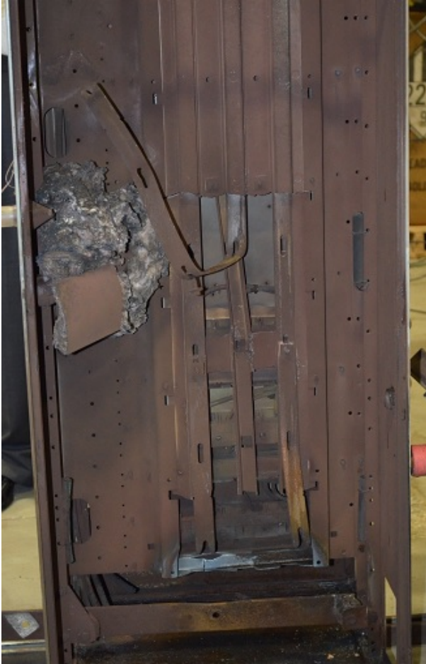
(a) Bottom Arc Damage
