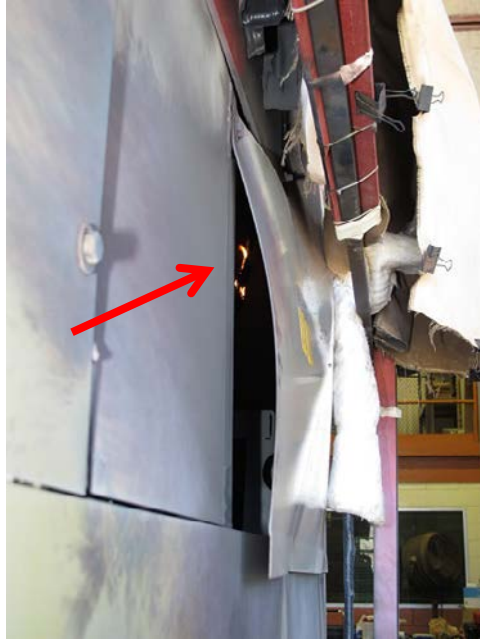
Figure 5.7-9. SWGR Test 6 Cabinet 8 Breaker Control Interior Wire Fire
