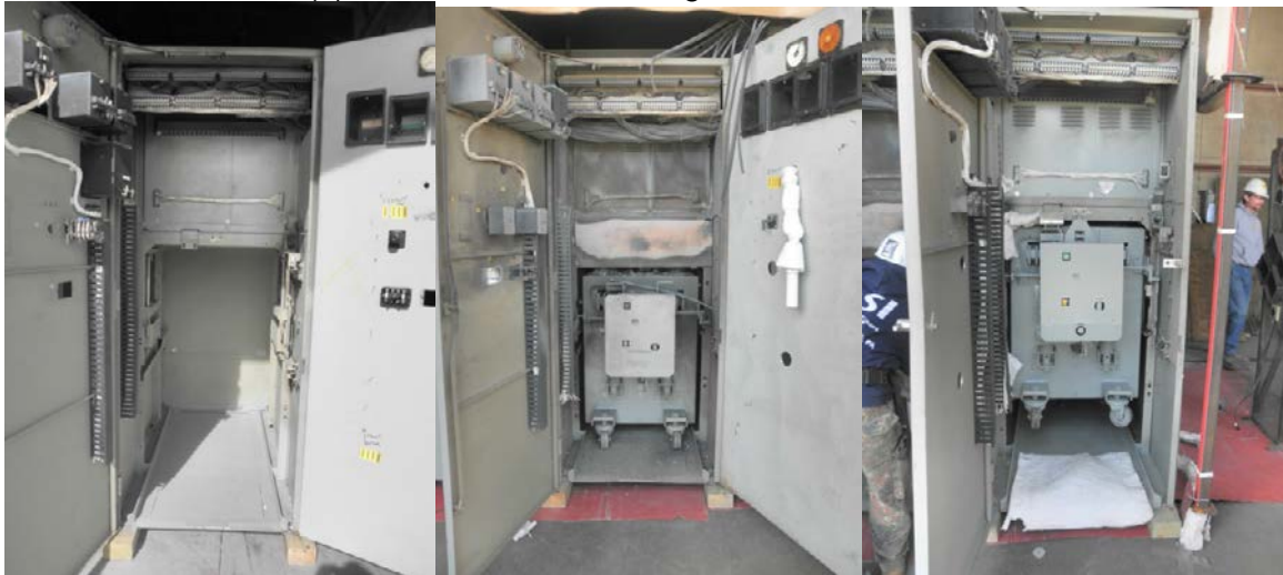
Figure 5.7-7. SWGR Test 6 Cabinet Interior Damage
