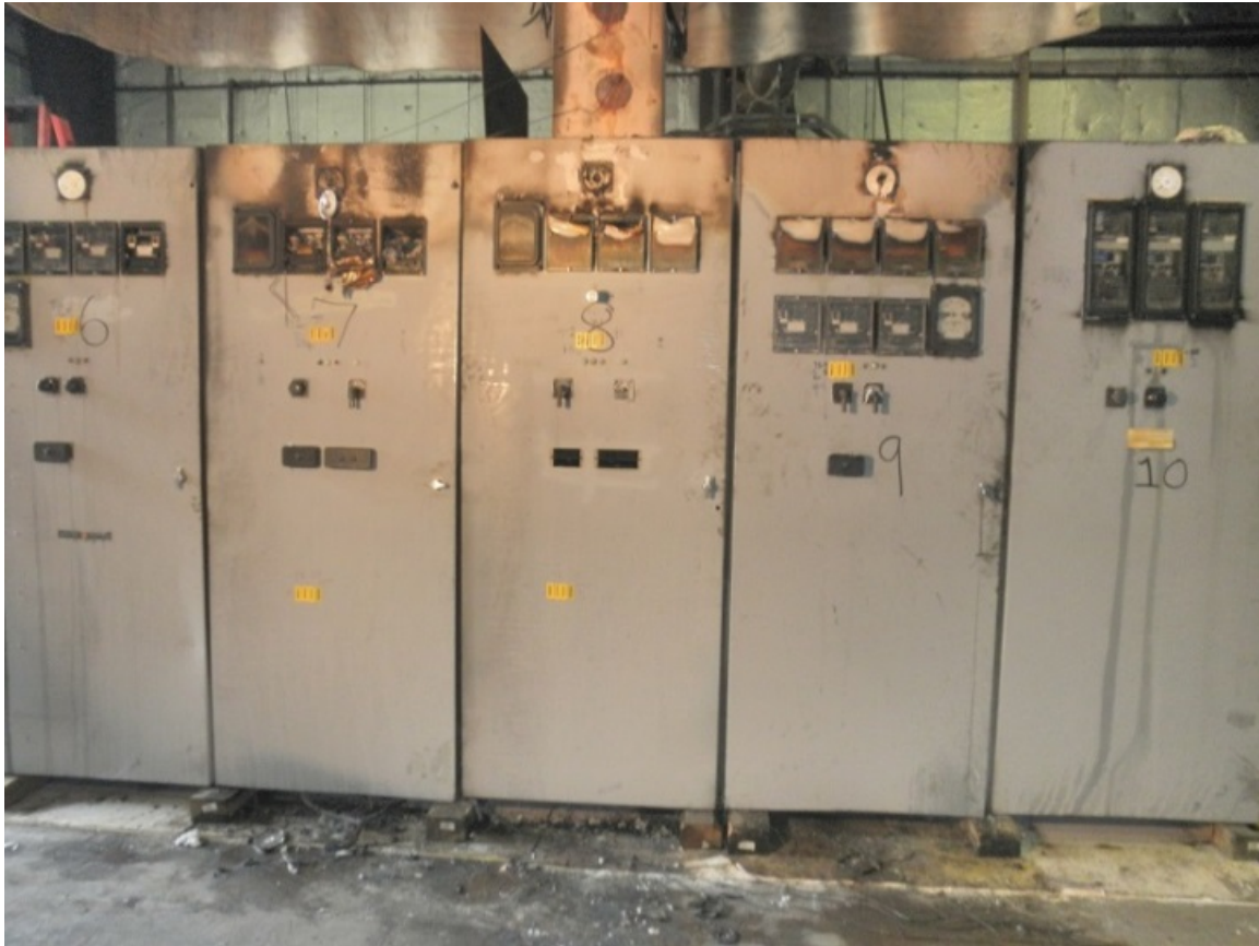
Figure 6.10-4. Test 2 Exterior Cabinets Damage
