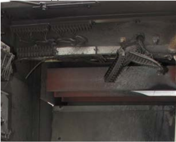
(a) Cabinet 6 Cables
