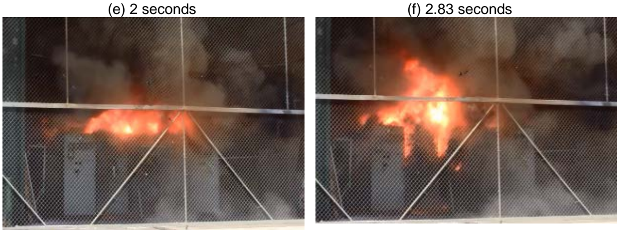
Figure 4.10-1. SWGR Test 3 Arc, continued
