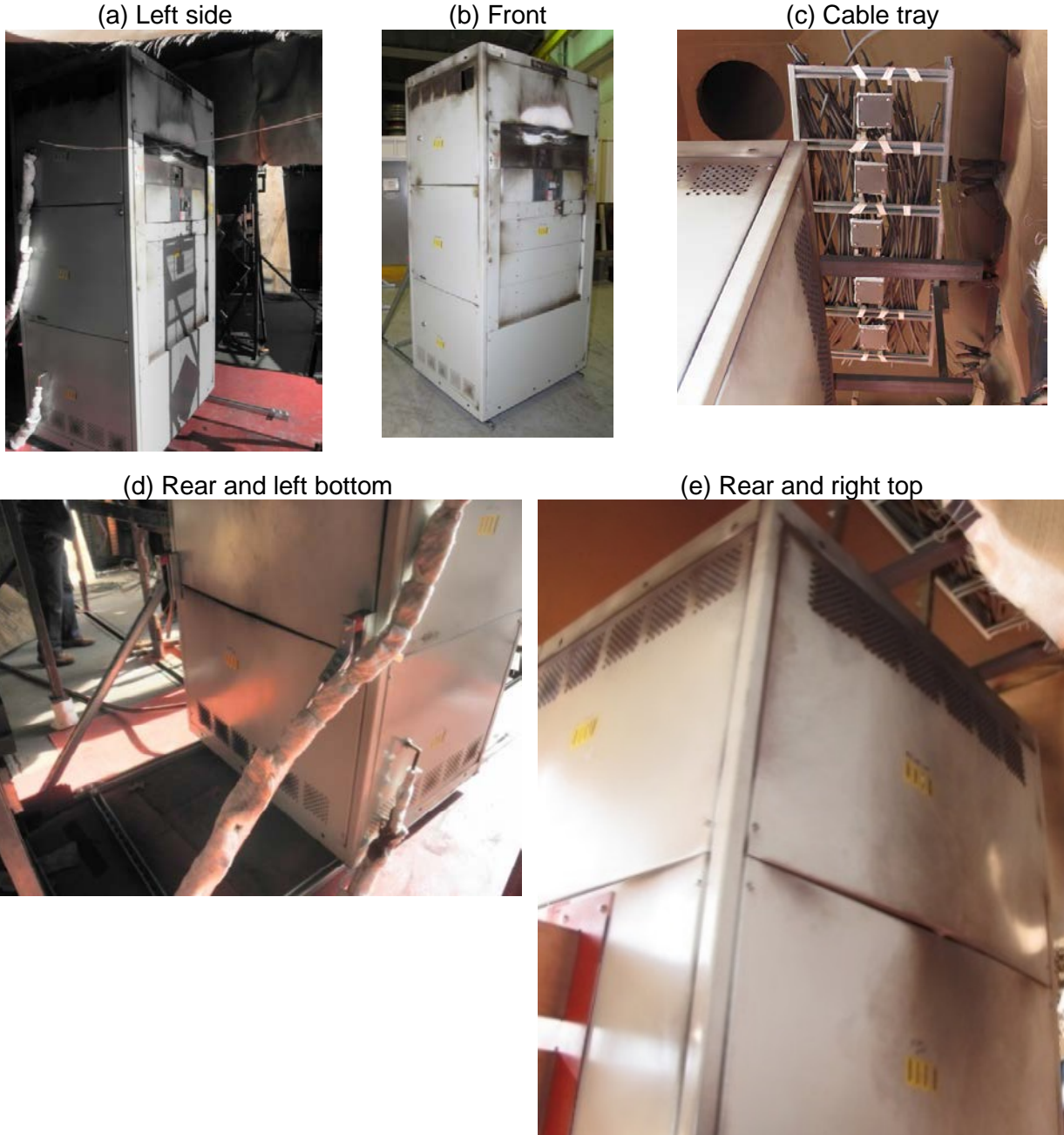
Figure 2.13-4. DP Test 6 Exterior Damage
