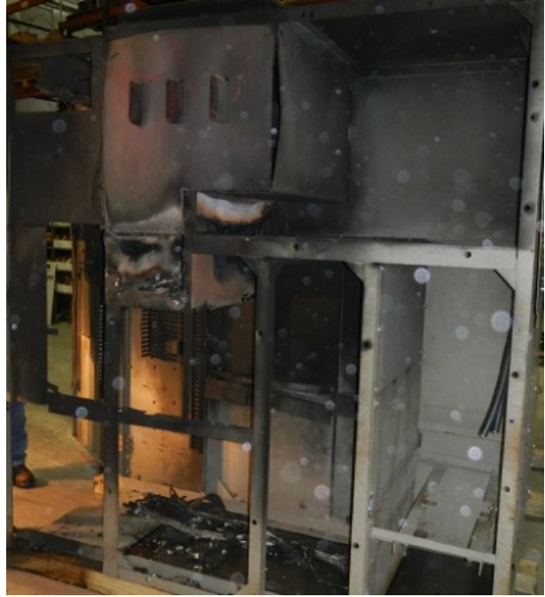
Figure 4.7-5. SWGR Test 1 Interior Damage, Detailed, continued
