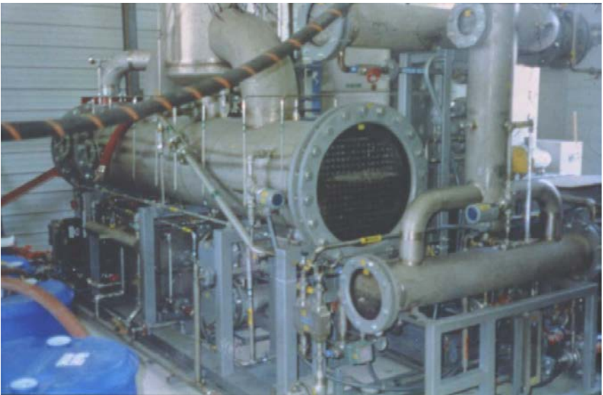
Processed water disposal system disposed of 2.3 million gallons of processed accident-generated water by evaporation and disposal of solid residue.
