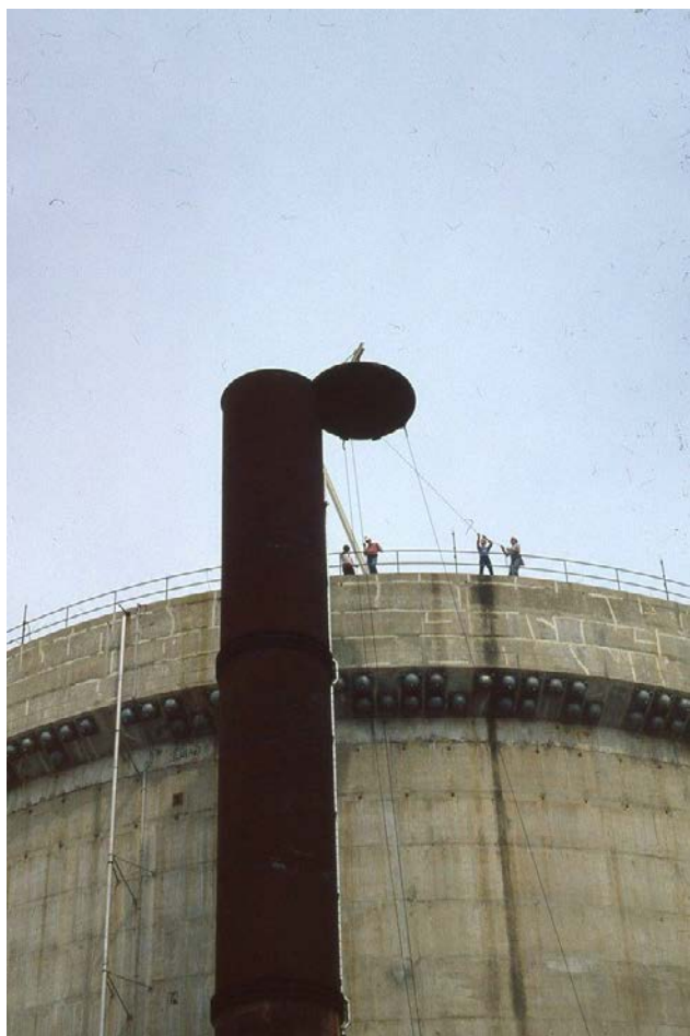
The TMI-2 ventilation stack being uncapped for the planned purge of accident-generated radioactive krypton gas from the reactor building. The ventilation stack was previously capped to redirect ventilation from the auxiliary and fuel handling building to the temporary supplementary air filtration system.
