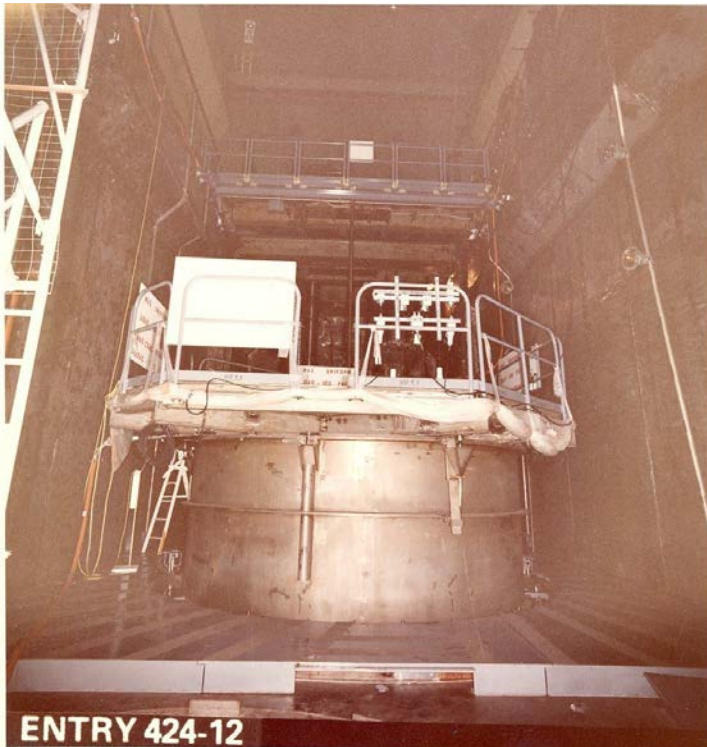
Internals indexing fixture with its temporary cover mounted on the reactor vessel flange. This fixture would eventually be mated to the defueling work platform.
