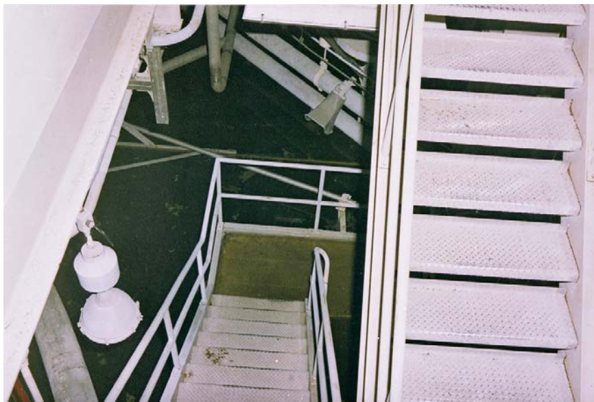
Water level in the basement reached the first stairwell landing indicating about 8 feet of water accumulation.
