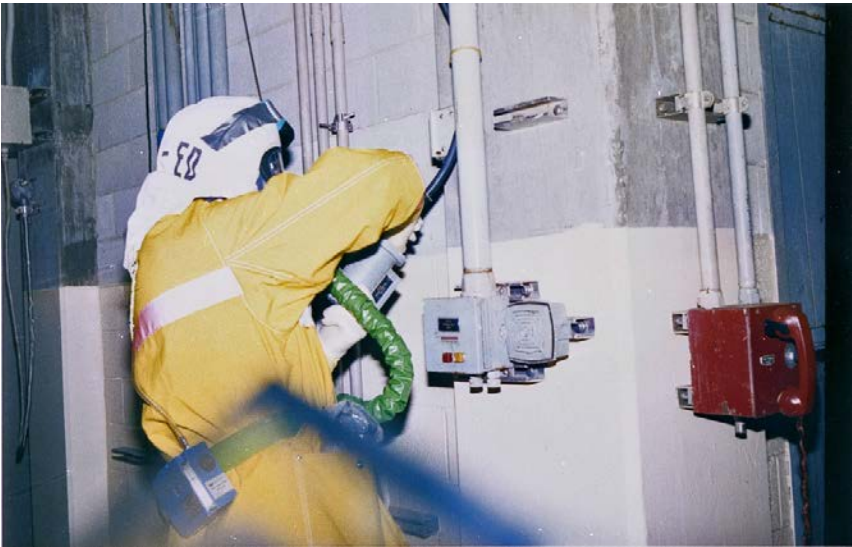
Several electrical components from the reactor building were retrieved and examined as part of the DOE-sponsored Instrumentation and Electrical Program. Shown is the removal of an area radiation monitor (HP-R-211) from the northeast elevator wall.
