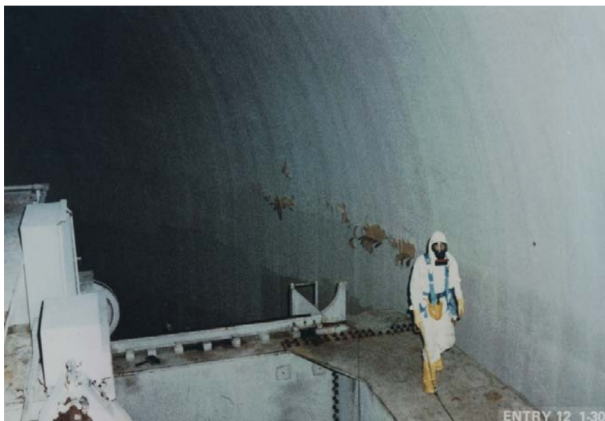
Reactor building polar crane being inspected for use in defueling preparations.
