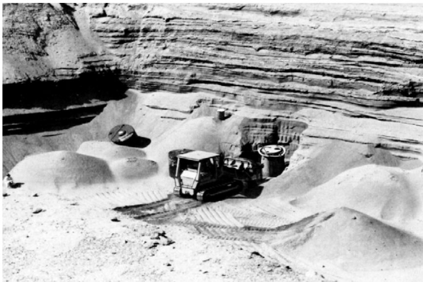
Demonstration high integrity container (HIC) being covered in the trench at the commercial radioactive waste disposal site near Richland, Washington. The HIC contained the highly loaded EPICOR II prefilter No. 18. The demonstration set the precedent for disposing of the remaining EPICOR II prefilters that were temporarily stored at INEL.
