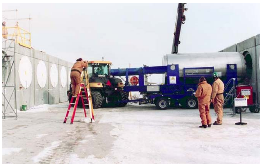
Independent spent fuel storage installation (ISFSI) for the dry storage of TMI-2 fuel debris located at the INEL. The TMI-2 defueling canisters were removed from the storage pool, dewatered, dried, and placed in a dry shielded canister. The dry shielded canister with up to 12 defueling canisters was placed inside a reinforced concrete horizontal storage module. The ISFSI was certified and licensed by the NRC.
