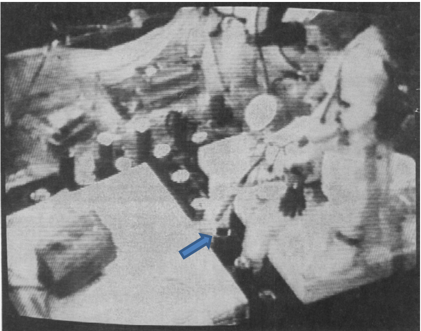
The first closed-circuit video inspection of the upper reactor core region was performed on July 21, 1982. A technician sitting on a platform positioned on top of the reactor vessel service structure is inserting a camera, 1.5 inches in diameter and 12 inches long, through an empty leadscrew support tube.
