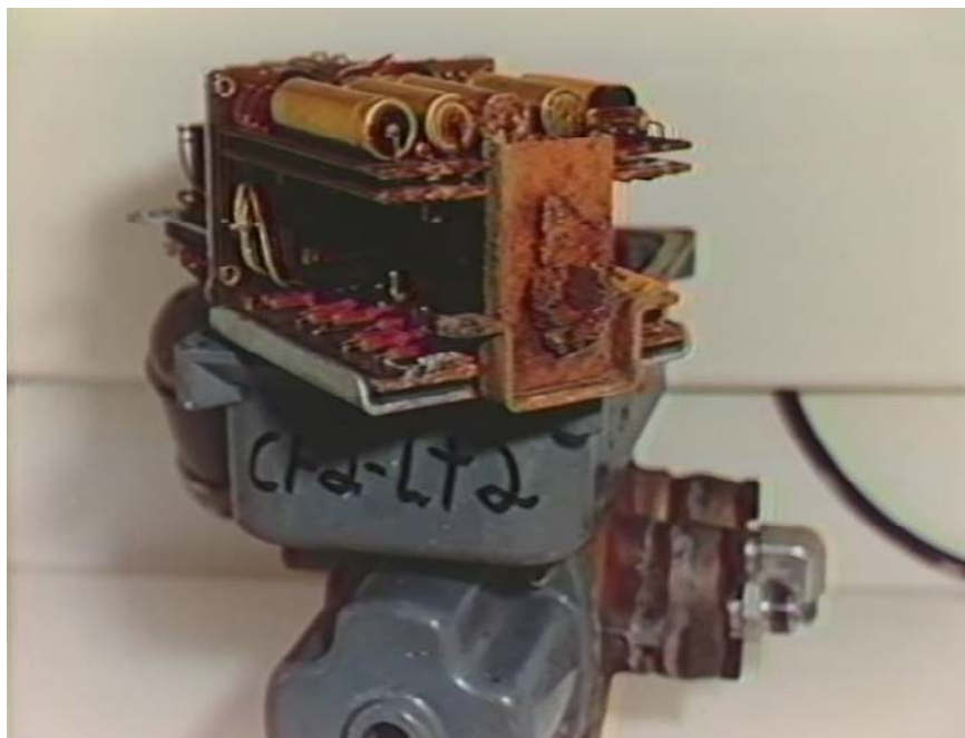
Core flood tank 1A level monitor CF-2-LT2 showing the condition of the enclosed electronic module. There was severe corrosion and degradation of internal components rendering the unit inoperable.
