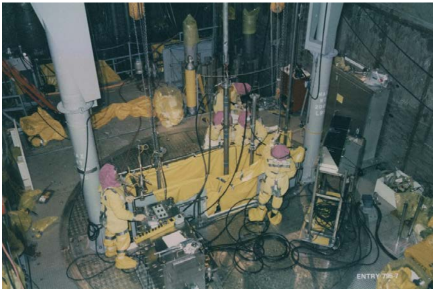
Defueling operations from the rotating defueling work platform with a worker holding a long-handled defueling tool down through the slit into the reactor vessel. Two jib cranes at each end of the slit were used to lower larger tools.
