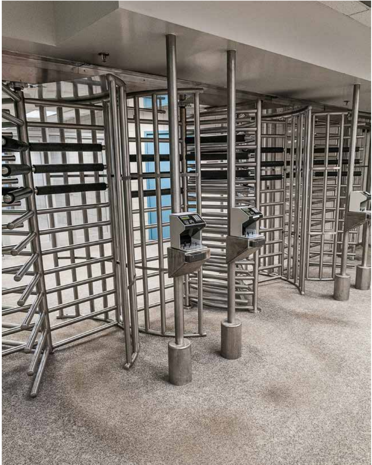
Security gates at Calvert Cliffs Power Plant.
