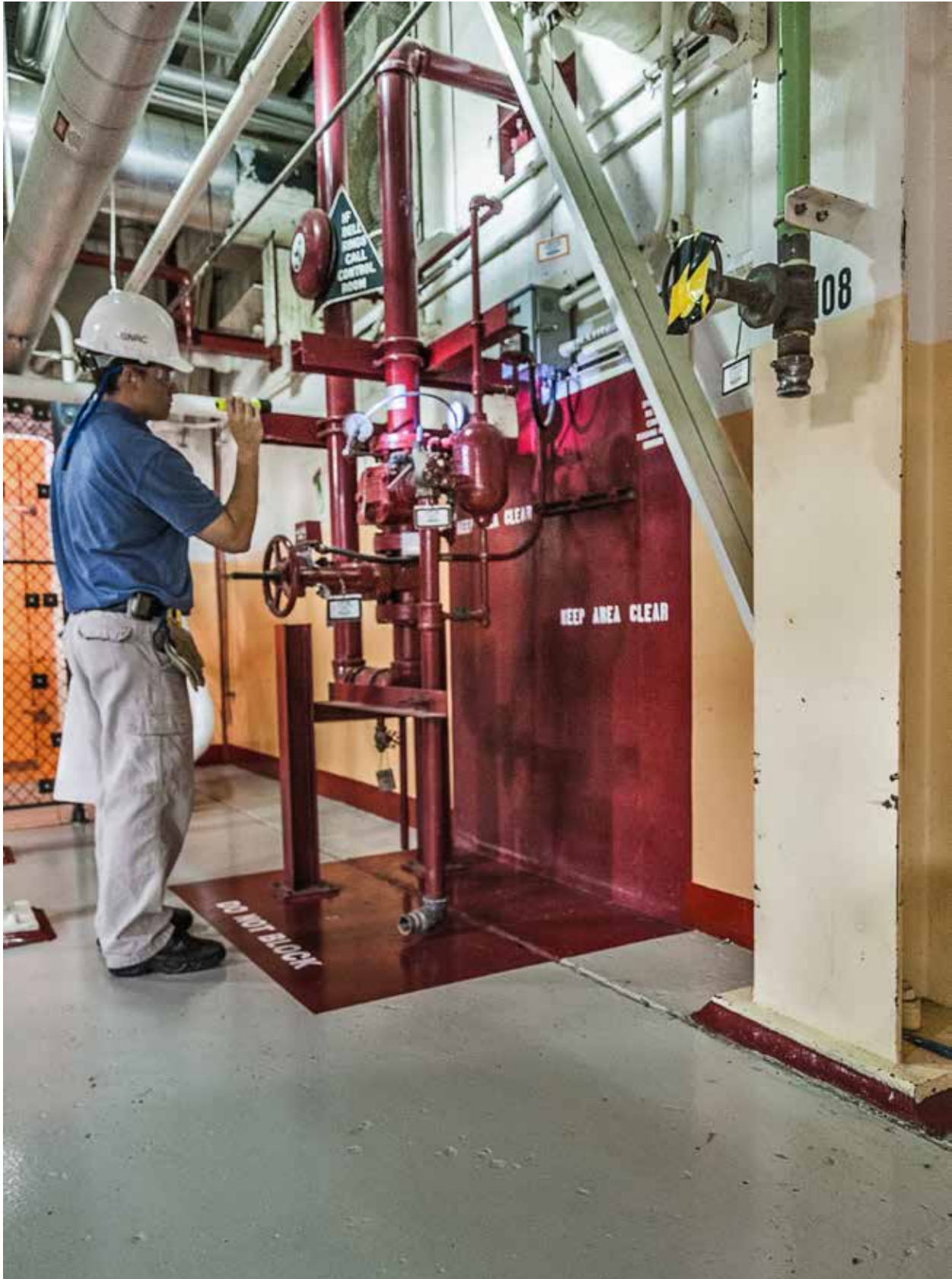
Fire equipment inspection by NRC Resident Inspector.
