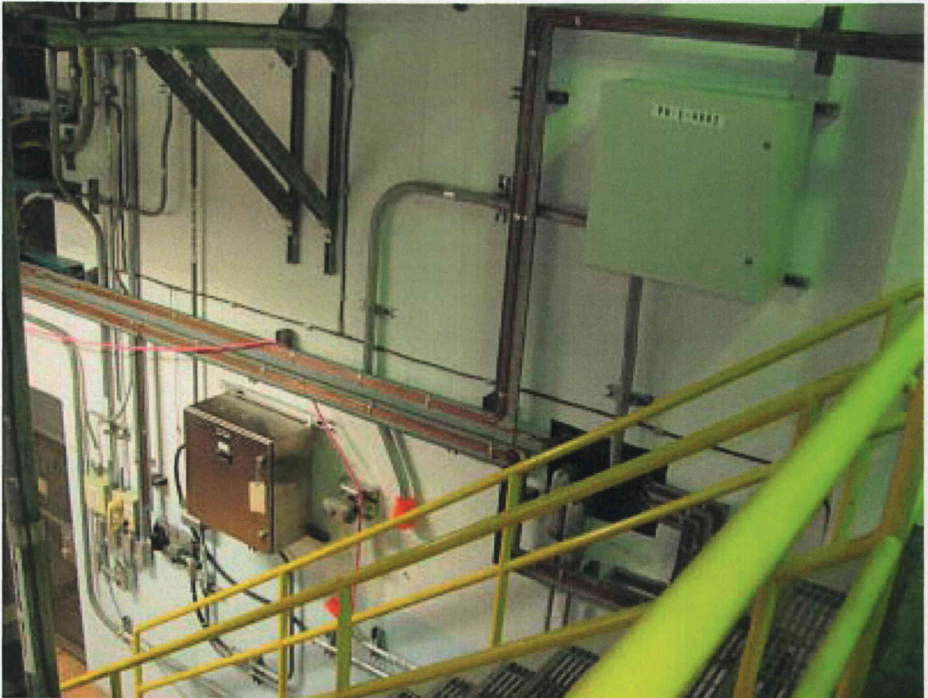
Spent Fuel Pool Level Indication Primary Level Indicator
