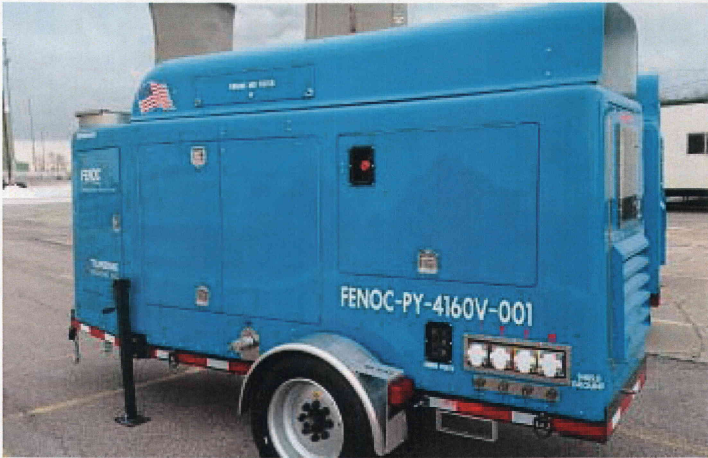
4160 Vac Generator in parking lot
