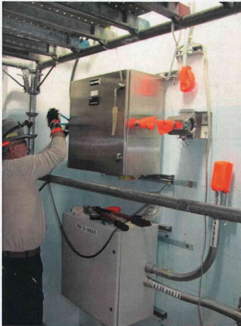
Spent Fuel Pool Level Indication Secondary Level Indicator
