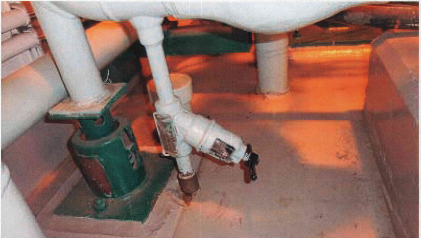
Connection for Fuel Oil to run FLEX 4160 Vac Generator
