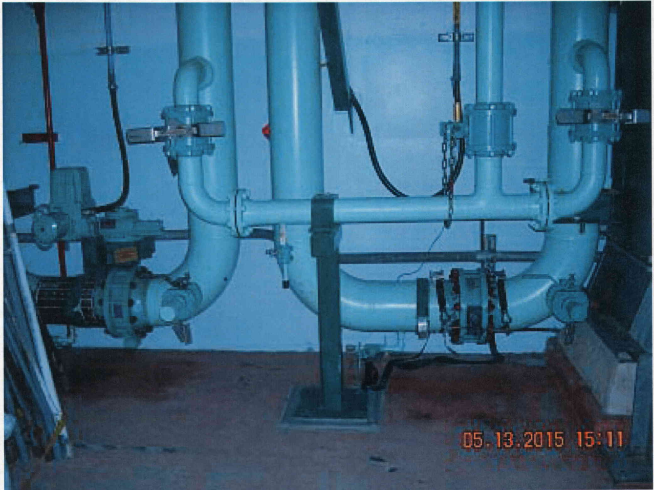
Additional view of ESW to SFP Fill Line
