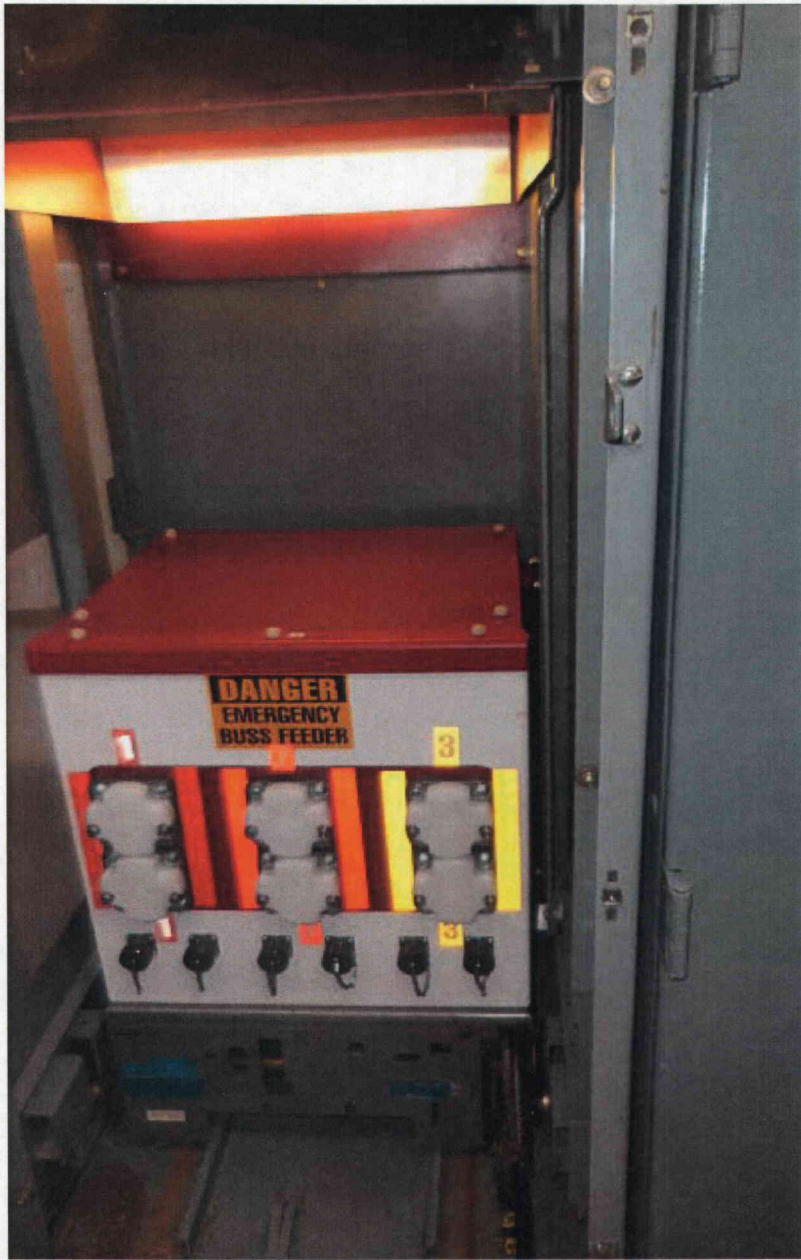
Emergency Buss Feeder during testing at Maintenance training facility
