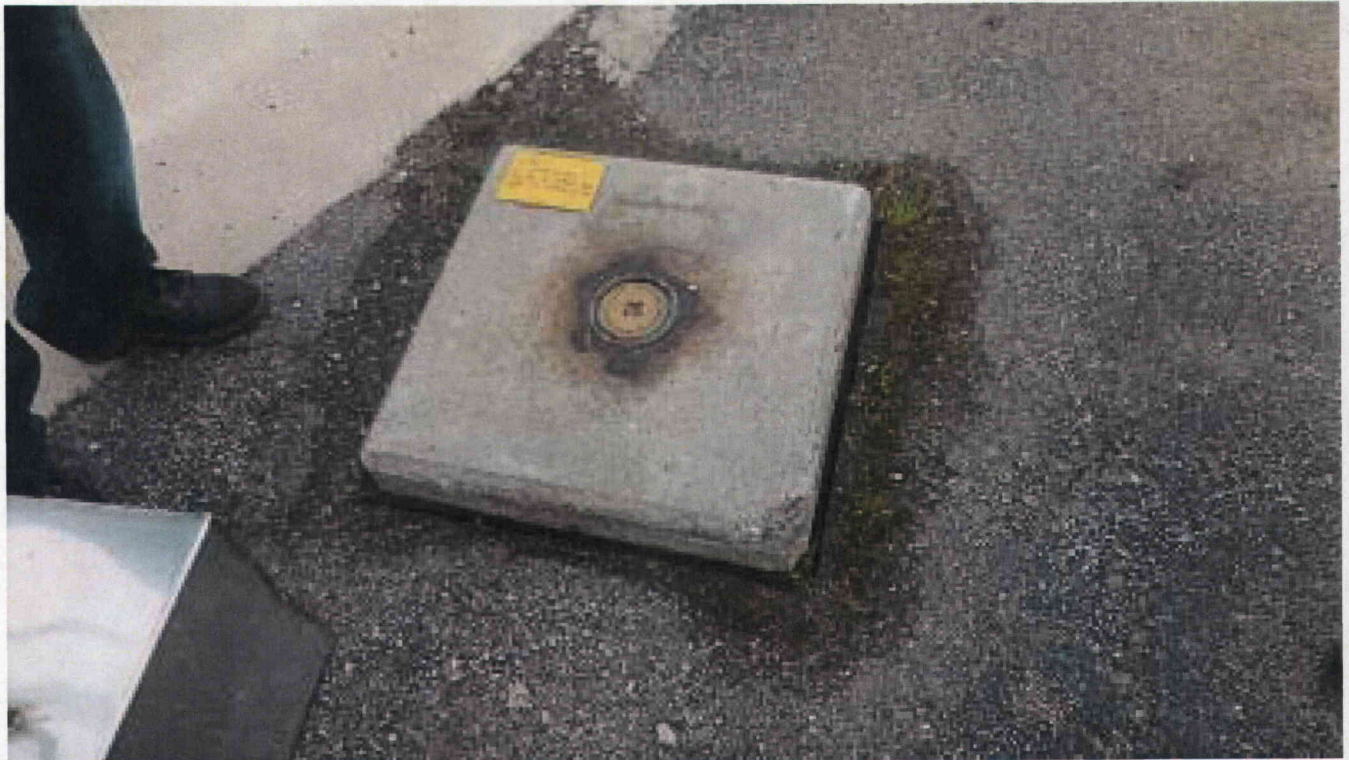
Diesel Fuel Oil Storage Tank Cover, location of fuel oil for use in FSG 70.2, SUPPLYING FUEL OIL TO ESWPH FLEX GENERATOR
