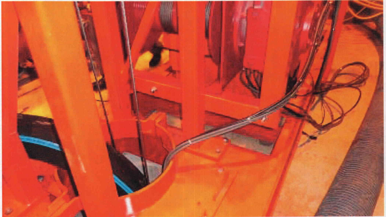
FLEX Lake Water Pump lowered into the ESW Pumphouse bay during pump testing
