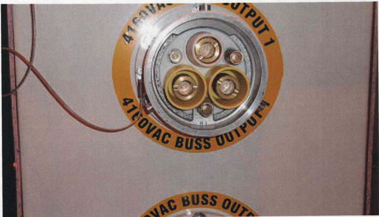
Close up of connection on Emergency Bus Feeder for use in EH 2101 and 2102
