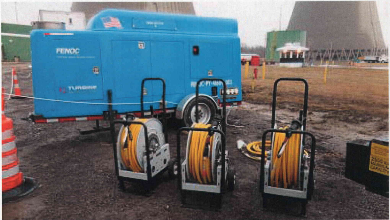
Cables and 4160 Vac Generator at ESW Pumhouse for Lake Water Pump Testing
