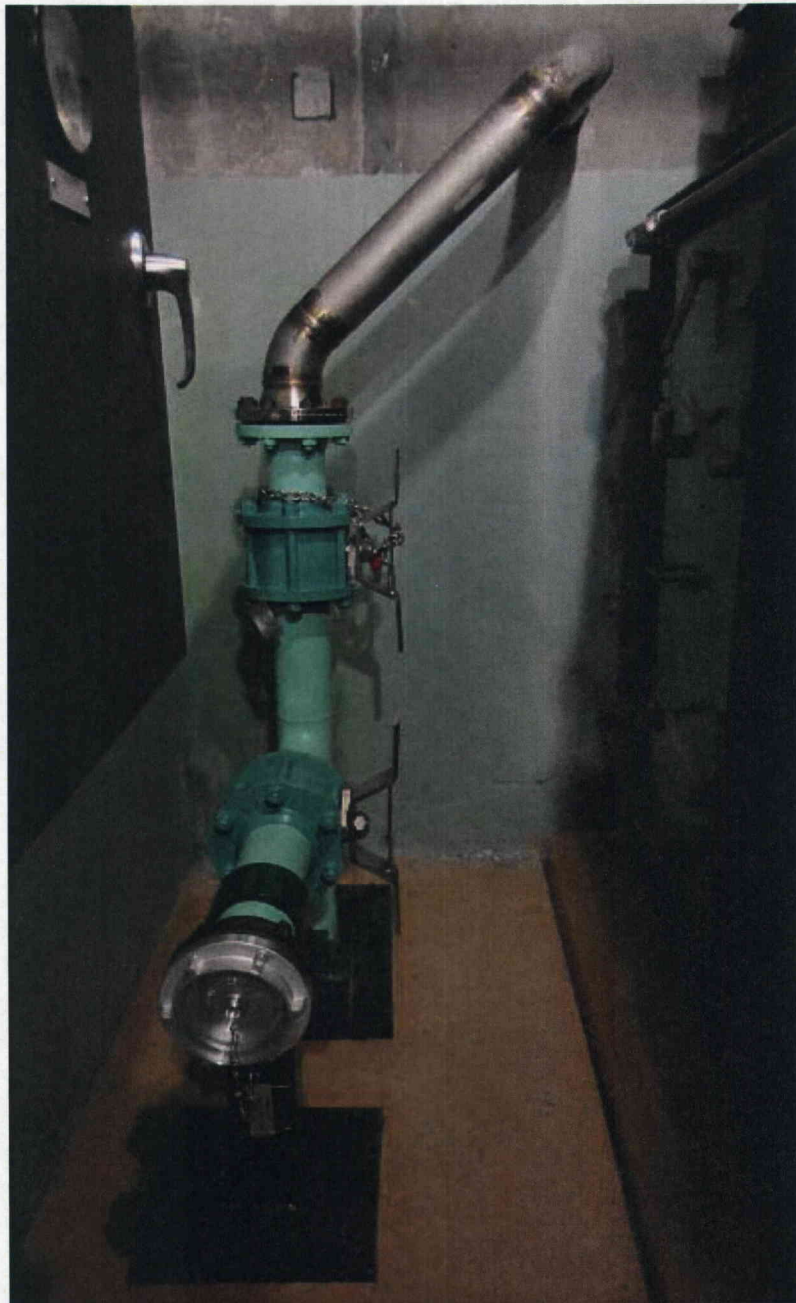
Spent Fuel Pool Fill Connection Intermediate Building 620 foot elevation
