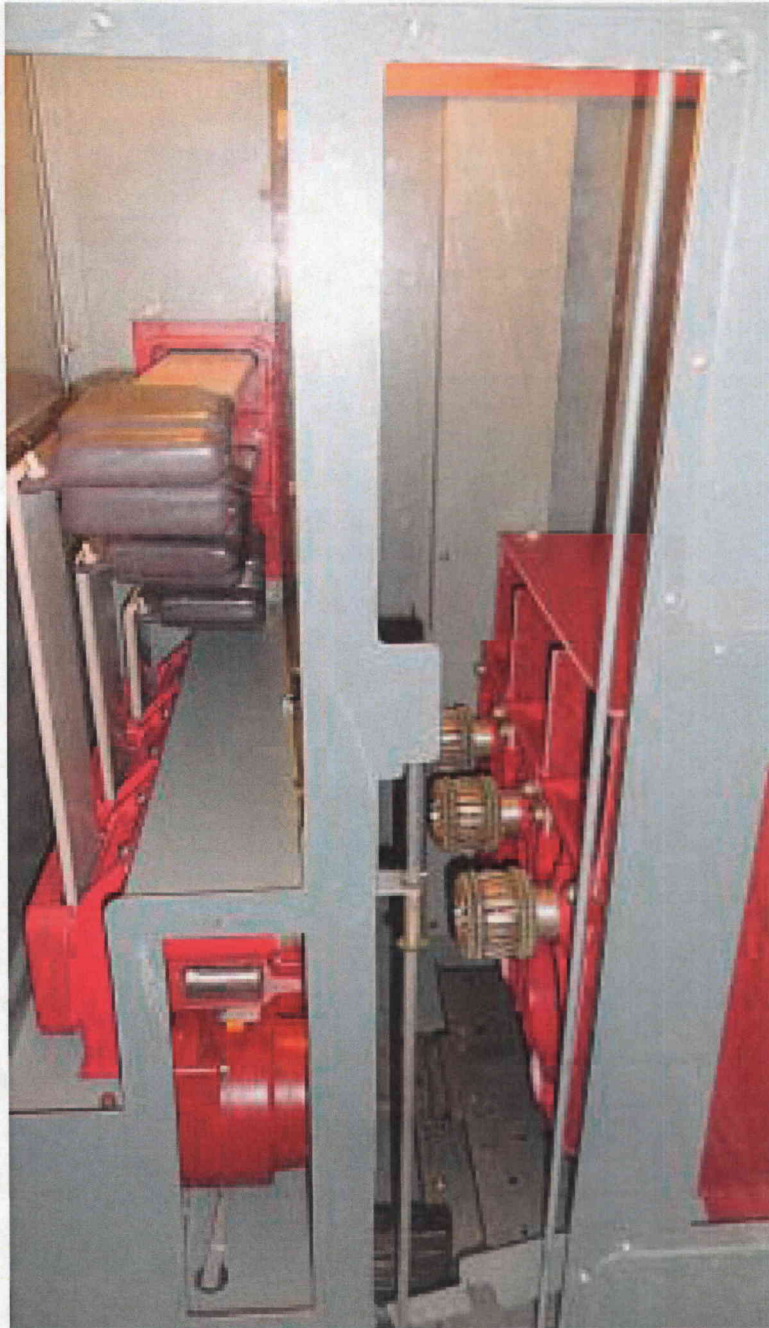
Emergency Buss Feeder side view being racked in during testing at Maintenance training facility, note: Plexiglas covers over side of panel
