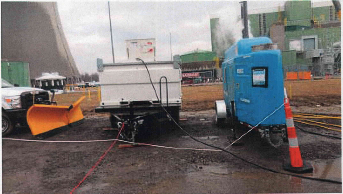
Debris Removal Truck, Transcube and FLEX 4160 Vac generator at ESW Pumphouse for FLEX Lake Water Pump Testing
