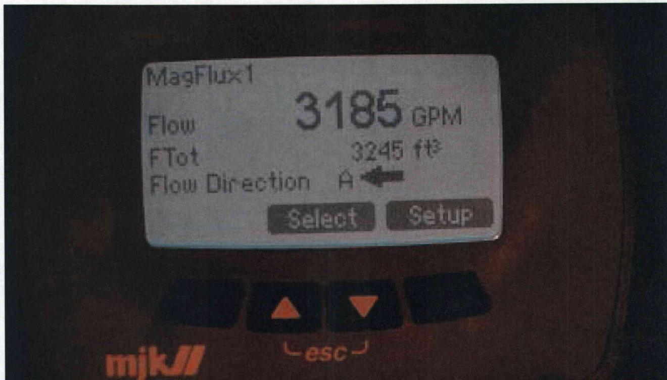
FLEX Lake Water Pump control panel during testing
