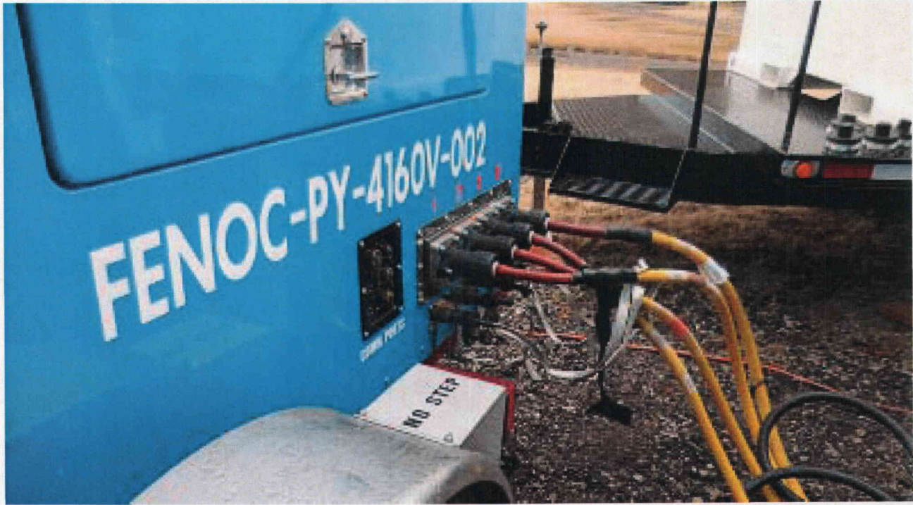
Cables connected to 4160 Vac Generator during FLEX Lake Water Pump Testing
