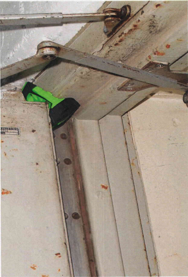
FLEX Door blocking device in use holding open door to ESW Pumphouse for 4160 Vac cables during FLEX Lake Water Pump testing
