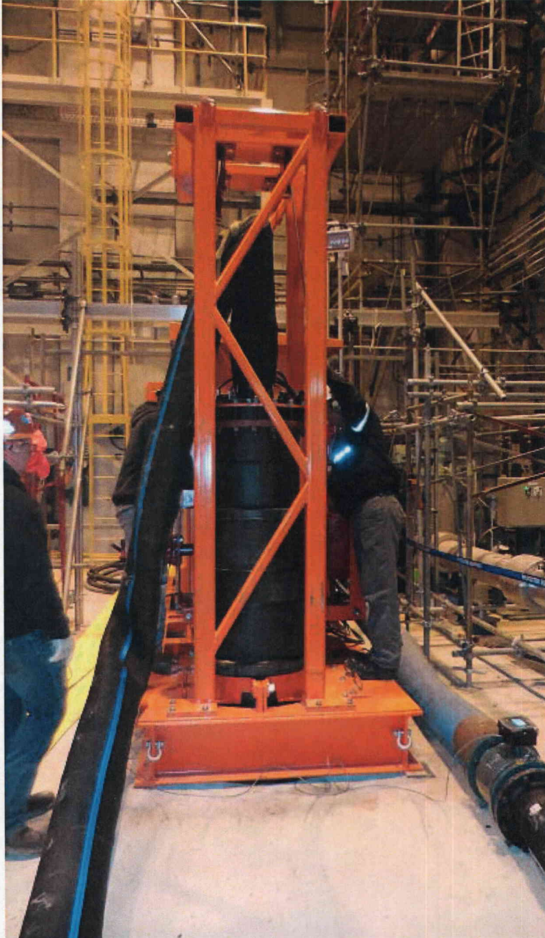
FLEX Lake Water Pump in stand, flow test meter installed at right of photo
