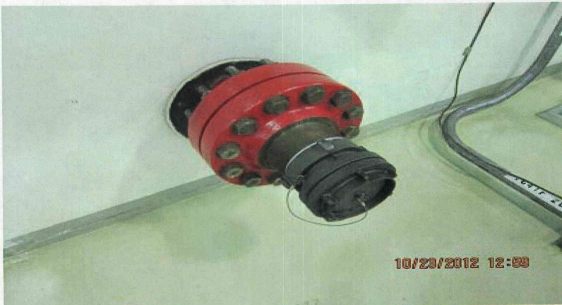
HPCS Connection Auxiliary Building 620 foot elevation west side
