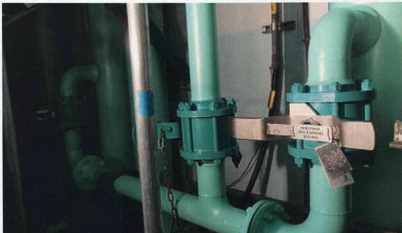
ESW Loops A (right) and B (left) connection to Spent Fuel Pool fill line (center)
