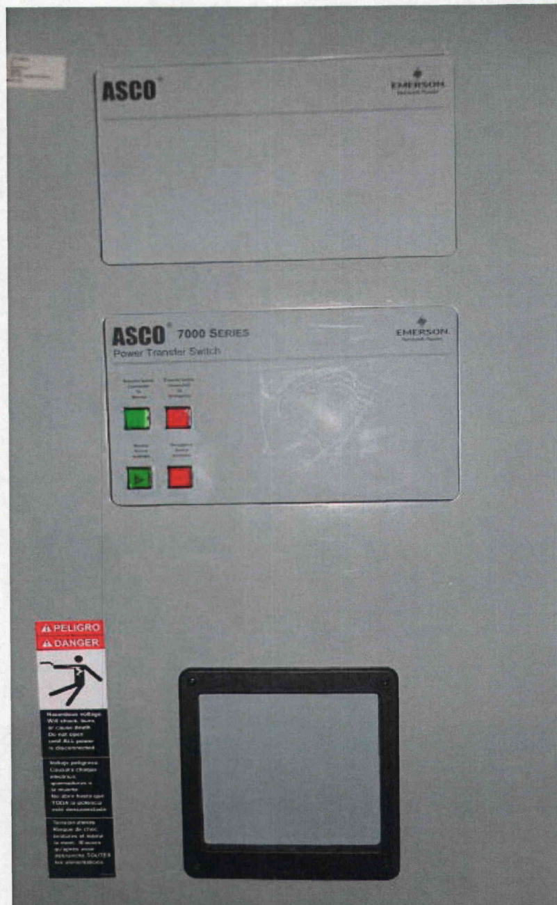
Suppression Pool Cleanup Power Transfer Switch
