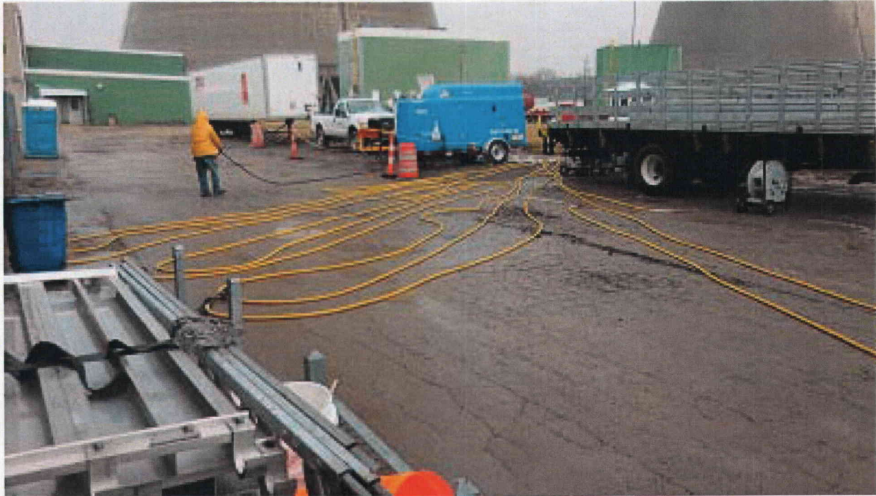
Cables laid out at ESW Pumphouse during FLEX Lake Water Pump testing
