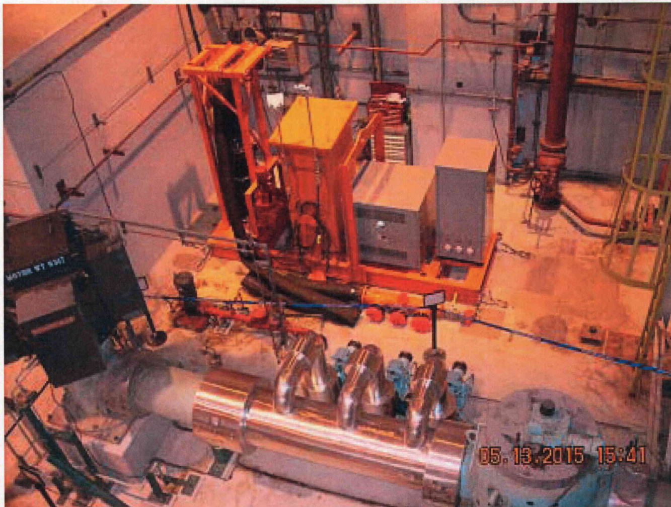
FLEX Lake Water Pump with distribution header attached, A side
