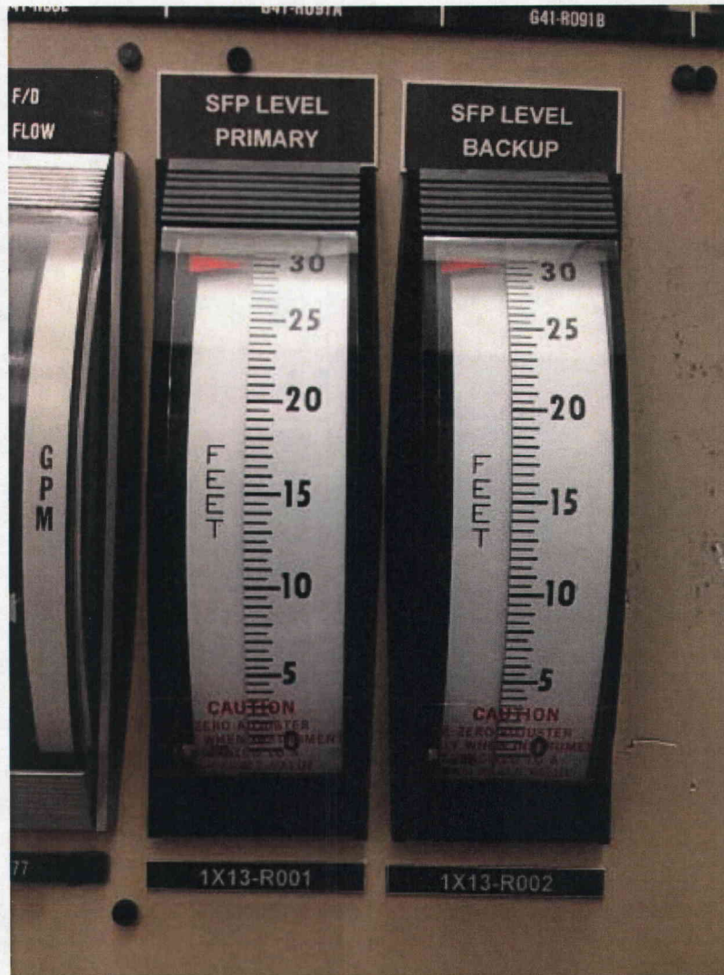
Control Room Spent Fuel Pool Level Indication
