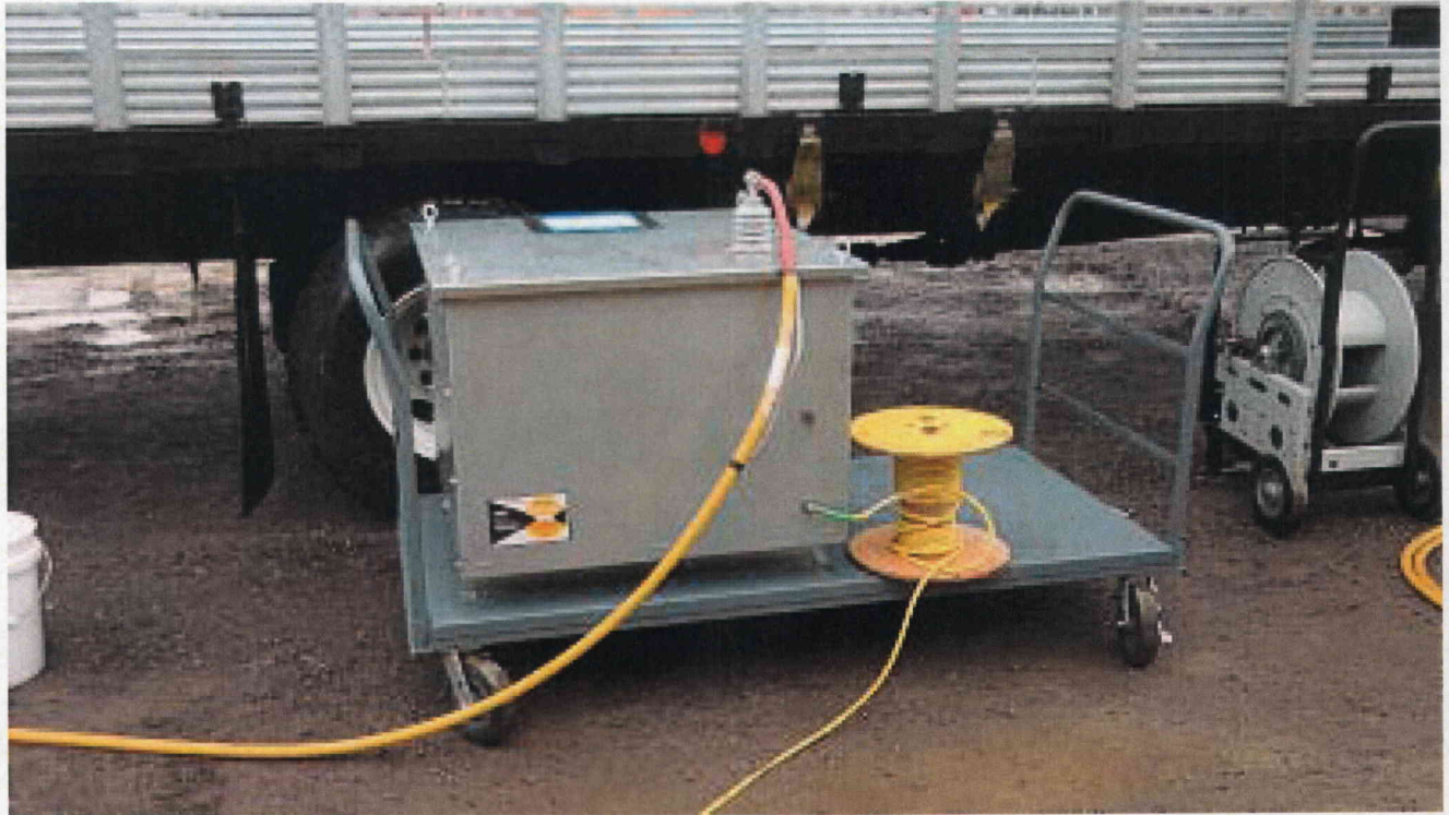
Neutral Ground Resister connection during 4160 Vac Generator run for FLEX Lake Water Pump Testing
