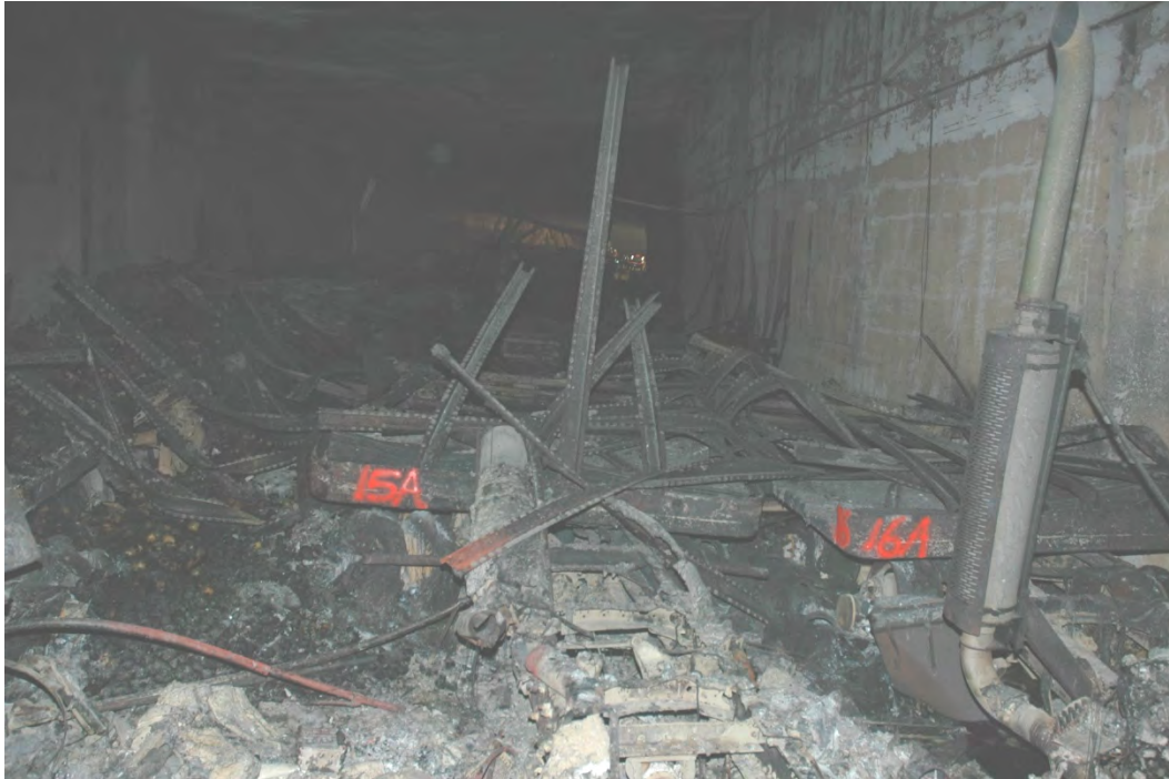
12 13 Figure 2.7. Vehicles Near Middle of Tunnel, View Toward Tunnel Entrance (photo from MAIT 14 Report, CHP 2007, reprinted with permission.) 15
