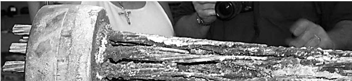
Figure 3-8 Corrosion observed near ends of tendons from the Sunshine Skyway Bridge
