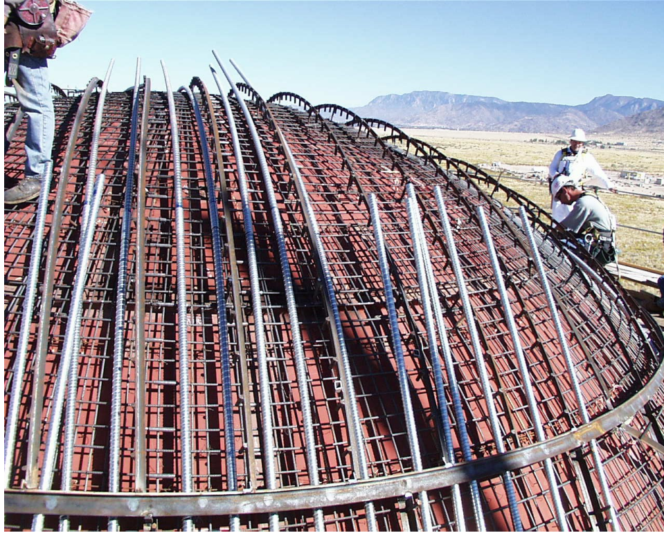
Figure 2-11 Tendon ducts (silver colored tubes) in 1:4-scale PCCV with and without connections as well as traditional rebar
