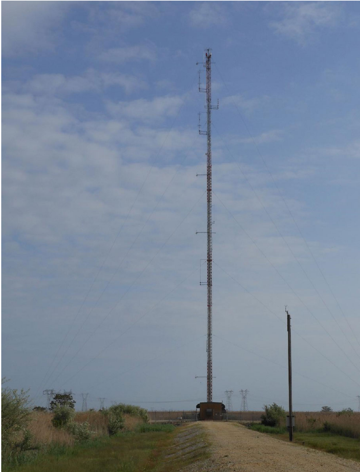
Figure 2-34. Existing PSEG Meteorological Tower and Meteorological Building with Backup Meteorological Tower in Foreground (Source: NRC staff photograph)
