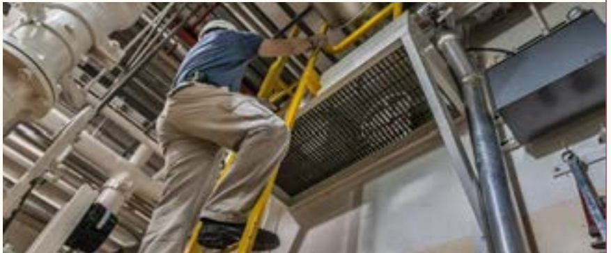
An NRC inspector conducts routine inspections of plant equipment to ensure the plant is meeting NRC regulations.
