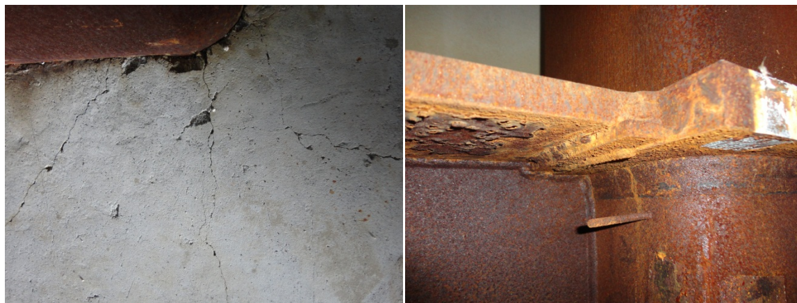
Figure 2-11 Cracks in concrete slab and rust on steel member.
