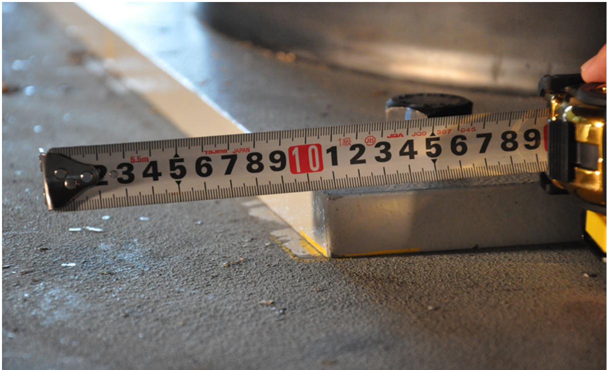
Figure 5-12 Permanent displacement of around 1.1 cm on the East bearing due to sliding of the bottom steel plate
