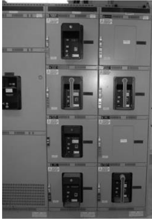
Figure C-9 Front View of Load Center (Low Voltage Switchgear)
