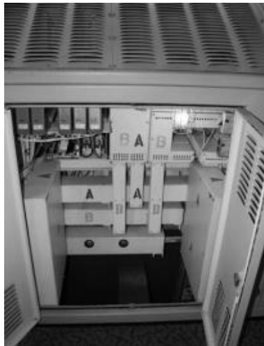
19 Figure 4-4 20 Photograph of Metal Enclosed Wire-Ways Within Electrical Enclosure (MCB)
