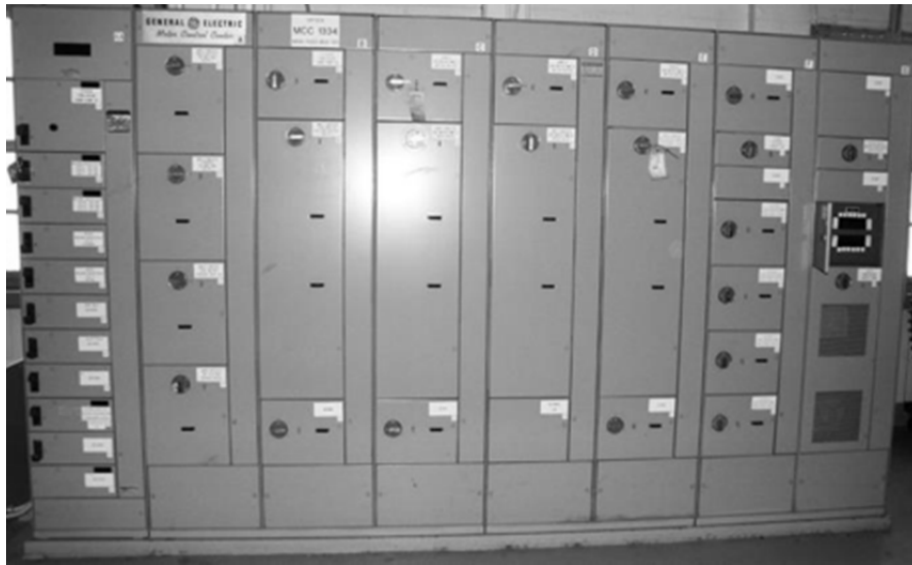
8 9 10 Figure 3-3 11 A Typical Bank of MCC Cabinets
