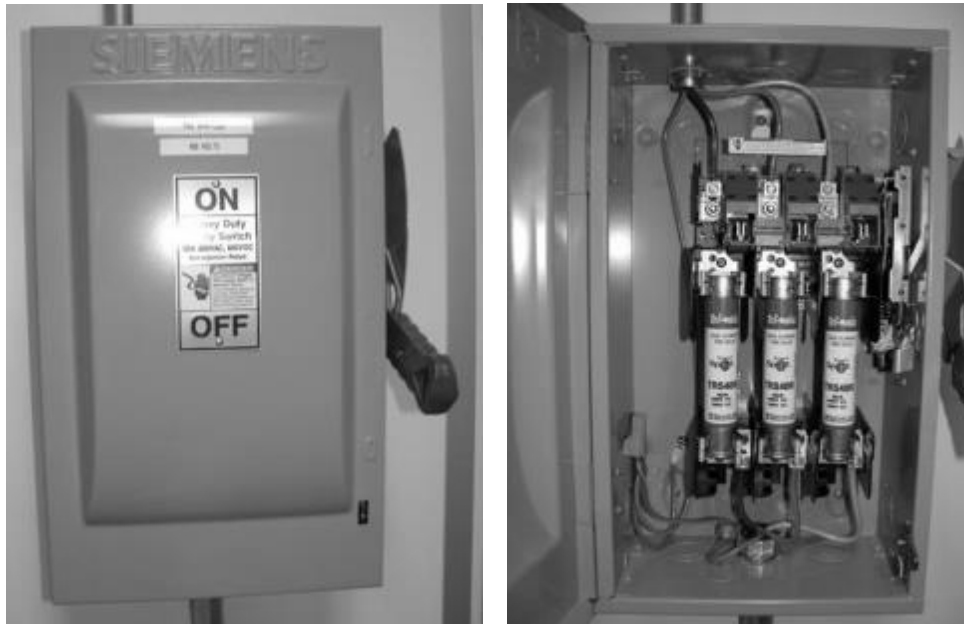
10 11 12 13 14 Figure C-23 15 Wall Mounted Low Voltage AC Fused Disconnect Switches 16 17 18
