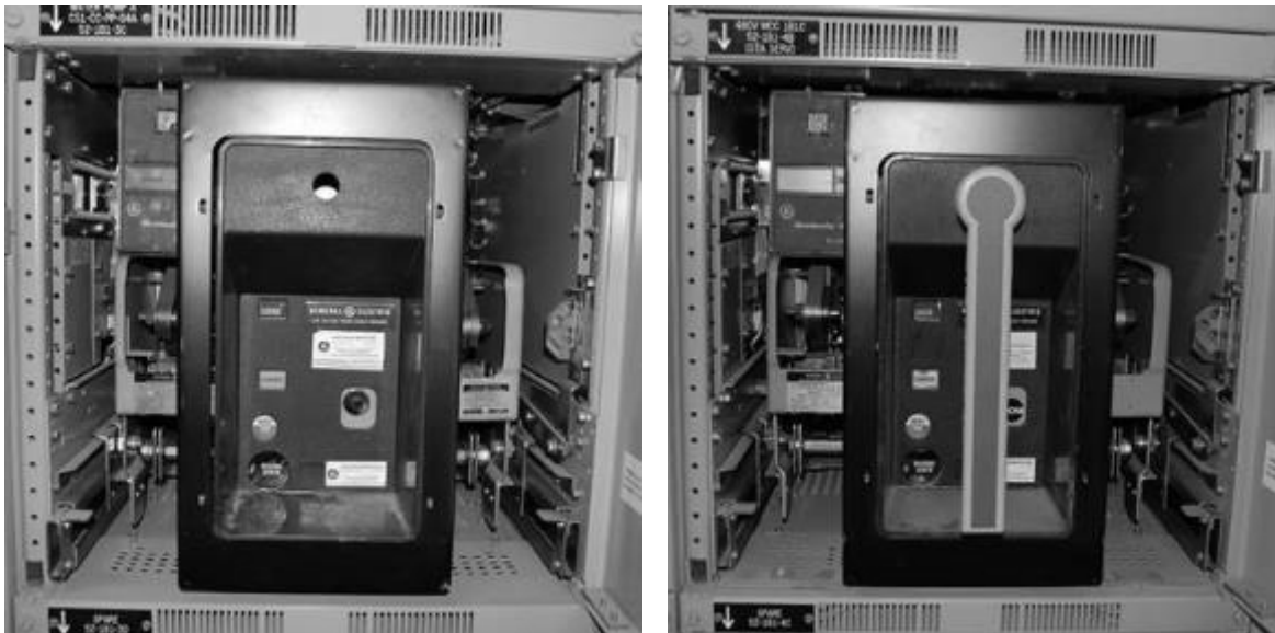
Figure C-10 Low Voltage Load Center Breaker
