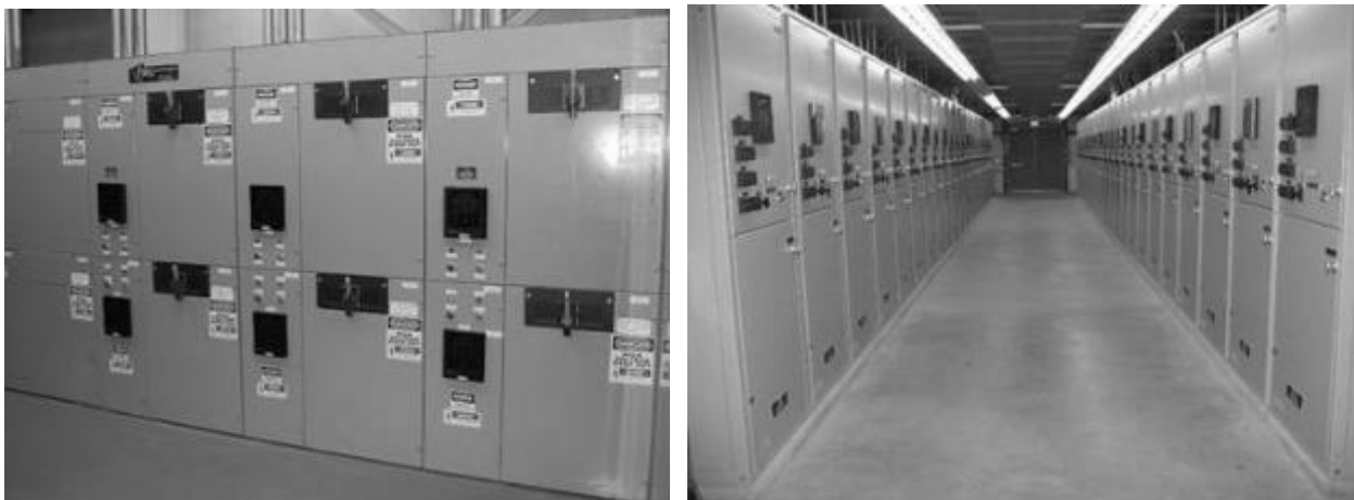
Figure C-1 Front View of Medium Voltage Switchgear Banks
