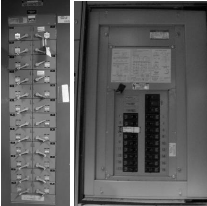
Figure C-24 125 VDC Distribution Panel (Left) and 120 VAC Distribution Panel (Right)
