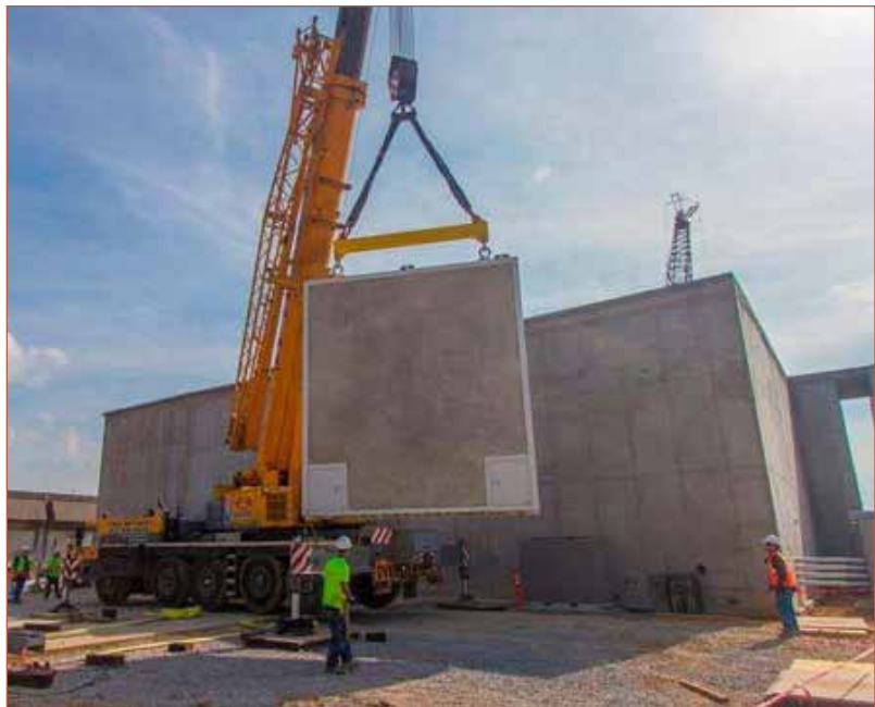
Photo courtesy of Tennessee Valley Authority
