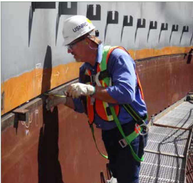
Top, NRC Resident Inspector Patrick Donnelly inspects the V.C. Summer Unit 3 nuclear island rebar.
