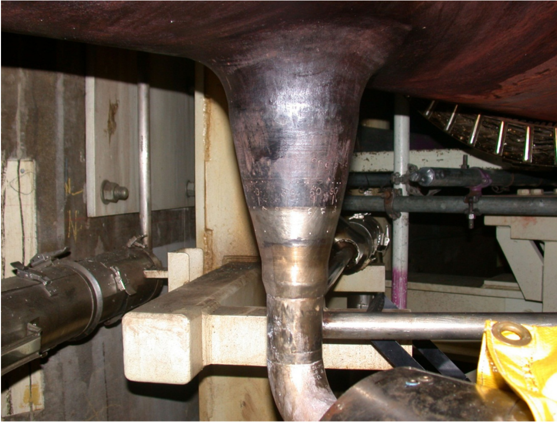
Figure D.11 Photograph of Letdown and Drain Nozzle, Nozzle Weld, and Safe End
