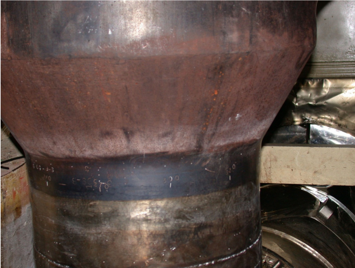
Figure D.23 Photograph of Shutdown Cooling Nozzle, Nozzle Weld, and Safe End
