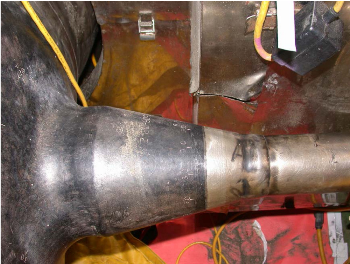
Figure D.26 Photograph of Spray Nozzle, Nozzle Weld, and Safe End
