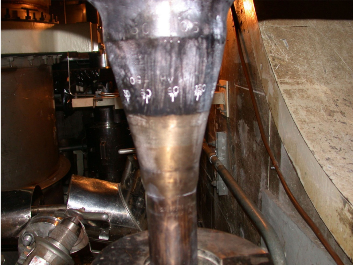
Figure D.14 Photograph of Hot Leg Drain Nozzle, Nozzle Weld, and Safe End
