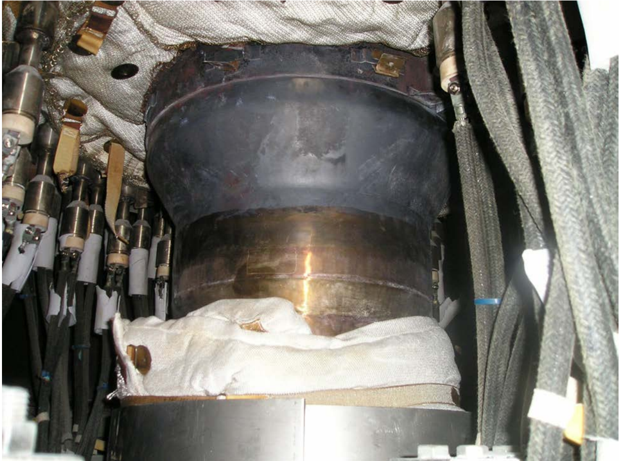
Figure C.2 Photograph of Pressurizer Surge Nozzle, Nozzle Weld, and Safe End
