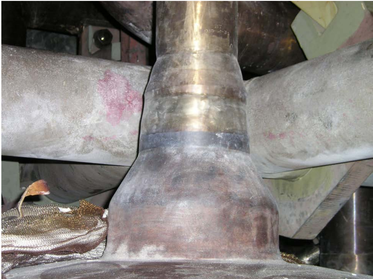
Figure C.5 Photograph of Pressurizer Spray Nozzle, Nozzle Weld, and Safe End
