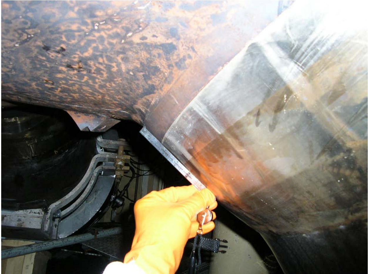
Figure C.13 Photograph of Steam Generator Hot Leg Nozzle, Nozzle Weld, and Safe End
