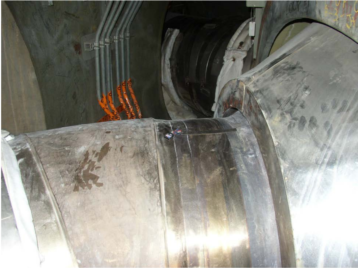
Figure C.19 Photograph of RPV Cold Leg Nozzle
