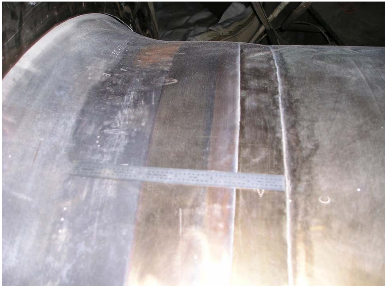
Figure C.10 RPV Hot Leg Nozzle, Nozzle Weld, and Safe End
