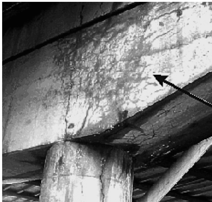
Figure 4.7. Cracking damage in a concrete structure due to DEF [91].
