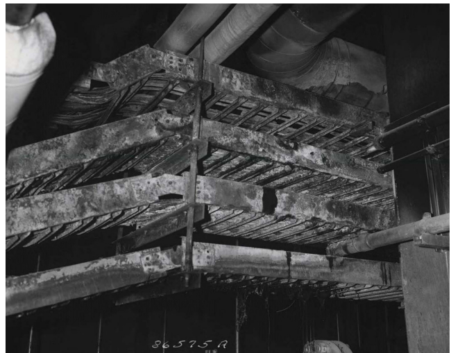
Figure 7: The Browns Ferry fire damaged hundreds of safety-related electrical cables. It underscored the need for fire-safety training and greater safety research.
