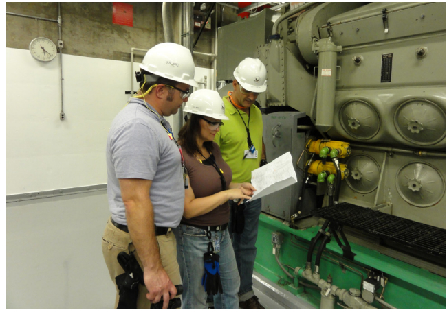
Figure 6: Critical to avoiding a station blackout are the power plant's emergency diesel generators, such as the one pictured here. In 1988, the NRC developed a new rule on station blackouts and guidance on diesel generator performance.
