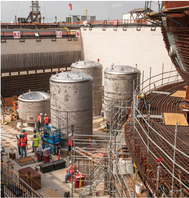
Top, Construction Resident Inspector Dave Failla observes the V.C. Summer Unit 2 containment vessel bottom head lift.
