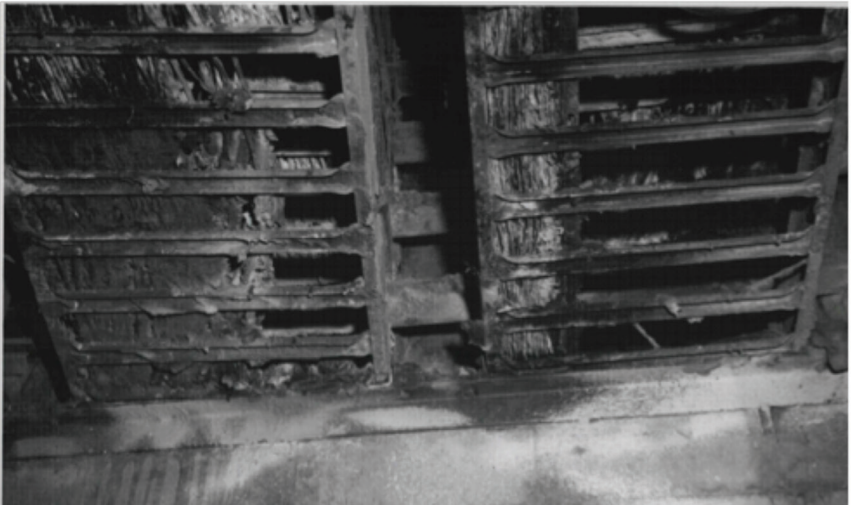
The Browns Ferry (BFN) cable tray penetration after the 1975 fire. The fire forever changed how the NRC and industry view the threat of fire (NUREG/KM-0002).
