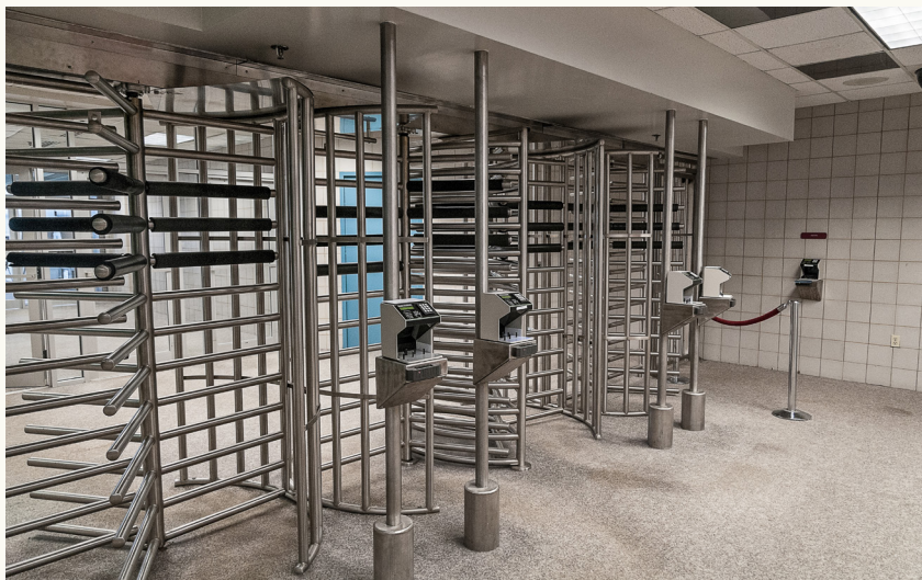
Access control security gates within a nuclear facility provide another layer of protection.
