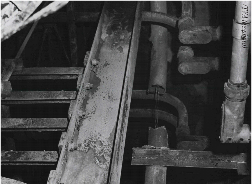
Picture of Browns Ferry Fire Cable Spreading Room. Note the melted aluminum electrical cable conduit.
