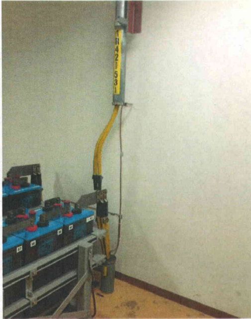
File Name: 2-73-4-4-02.jpeg Description: View of attached line
