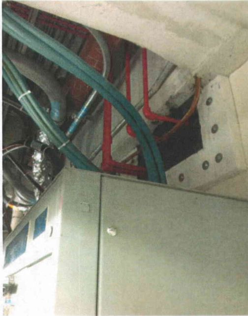
File Name: 2-73-10-4-22.jpeg Description: View of top attached lines
