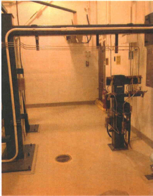
File Name: 2-63-11-1-08.jpeg Description: General view with attached lines
