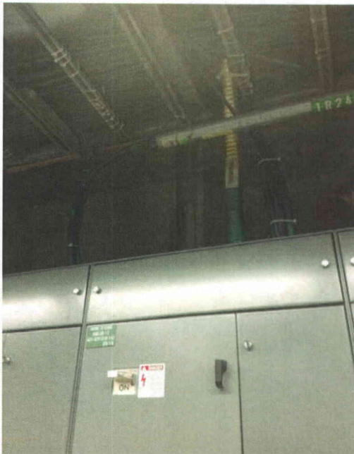
File Name: 2-64-7-4-22.jpeg Description: View of top attached lines
