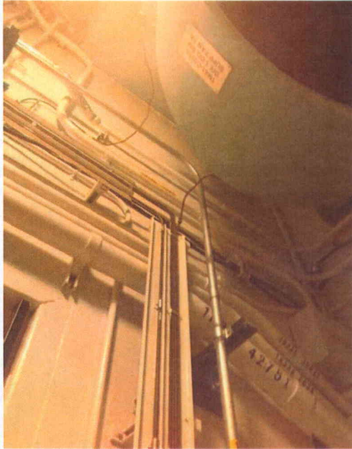
File Name: 2-63-18-4-08.jpeg Description: View of attached small lines
