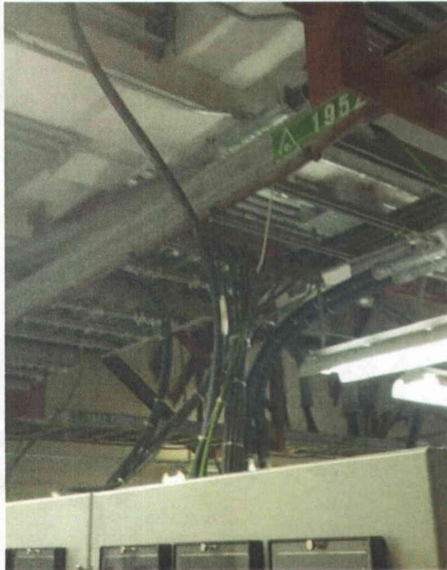
File Name: 2-63-4-4-06.jpeg Description: View of attached lines
