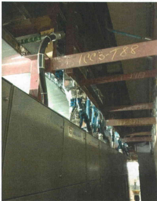
File Name: 2-64-6-4-22.jpeg Description: View of top attached lines
