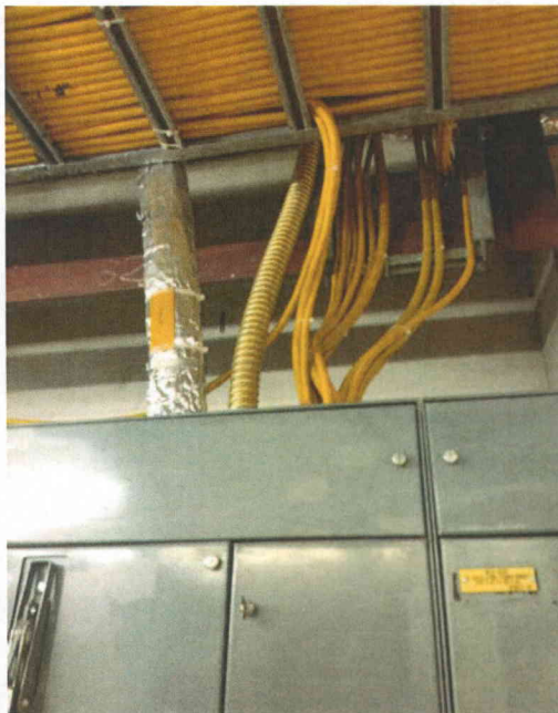
File Name: 2-64-12-4-06.jpeg Description: View of top attached lines
