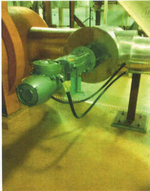
File Name: 2-73-2-1-01.jpeg Description: Main line support and attached lines
