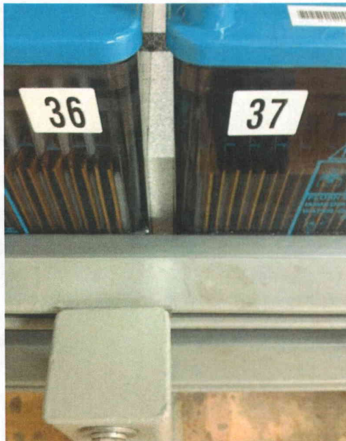
File Name: 2-94-4-4-02.jpeg Description: View of battery cells separation
