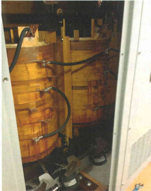
File Name: 2-63-1-4-06.jpeg Description: View of transformer coils inside cabinet
