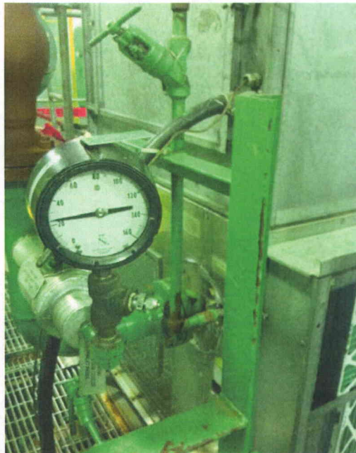
File Name: 2-64-15-4-18.jpeg Description: View of attached lines
