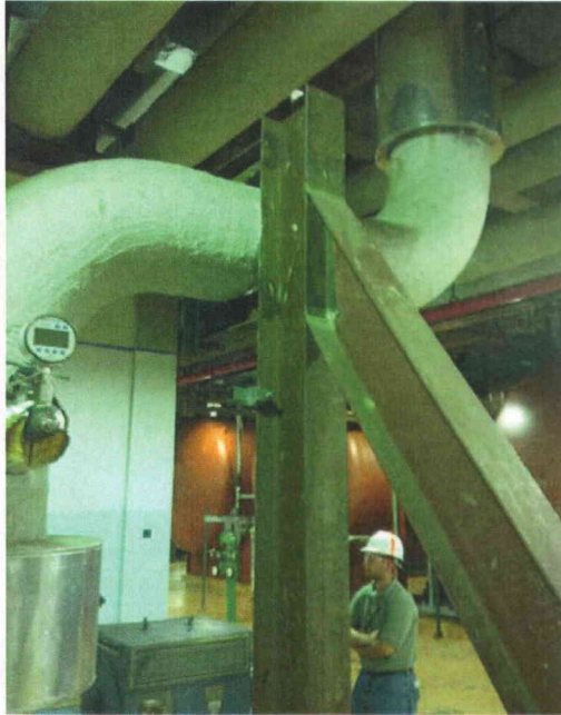
File Name: 2-63-4-4-01.jpeg Description: View of main pipe line bracing
