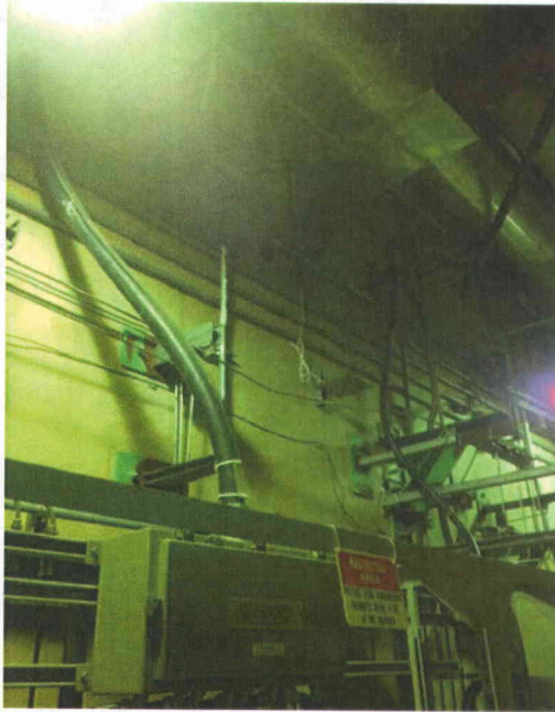
File Name: 2-73-6-4-18.jpeg Description: View of top attached lines
