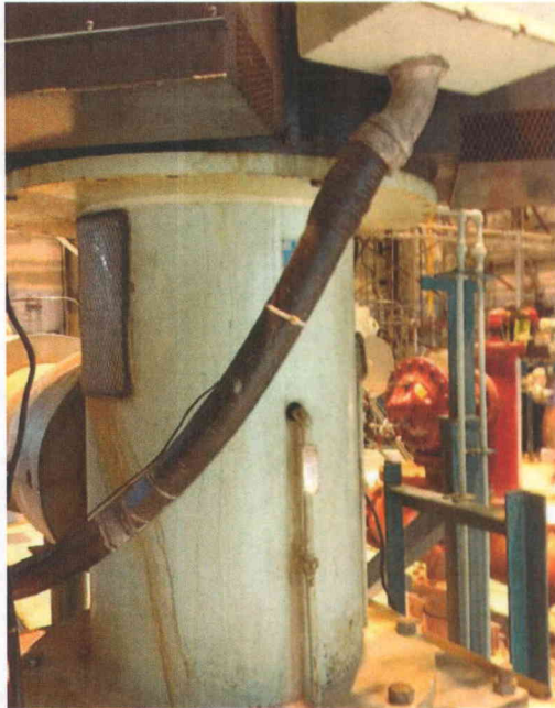
File Name: 2-63-7-4-05.jpeg Description: View of attached lines
