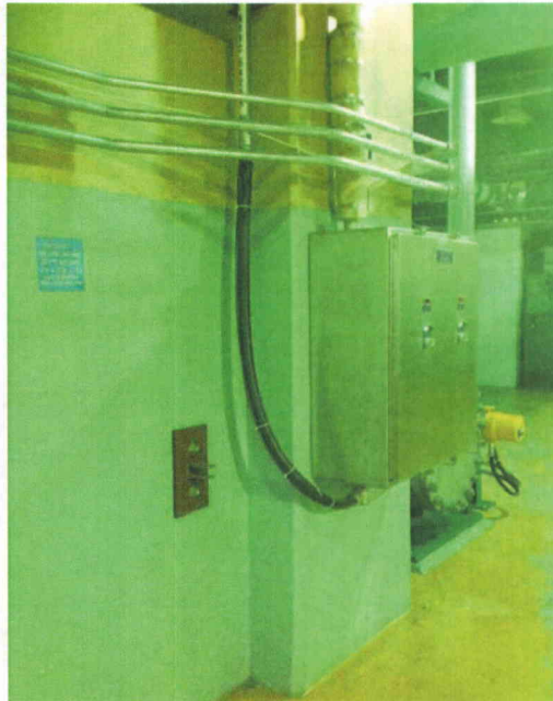
File Name: 2-64-3-4-22.jpeg Description: View of attached line
