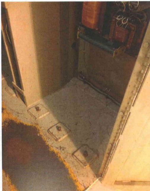
File Name: 2-96-10-4-08.jpeg Description: View of anchorage detail from inside of cabinet
