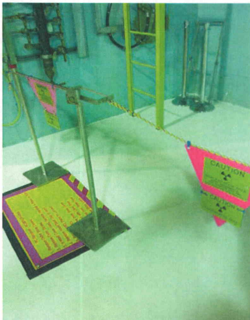
File Name: 2-62-4-4-18.jpeg Description: High radiation area signage
