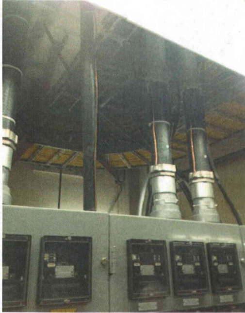
File Name: 2-63-9-4-06.jpeg Description: View of top conduits
