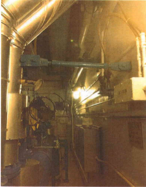
File Name: 2-73-9-4-08.jpeg Description: View of lateral wall-mounted support
