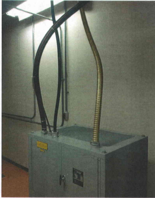
File Name: 2-73-13-4-06.jpeg Description: View of top attached lines
