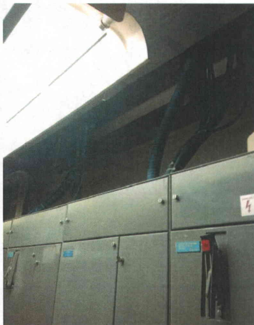
File Name: 2-64-5-4-22.jpeg Description: View of top attached lines
