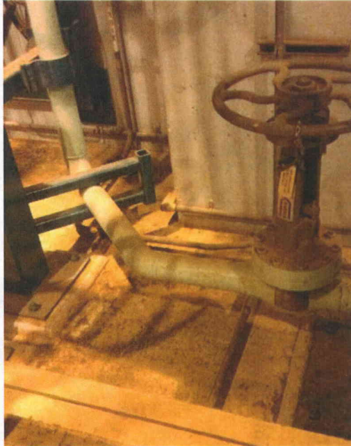
File Name: 2-63-5-4-05.jpeg Description: View of pipe line supports
