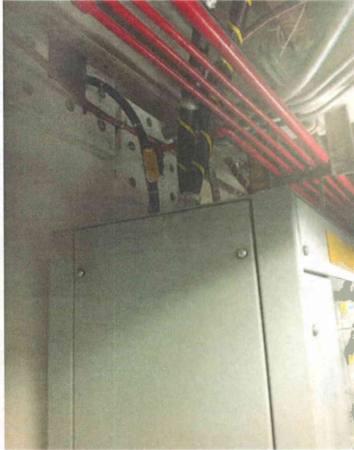
File Name: 2-73-8-4-22.jpeg Description: View of top attached lines
