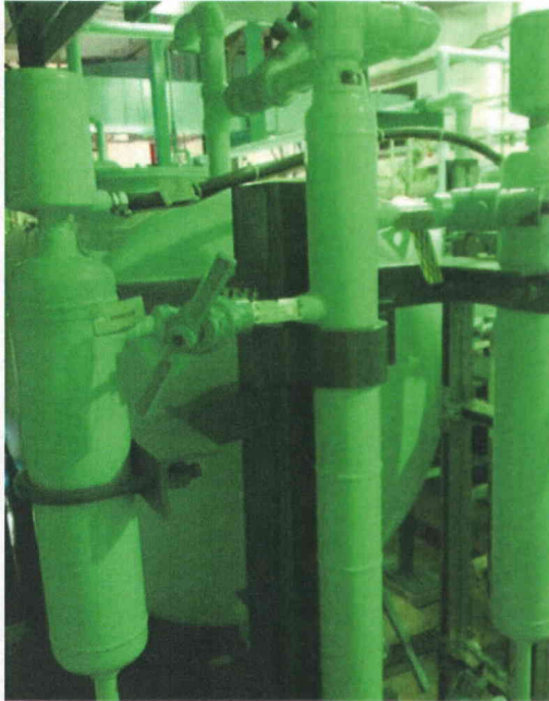
File Name: 2-63-1-4-11.jpeg Description: View of pipe line lateral supports
