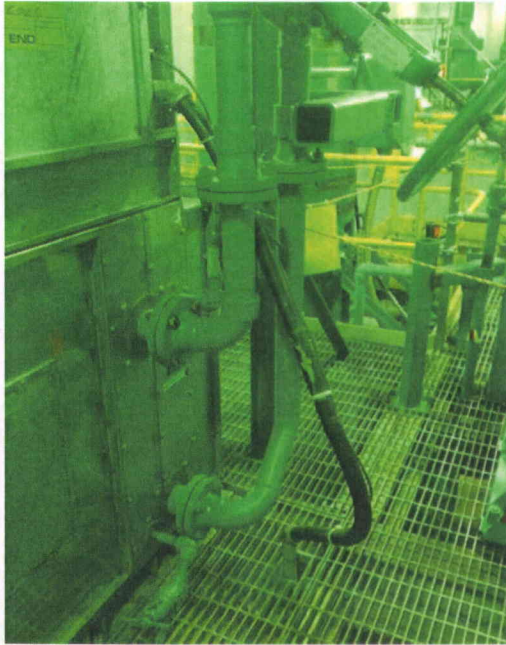
File Name: 2-73-9-4-18.jpeg Description: View of pipe lines attached to component
