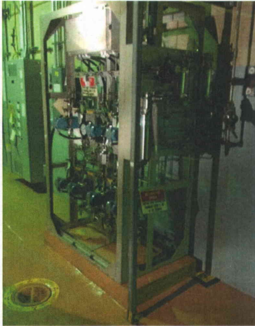
File Name: 2-63-7-4-18.jpeg Description: General view of component rack
