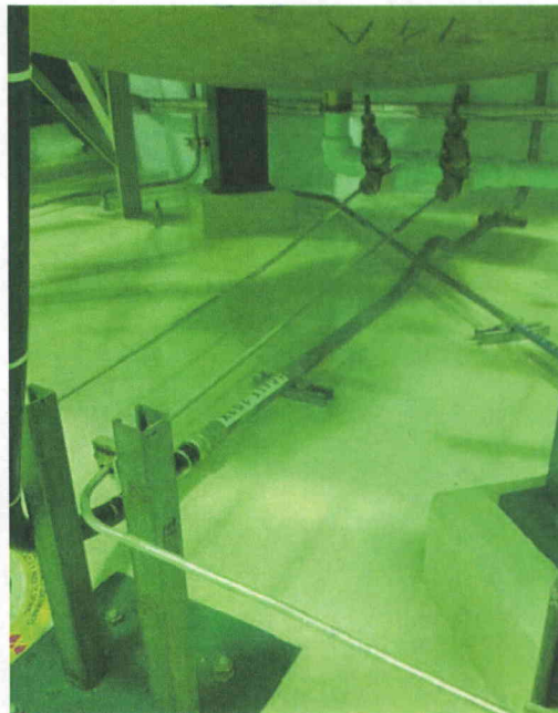
File Name: 2-64-1-4-09.jpeg Description: View of attached lines
