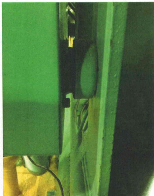
File Name: 2-63-1-1-01.jpeg Description: Isolator close up
