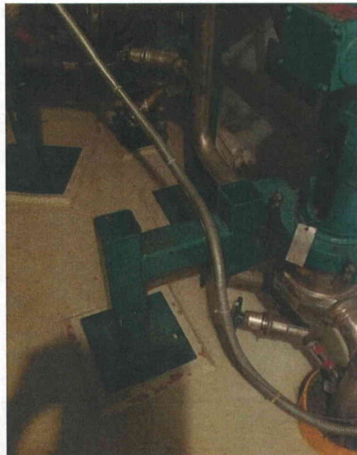
File Name: 2-64-1-4-17.jpeg Description: View of attached line
