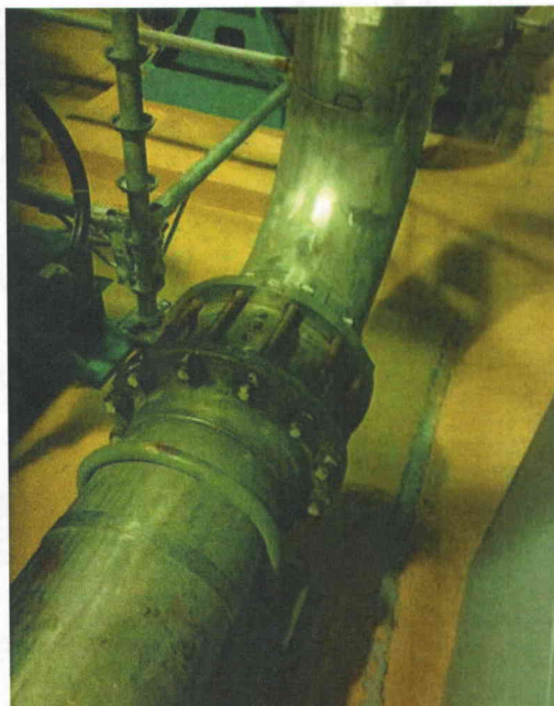
File Name: 2-62-3-4-21.jpeg Description: View of valve location in pipe main line
