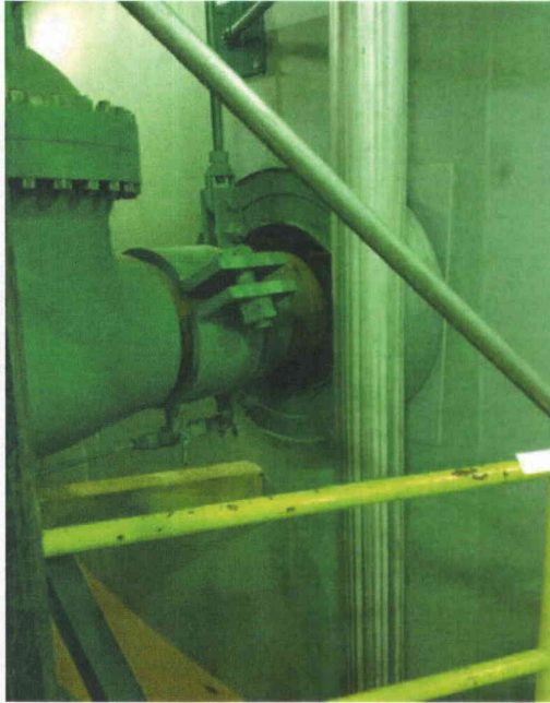
File Name: 2-63-8-4-18.jpeg Description: View of main pipe line run through shield building
