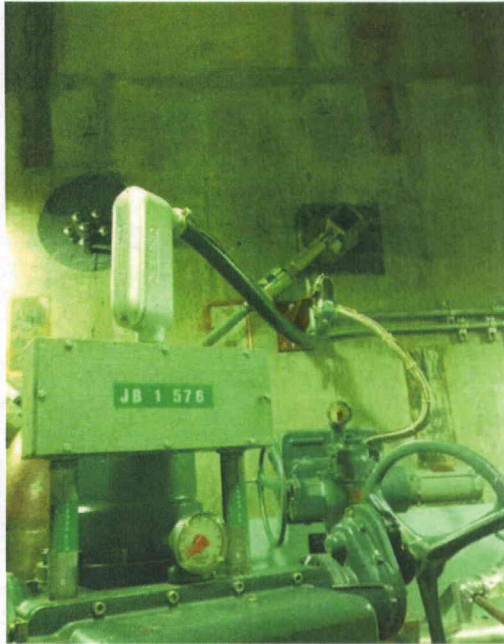
File Name: 2-63-1-4-10.jpeg Description: View of attached lines
