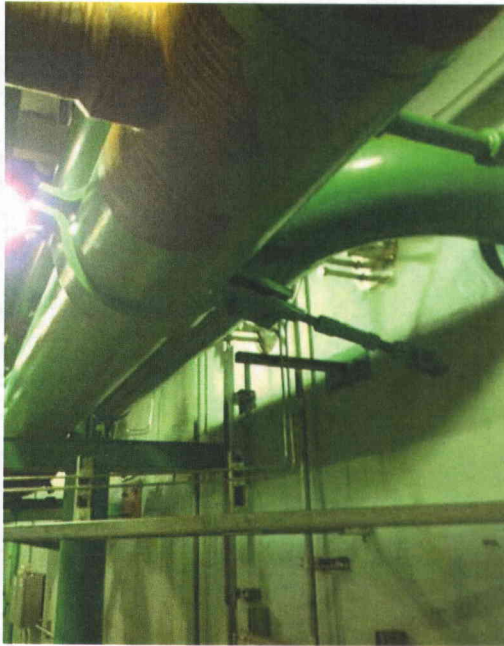
File Name: 2-63-13-4-18.jpeg Description: View of pipe line lateral supports
