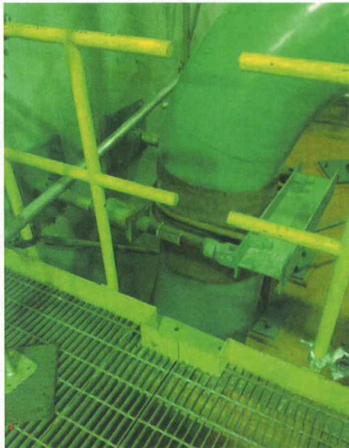
File Name: 2-94-8-4-18.jpeg Description: View of main pipe line support configuration
