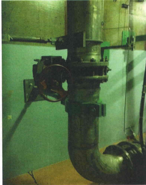
File Name: 2-63-8-1-21.jpeg Description: View of pipe line support configuration
