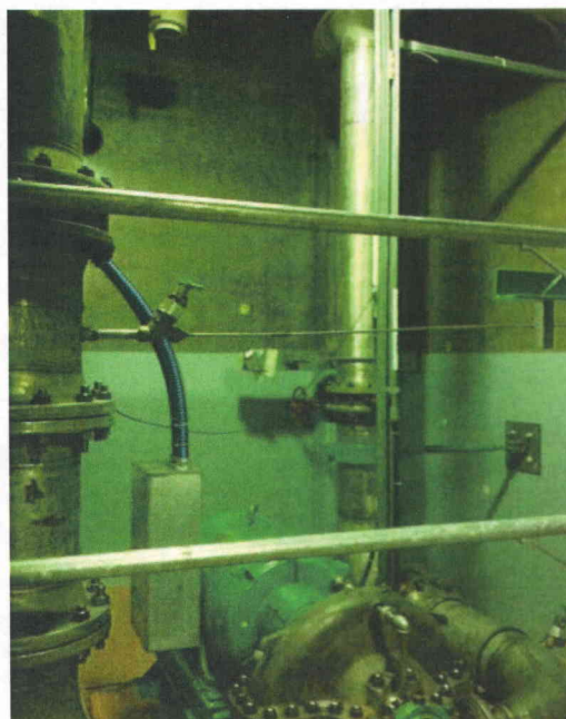
File Name: 2-62-1-4-21.jpeg Description: View of attached lines
