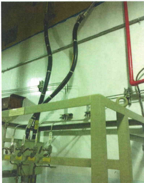
File Name: 2-64-7-4-01.jpeg Description: View of attached top lines
