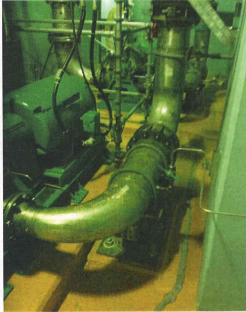
File Name: 2-63-3-4-21.jpeg Description: View of main pipe line connected to component
