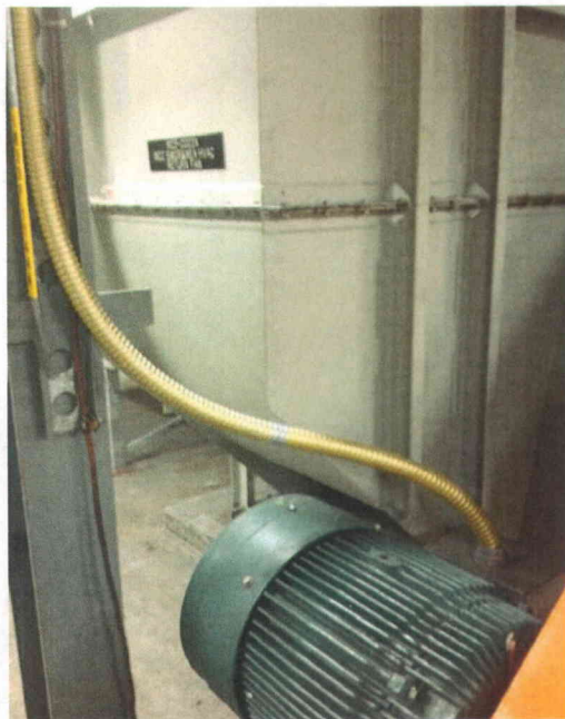
File Name: 2-73-3-4-04.jpeg Description: View of attached line
