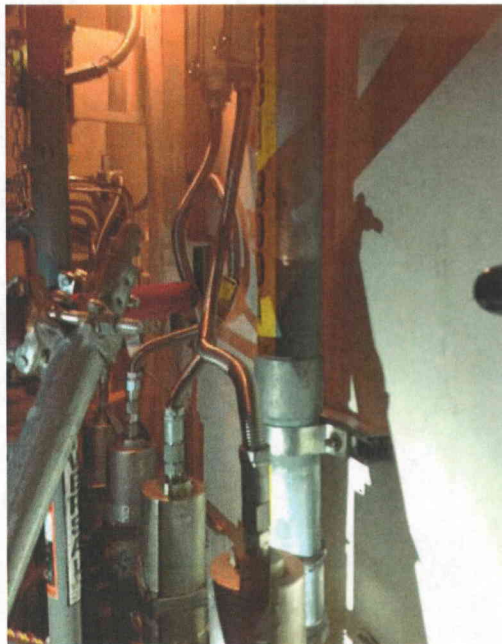
File Name: 2-62-3-4-12.jpeg Description: View of attached lines
