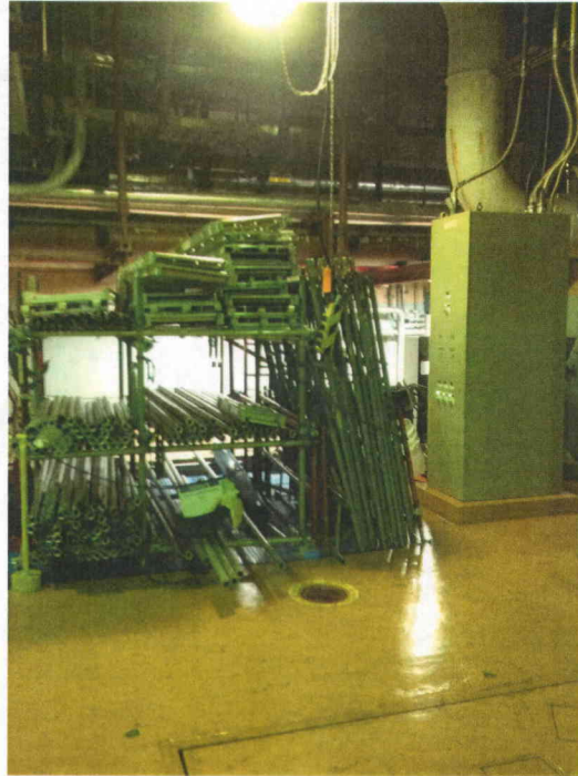
Figure 6-4: Scaffold storage rack close to HVAC control panel
