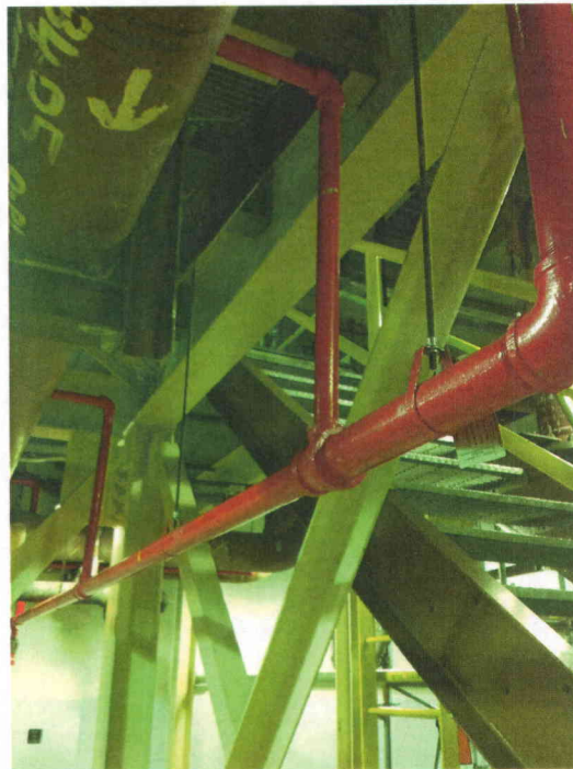
Figure 6-5: Branch lines for fire protection piping located in CC-1 at elevation 574'
