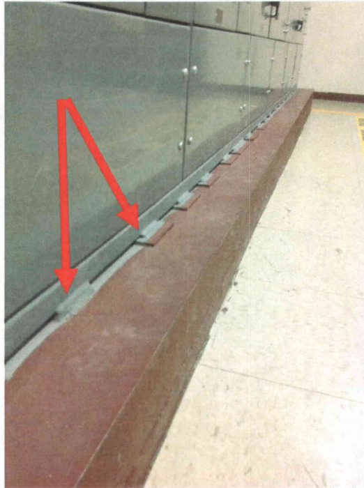
Figure 6-1: Missing shim plates on MCC embed
