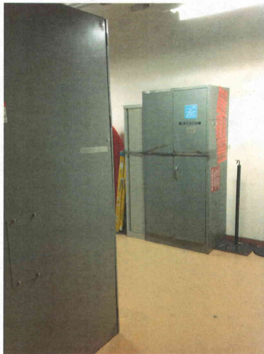
Figure 6-3: Storage locker near bus EH12
