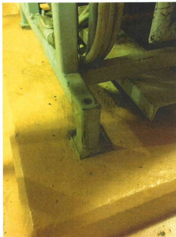
Figure 6-6: Unanchored instrument air dryers located in CC-1 on CC 574'
