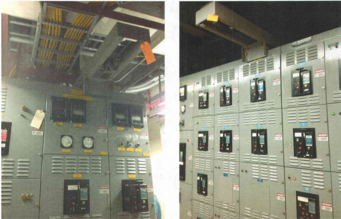
Figure 6-2: Centered trolley on top of switchgear
