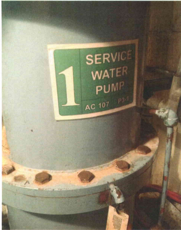
Photo 1 Minor Corrosion of Pump P3-1
