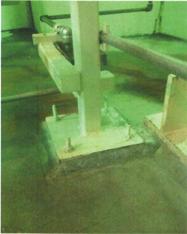
Photo 1 Anchor Threading Substantially Past Nut
