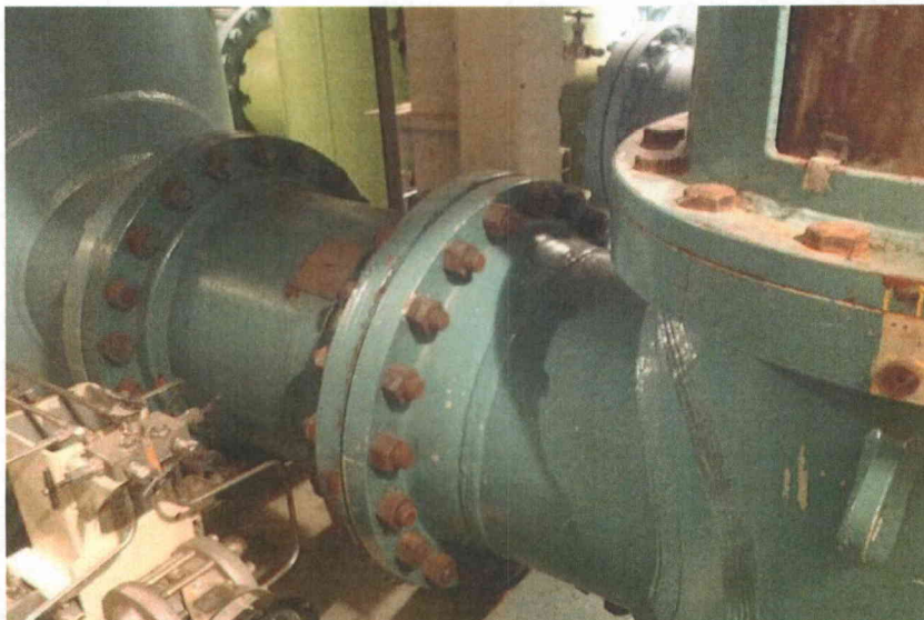
Photo 3 Minor Corrosion of Pump P3-2
