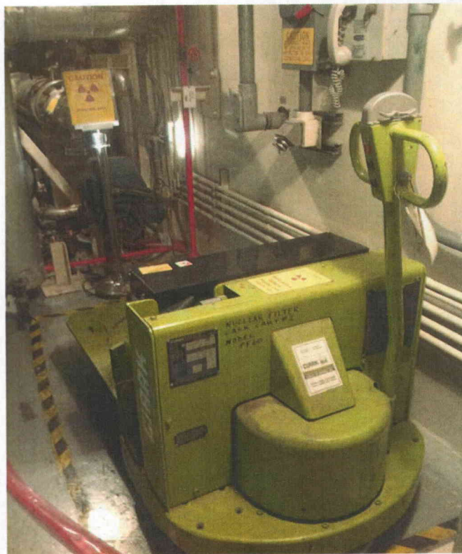
Photo 2 Nuclear Filter Cask Cart Not Restrained
