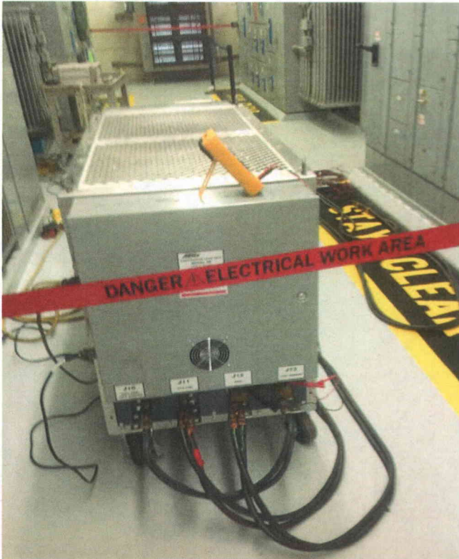
Photo 3 Unrestrained Work Cart
