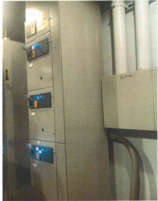
Photo 2 Movement of MCC Restrained by Adjacent Component
