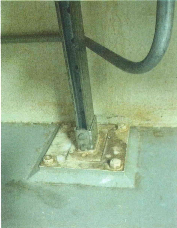
Photo 3 Minor Corrosion on Anchor Plate
