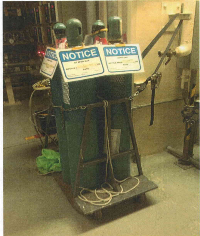
Photo 4 Cart Containing Gas Canisters Loosely Restrained
