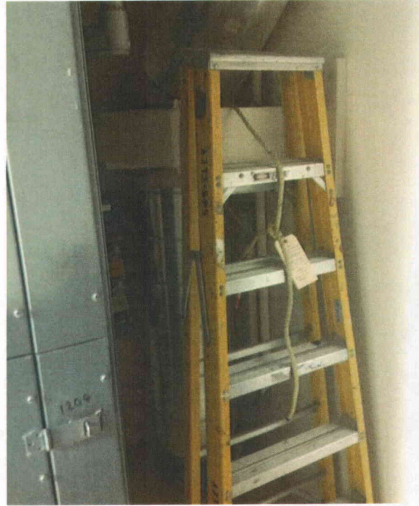
Photo 2 Ladder Loosely Tied Adjacent to MCC F11A
