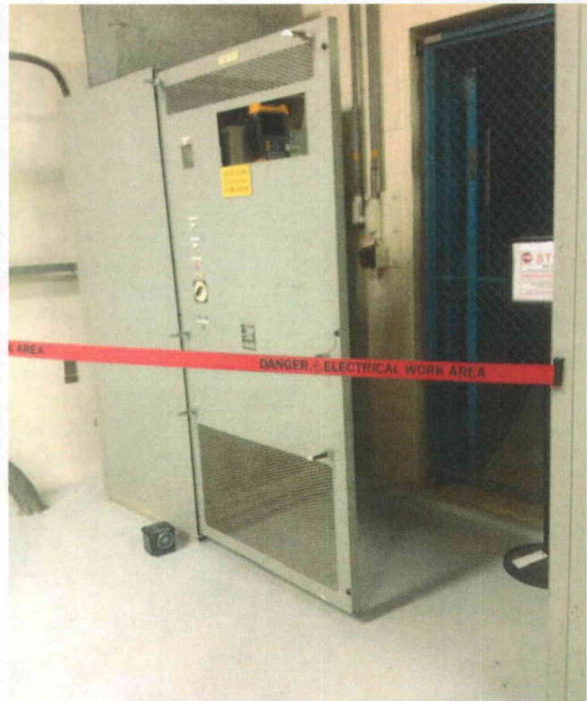
Photo 4 Cabinet DCB-2P Door Left Open
