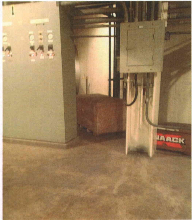
Photo 2 Unrestrained Storage Containers
