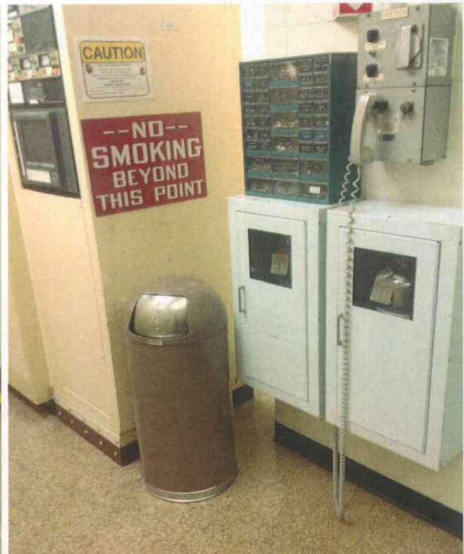
Photo 4 Unrestrained Trash Can and Light Bulb Storage
