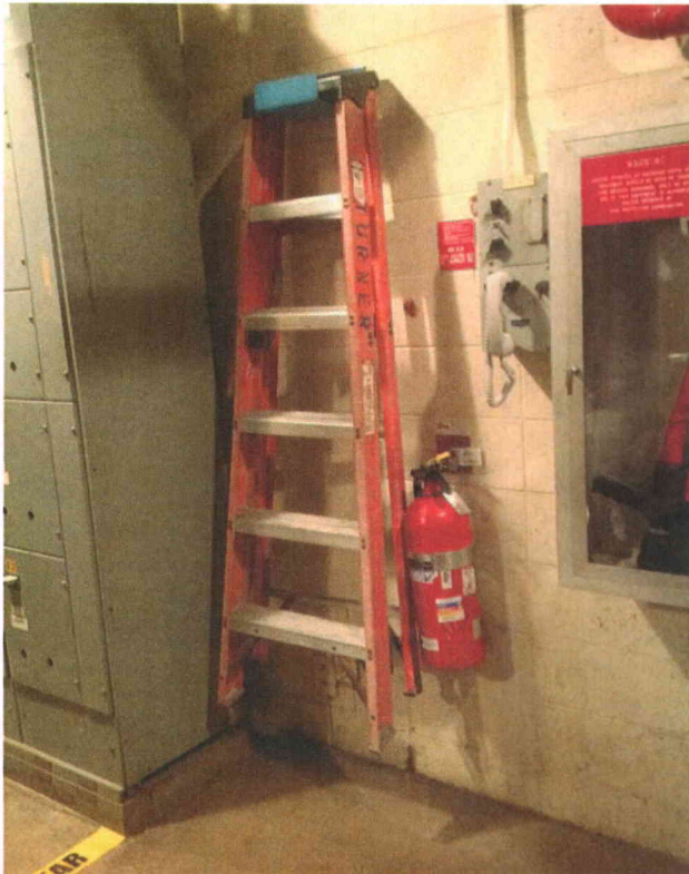
Photo 1 Fire Extinguisher not Restrained and Masonry Wall
