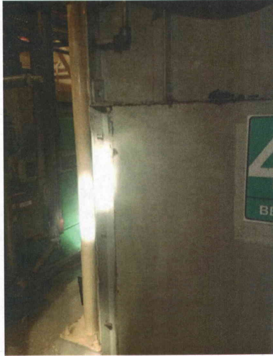
Photo 2 Missing Nuts on Cover of E31-4
