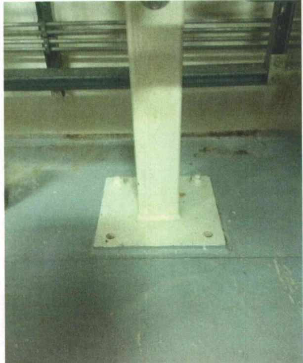
Photo 2 Missing Anchor Bolts
