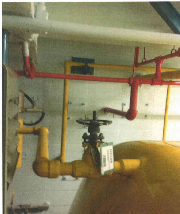
T46-1 masonry wall Potential interaction hazard from masonry wall near unit
