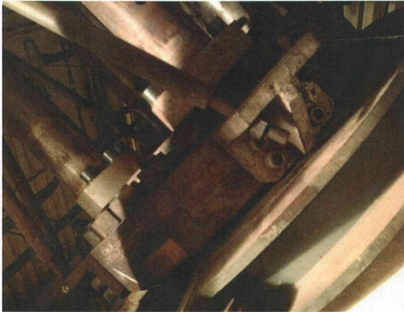
Ms101 attachment to steam pipe Valve connection to main steam line
