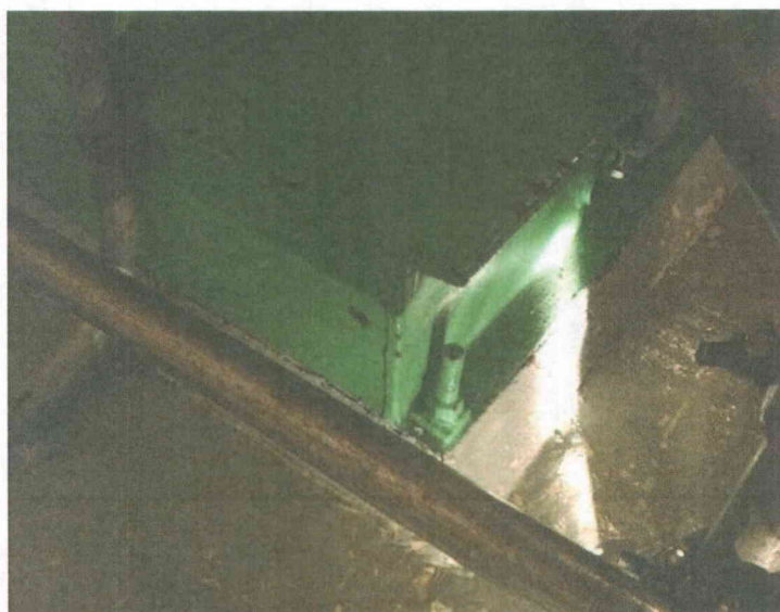
P42-1 anchorage2 Partial view of anchorage, view is typical of all anchors
