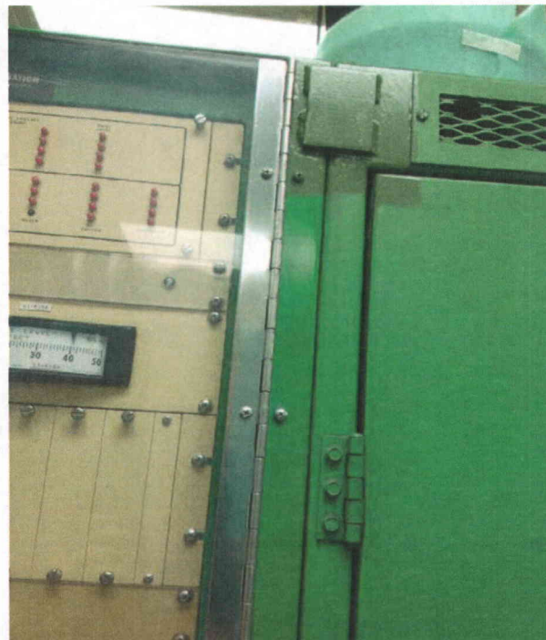
L311-511 cabinets welded together on right Cabinets are welded together on the right side
