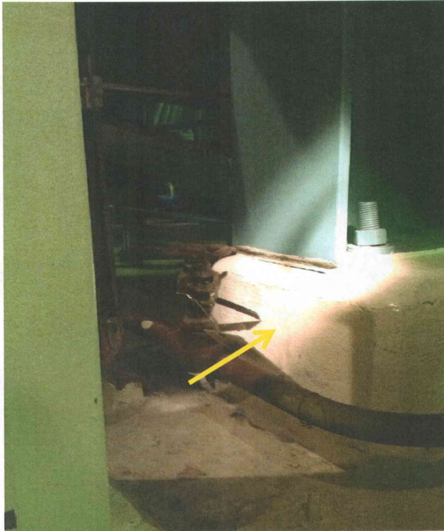
T12 Pedestal with Minor Hairline Crack
