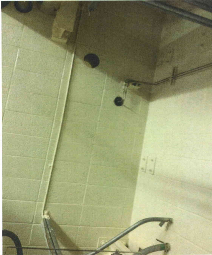
Sf47 adjacent block wall Potential interaction hazard from masonry wall near unit
