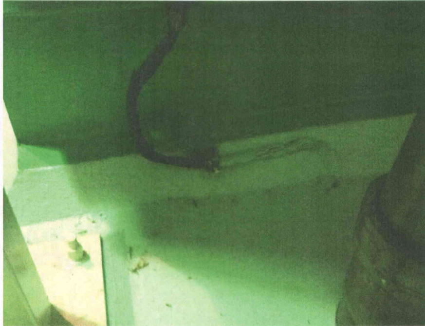
P43-2 anchorage Partial view of anchorage, view is typical of all anchors
