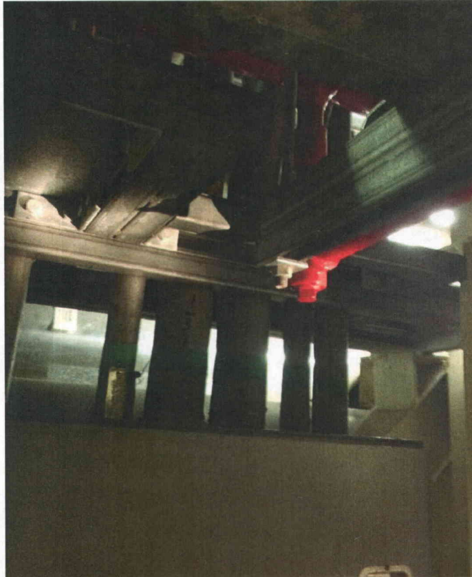
RC3701 Conduits Conduits Going into Cabinet
