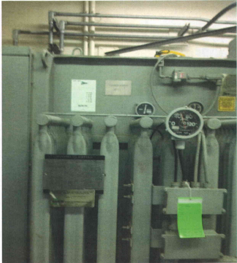
XDF1-2 General General view of component
