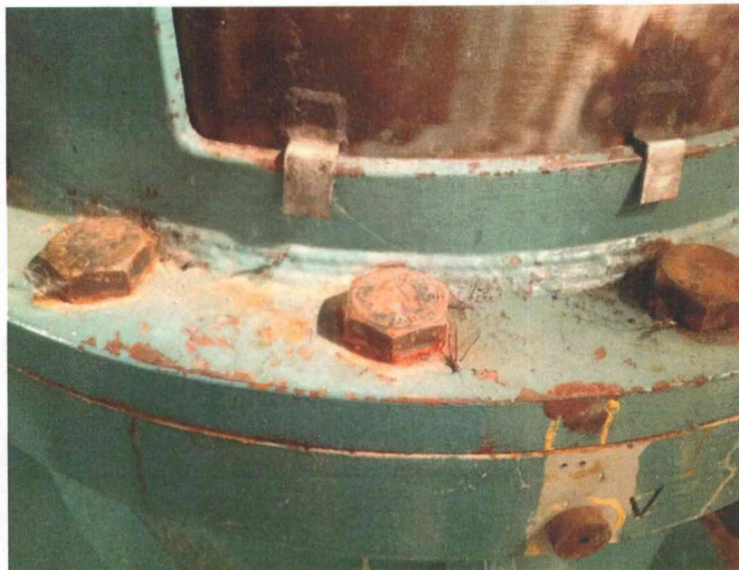
P3-2 corrosion on bolts
