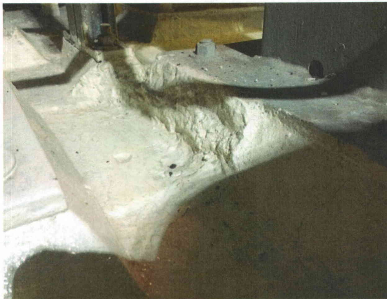
LT1402 Spalled Grout on Anchor Grout around base plate has crumbled away
