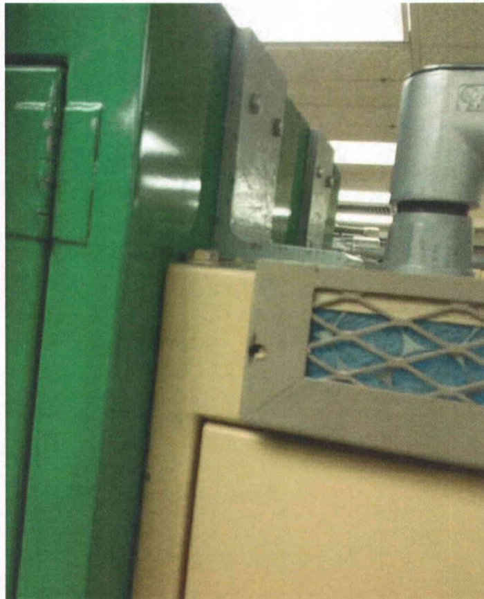
SP9B9-073 bolted at top Cabinet is bolted to adjacent cabinet at the top
