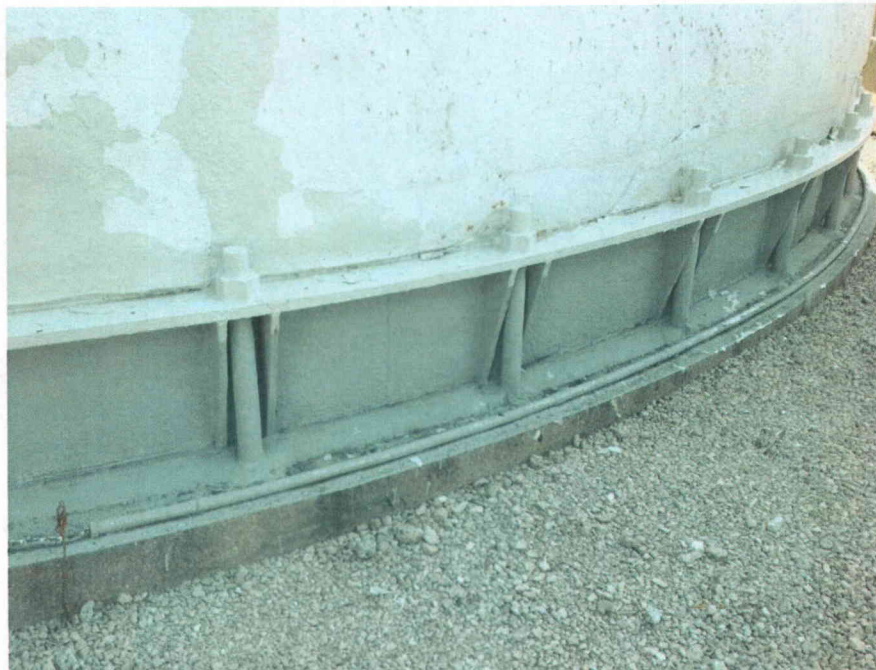
BWST Anchorage Partial view of anchorage, view is typical of all anchors
