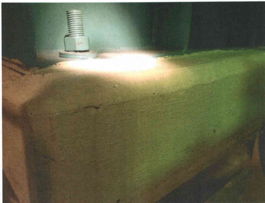
T12 loose bolt front right Anchor bolt coming loose on the front right of component
