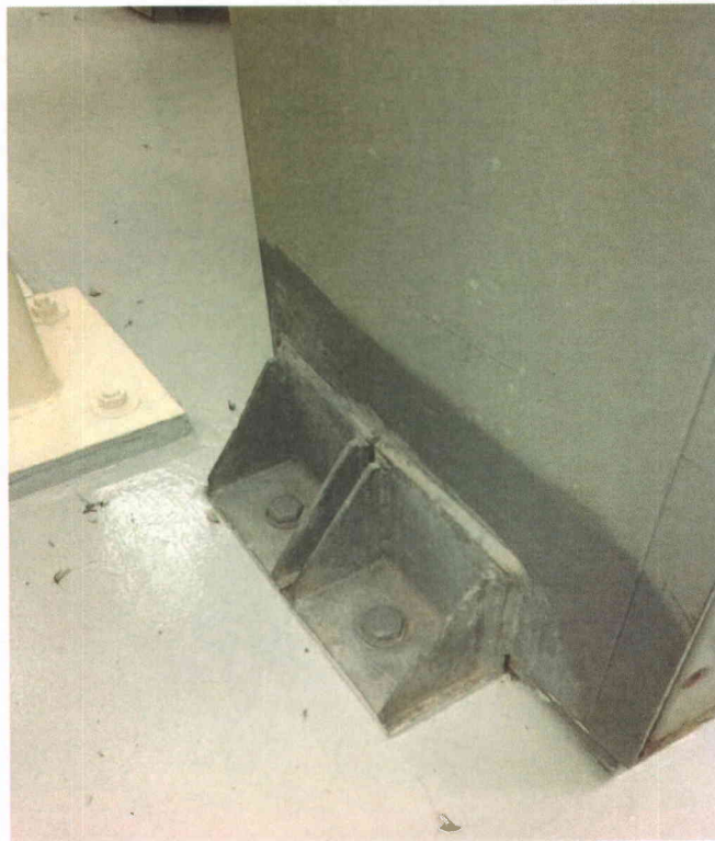
Y2 anchorage one side only Additional anchorage on outside of the unit, on one side only
