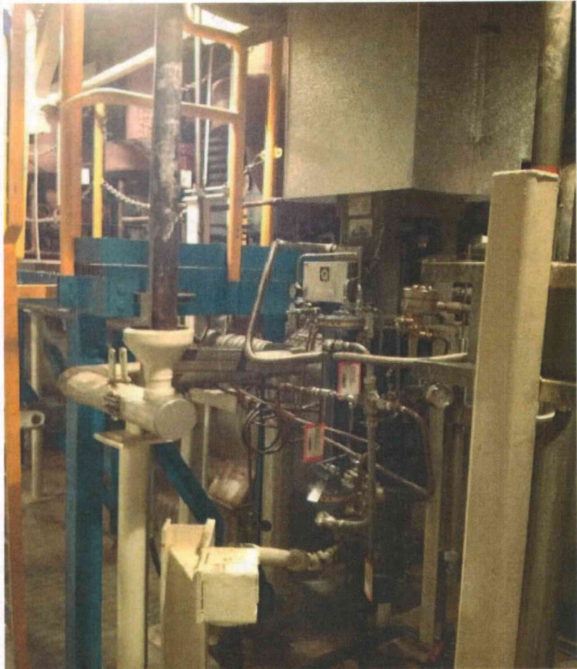
ICS11A General General view of component
