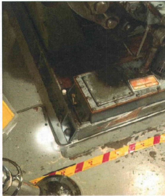
P372B anchorage Partial view of anchorage, view is typical of all anchors
