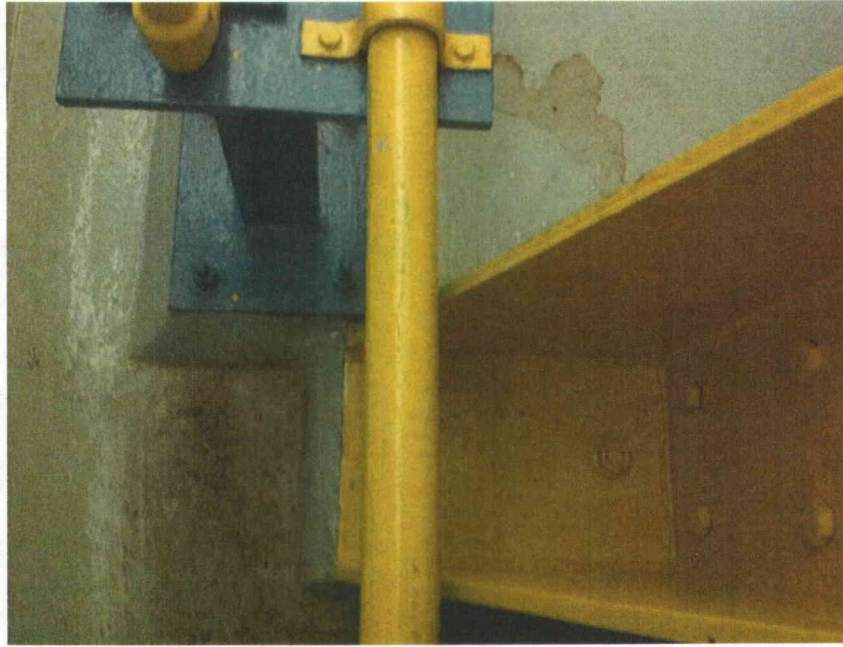
T46-1 anchorage Partial view of anchorage, view is typical of all anchors
