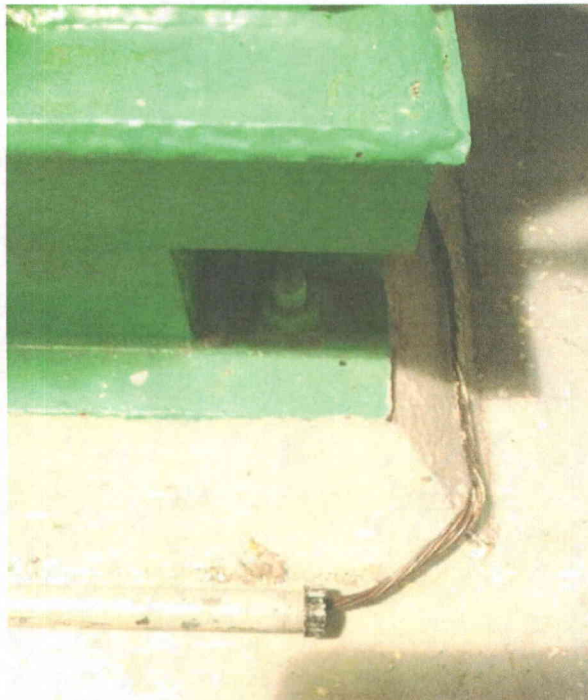
P58-1 anchorage Partial view of anchorage, view is typical of all anchors
