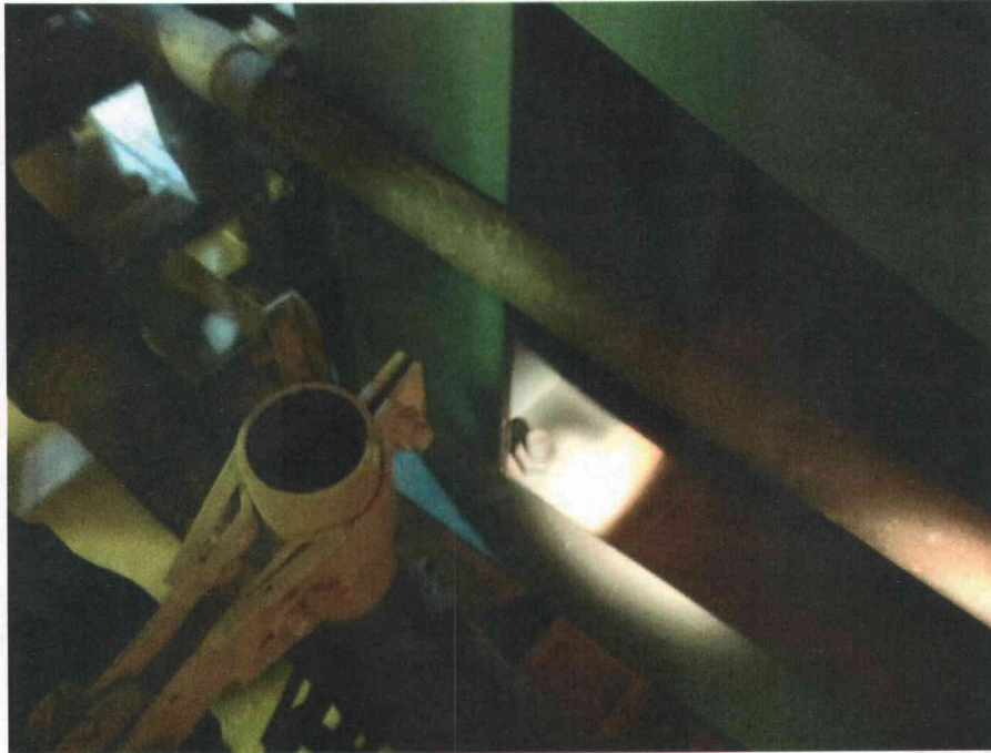
T12 anchorage typical Partial view of anchorage, view is typical of all anchors
