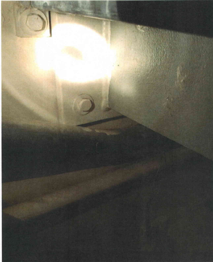
PS3689 anchorage typical Partial view of anchorage, view is typical of all anchors
