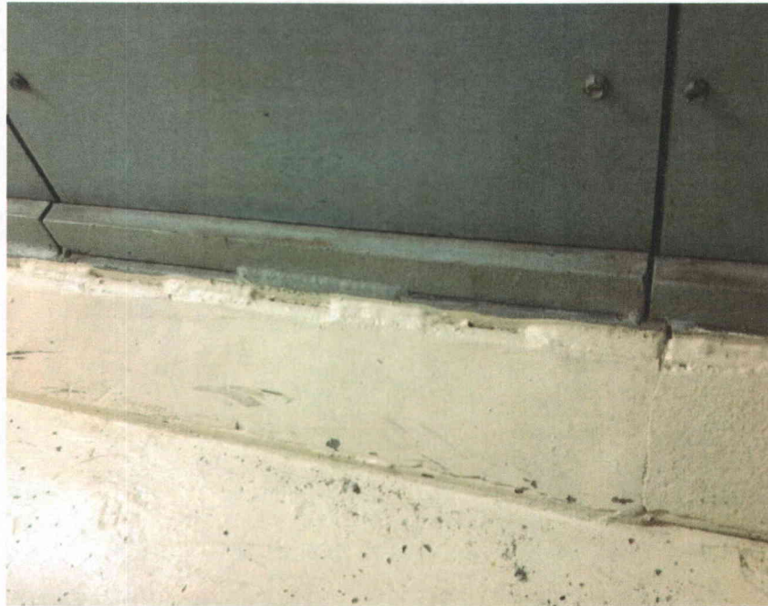
F11A stitch weld Partial view of anchorage, view is typical of all anchors
