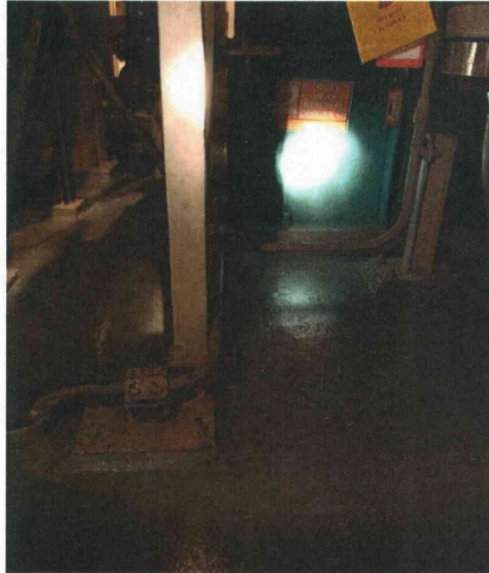
E27-2 anchorage Partial view of anchorage, view is typical of all anchors
