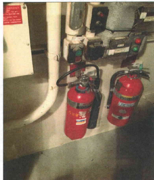
F12D fire ext to right Potential interaction hazard from fire extinguisher in the vicinity of component.
