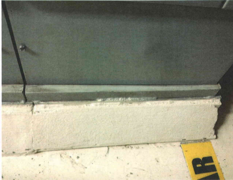
F11A crack in base of grout on corner Separation in base grout. Appears to be aesthetic grout only.
