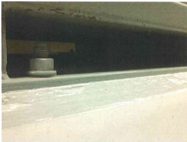
D2P anchor bolts Partial view of anchorage, view is typical of all anchors
