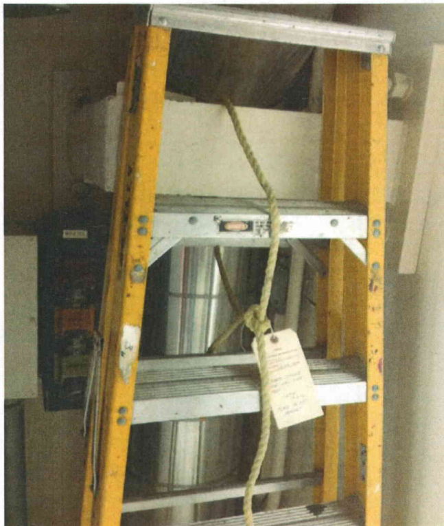
F11A poorly secured ladder in area of MCC Ladder loosely tied off.
