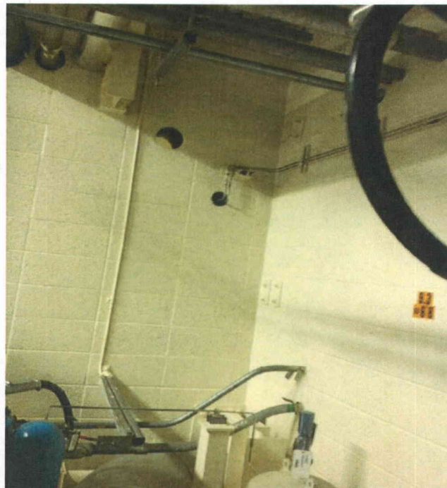
FIS1612 adjacent masonry wall Potential interaction hazard from masonry wall near unit
