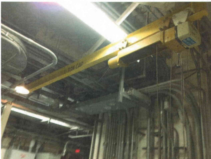
C4606 crane int Sliding crane located in component vicinity.
