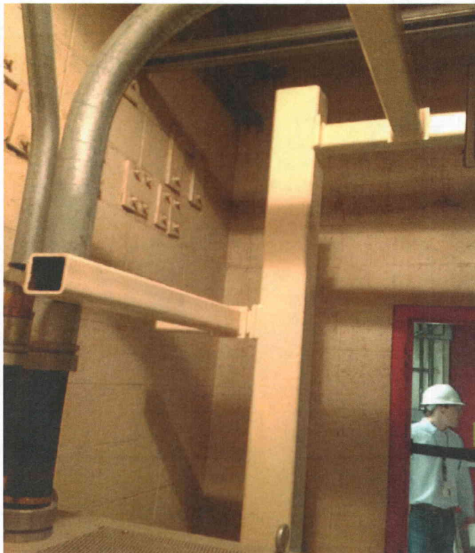
D2N masonry walls Potential interaction hazard from masonry wall near unit
