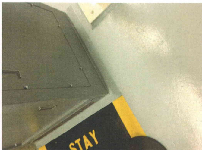
DBC2PN anchorage inaccessible Anchorage is not visible
