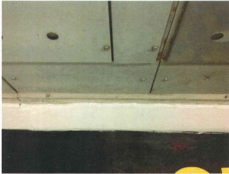
F12A stitch weld Partial view of anchorage, view is typical of all anchors
