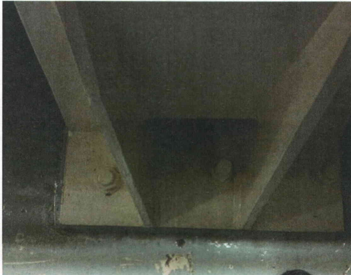
E22-1 anchorage left Partial view of anchorage, view is typical of all anchors
