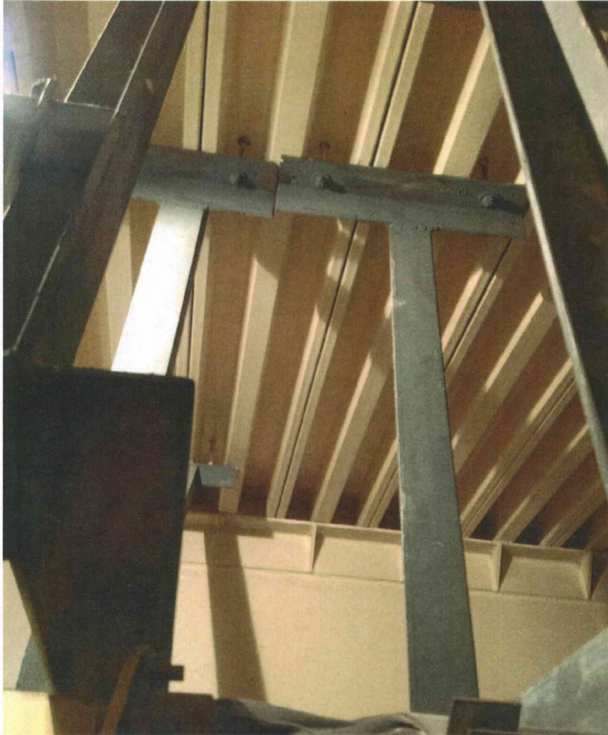
C78-2 anchorage Partial view of anchorage, view is typical of all anchors
