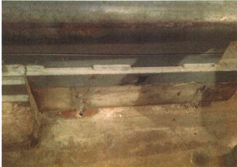
E12C grout missing View of mounting base showing stitch weld detail and grout
