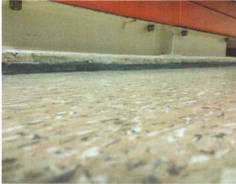
C5792A anchorage Partial view of anchorage, view is typical of all anchors
