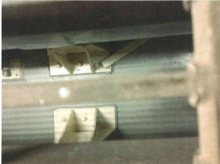
E22-2 anchorage right side Partial view of anchorage, view is typical of all anchors
