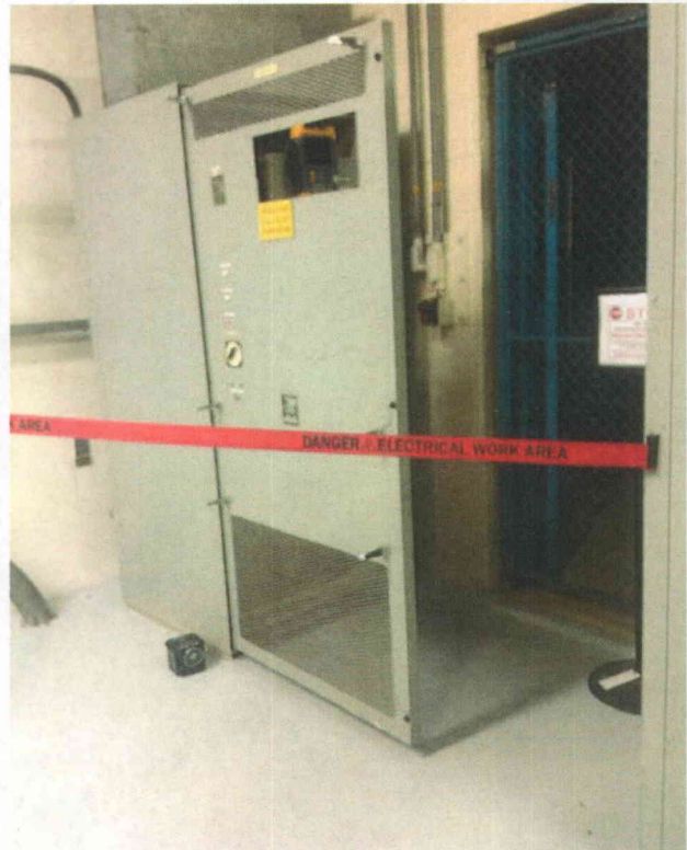
DBC2P masonry walls Potential interaction hazard from masonry wall near unit
