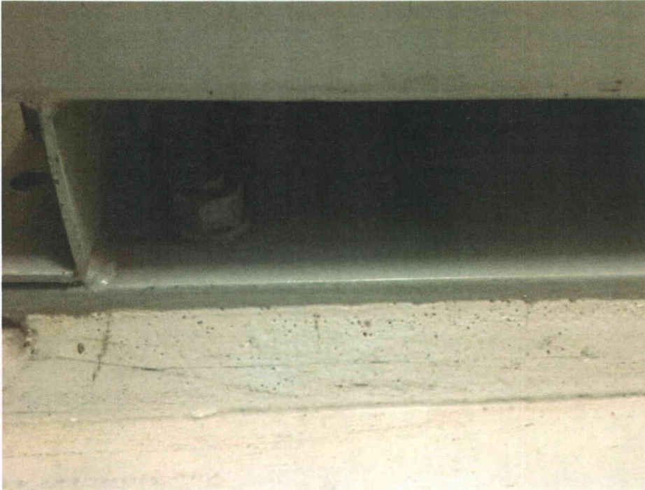
DIN anchorage Partial view of anchorage, view is typical of all anchors
