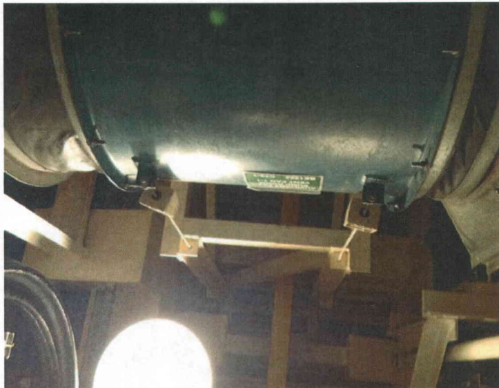
C73-1 plate and anchorage no lateral bracing View of anchorage, no lateral bracing is visible for hanging fan
