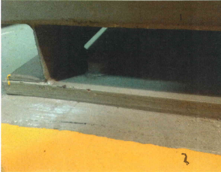
D2N 4 anchor bolts Partial view of anchorage, view is typical of all anchors
