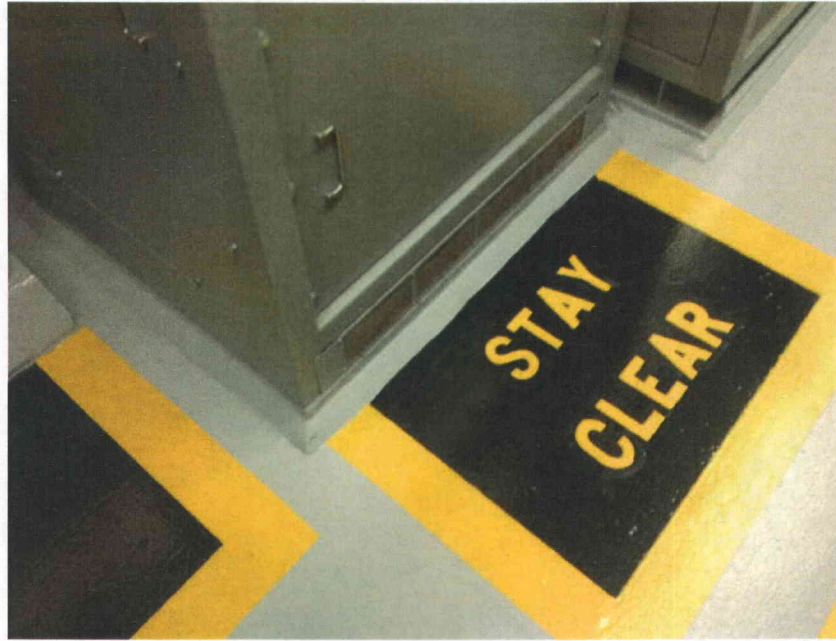
DBC1PN anchorage inaccessible Anchorage is not visible
