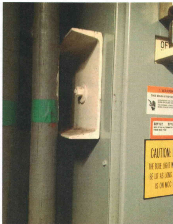
EF12C brace left View of channel section used to restrain front-to-back motion. Same detail at opposite side.
