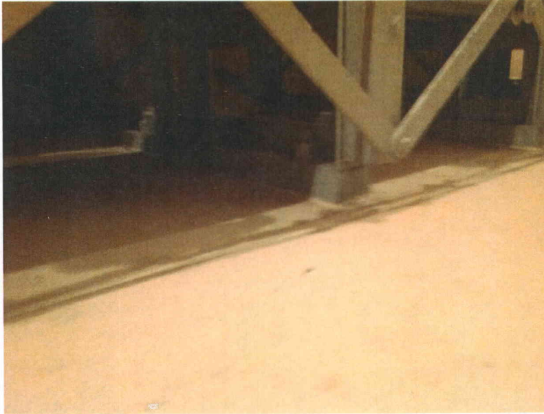
2N Anchorage Partial view of anchorage, view is typical of all anchors
