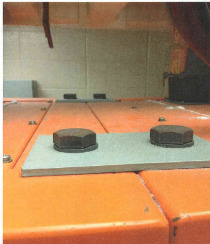
C5792A bolted to cabinet at right Adjacent cabinets are bolted together
