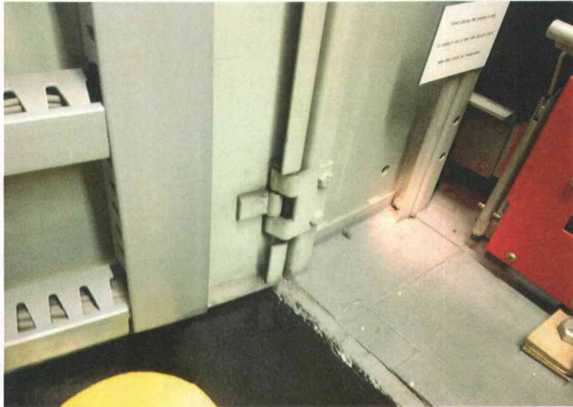
D1 Inside Cabinet View of floor detail inside D1 cabinet
