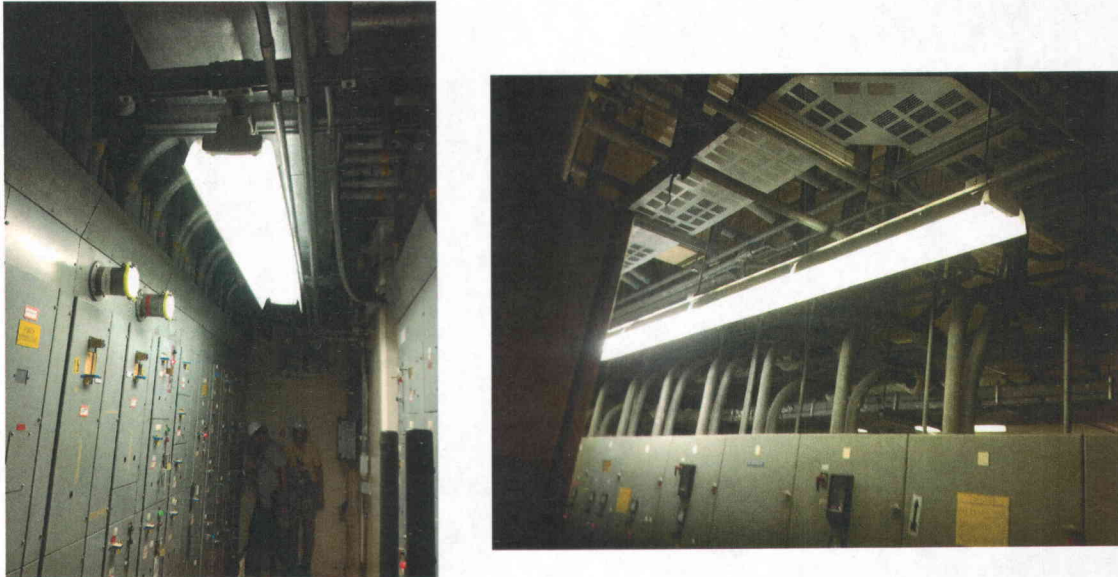
Figure 6-1: Unguarded Fluorescent Light Tubes
