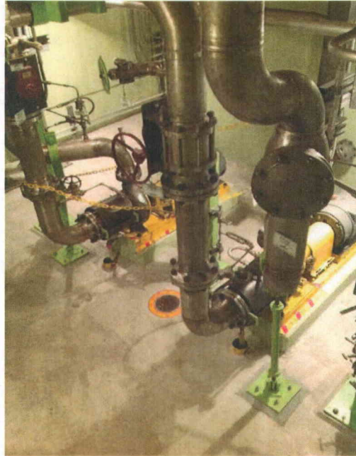
File Name: 1-65-3-3-29.jpeg Description: View of pipe lines attached to pumps in the area
