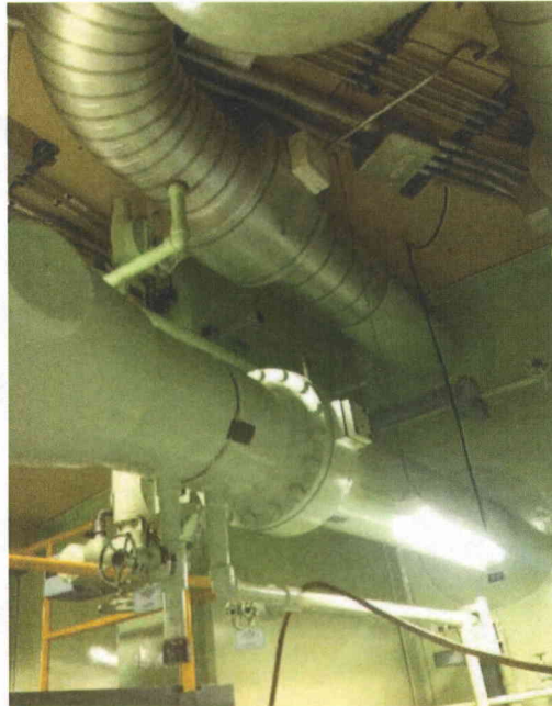
File Name: 1-67-2-3-12.jpeg Description: View of large diameter pipes
