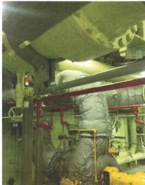
File Name: 1-71-5-3-03.jpeg Description: View of fire lines in the area
