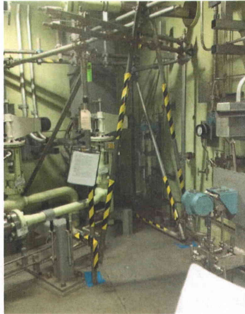
File Name: 1-60-3-3-25.jpeg Description: Scaffold identified in the area
