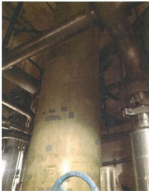
File Name: 2-63-3-2-18.jpeg Description: General view of Heat Exchanger 2RHS-E21B
