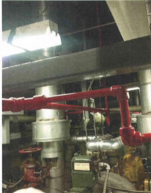
File Name: 1-59-5-3-23.jpeg Description: General view of fire line located in the area.
