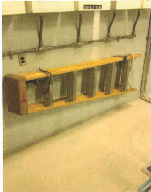
File Name: EDG2-1_Up(5).jpg Description: Properly restrained ladder identified in the area
