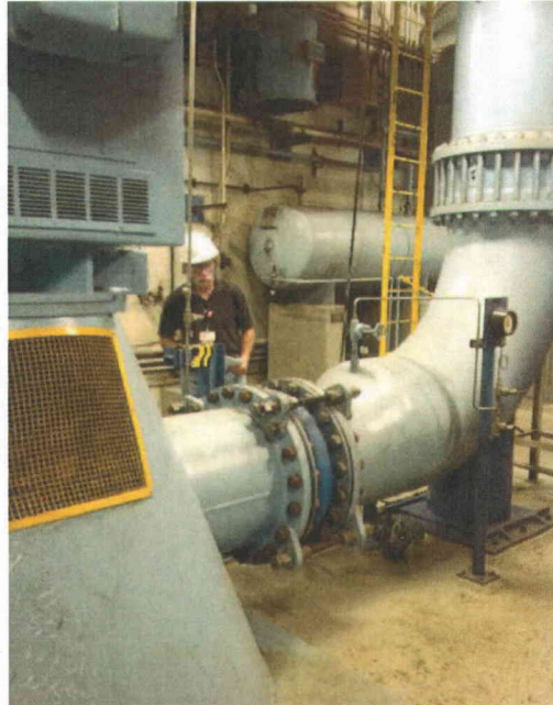
File Name: INTK_CUB_D(1).jpg Description: View of expansion joint located on pipe attached to vertical Pump 2SWS-P21A.
