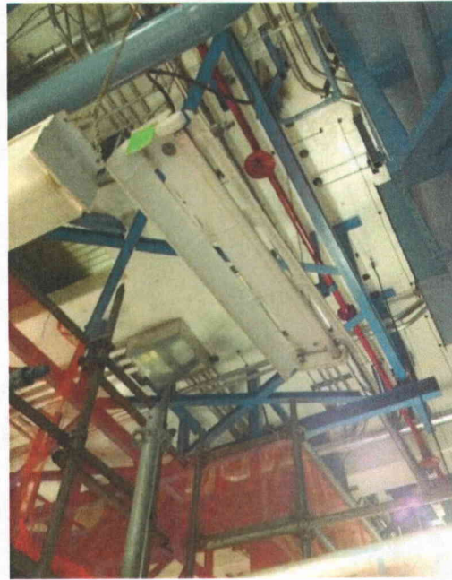
File Name: EDG2-1(9).jpg Description: View of lighting fixture with missing fluorescent tube.
