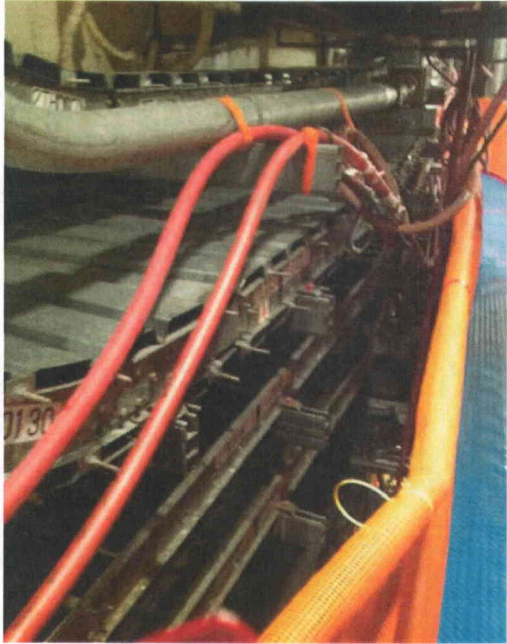
File Name: 1-65-2-3-19.jpeg Description: View of cable trays in the area.
