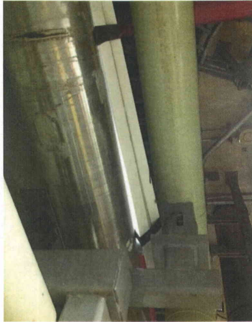
File Name: 1-65-5-3-23.jpeg Description: Hanging light bearing on top of pipe.
