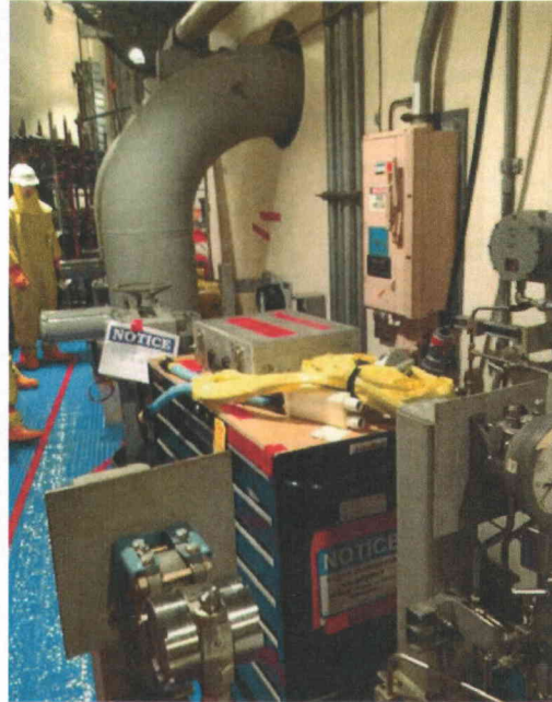
File Name: 1-59-4-3-19.jpeg Description: Temporary outage related maintenance equipment
