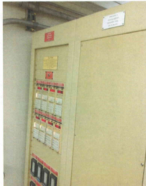
File Name: Control_Rm(4).jpg Description: View of cabinet in the area
