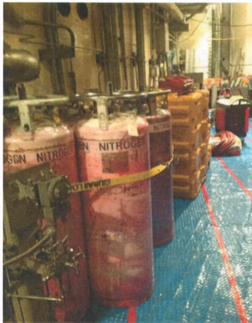
File Name: 1-60-5-3-19.jpeg Description: View of nitrogen bottles and storage boxes properly secured in the area
