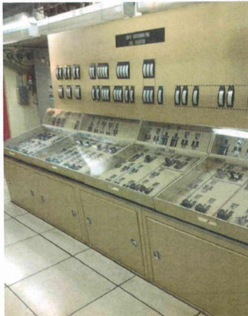
File Name: 1-60-3-3-06.jpeg Description: View of control panel
