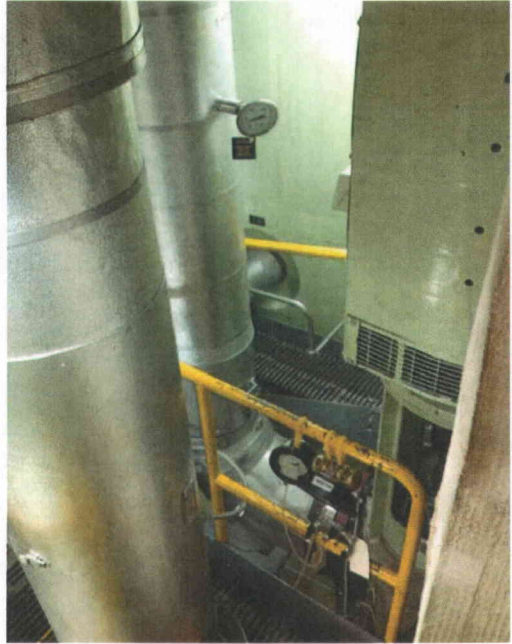
File Name: 1-67-8-3-23.jpeg Description: Insulated line attached to 2RSS-P21A.
