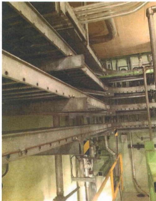
File Name: 1-60-2-3-29.jpeg Description: View of cable trays in the area
