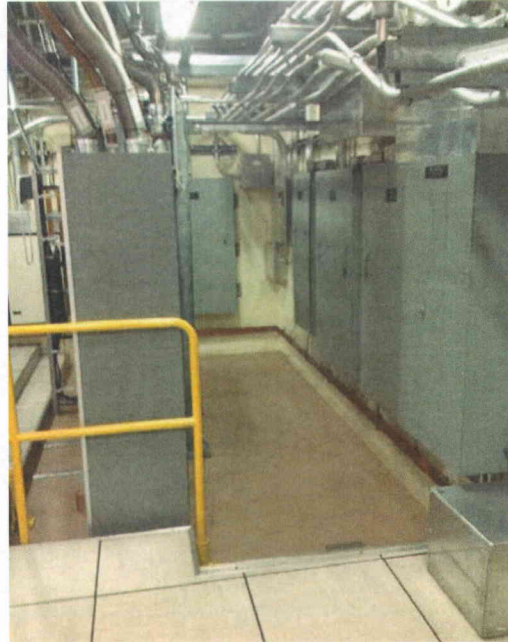
File Name: 1-65-3-3-06.jpeg Description: View of cabinet arrangement in the area
