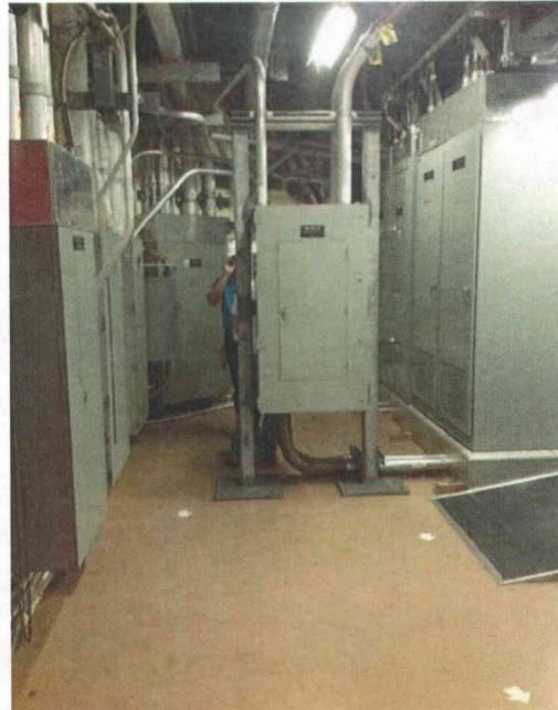
File Name: 1-59-4-3-06.jpeg Description: South-west area with wall mounted panels
