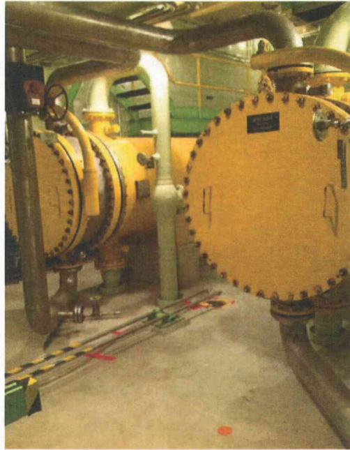
File Name: 1-59-2-3-29.jpeg Description: General view of Heat Exchangers
