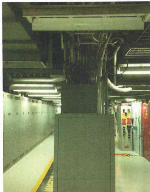
File Name: SWGR AE(2).jpg Description: General view of lighting fixtures and top cabinet conduits
