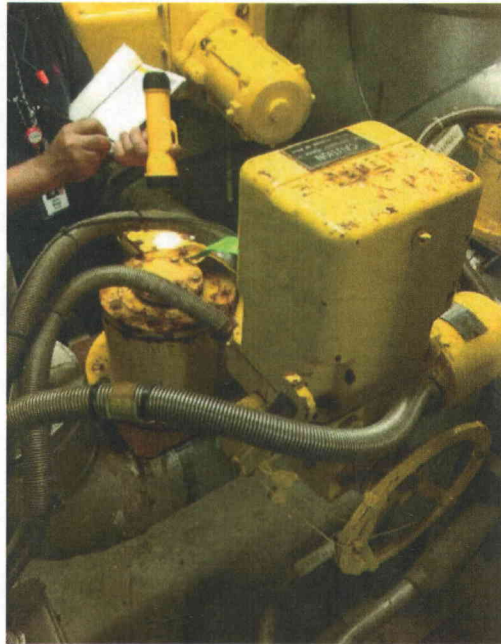
File Name: VLV_PT_A(3).jpg Description: Surface rust identified on several MOVs in the area.
