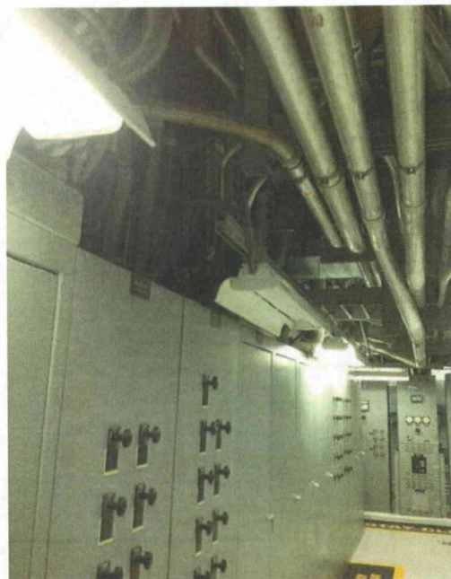
File Name: SWGR AE(6).jpg Description: View of ceiling conduits and lighting fixtures
