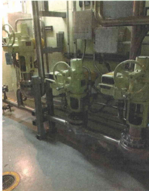
File Name: 1-59-5-3-01.jpeg Description: General view of valves in the area
