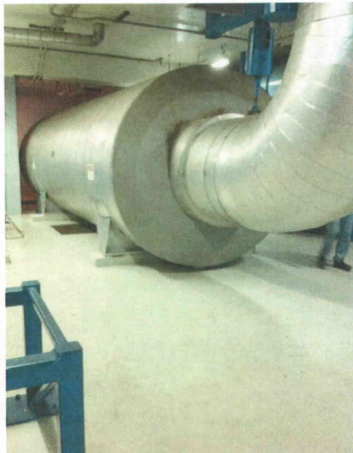
File Name: EDG2-1_Up(2).jpg Description: General view of DG exhaust muffler
