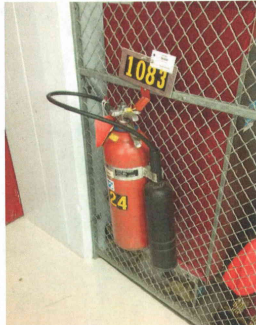
File Name: SWGR AE(3).jpg Description: Fire extinguisher located in the area
