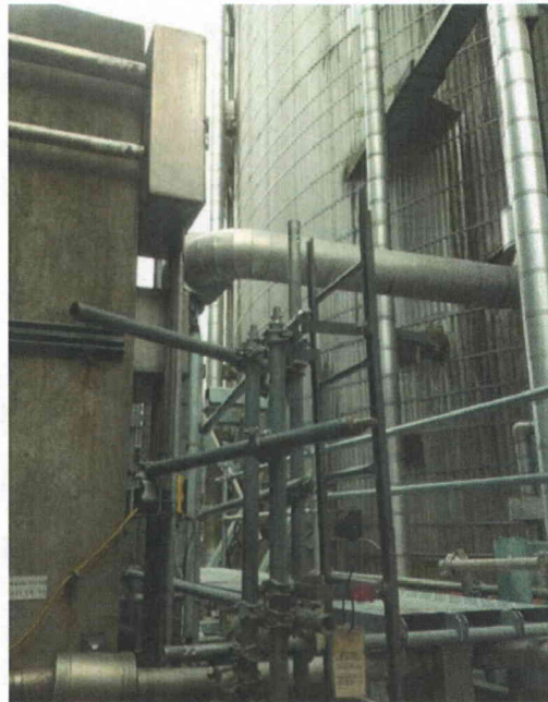
File Name: 1-60-4-3-29.jpeg Description: Scaffold located in the area.
