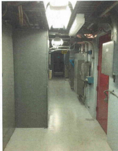
File Name: SWGR_DF(2).jpg Description: General view of cabinets and lighting fixtures
