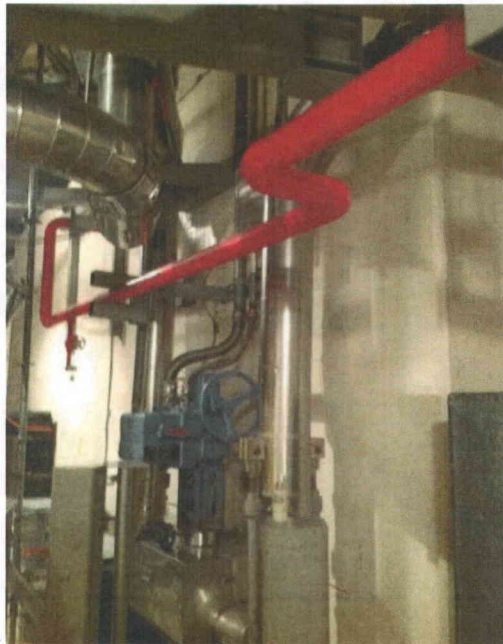
File Name: 1-60-4-3-17.jpeg Description: Fire line located above 2CHS-MOV310
