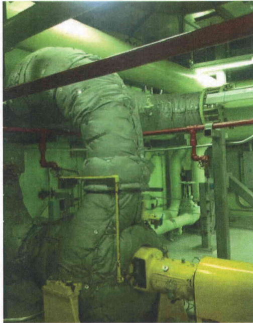
File Name: 1-67-5-3-03.jpeg Description: General view of insulated pipe lines.
