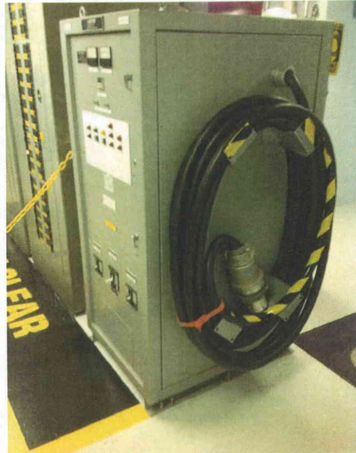
File Name: SWGR_DF(7).jpg Description: View of 1.5" diameter loops of cable mounted on the side of BAT-CHG2-9
