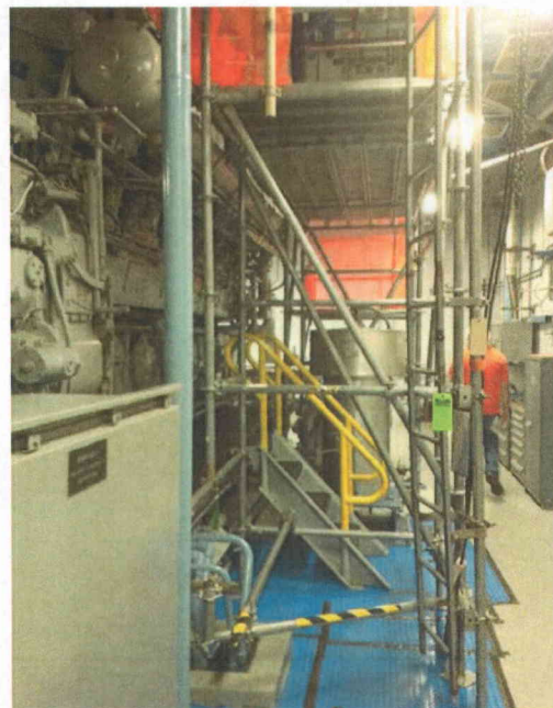
File Name: EDG2-1(6).jpg Description: View of scaffold located next to Diesel Generator
