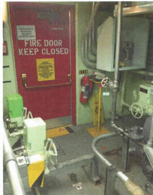
File Name: 1-60-5-3-16.jpeg Description: Fire extinguisher and floor mounted supports for room pipe lines.
