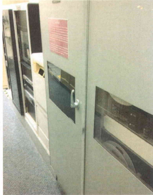
File Name: Control_Rm(1).jpg Description: View of panel PNL-2FAL-REC was not positively latched.
