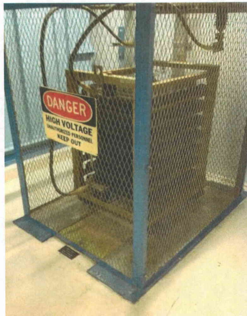
File Name: EDG2-1_Up(6).jpg Description: View of DG ground resistor
