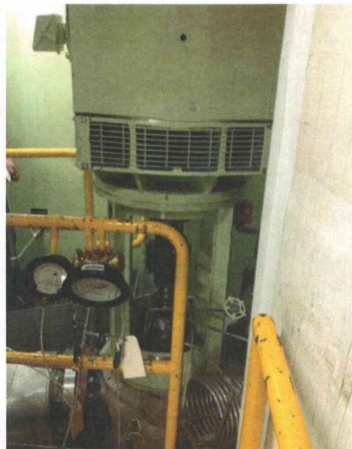
File Name: 1-60-8-3-23.jpeg Description: View of Recirc Spray Pump 2RSS-P21A.
