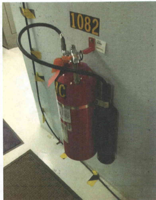
File Name: SWGR_DF(6).jpg Description: Fire extinguisher located in the area
