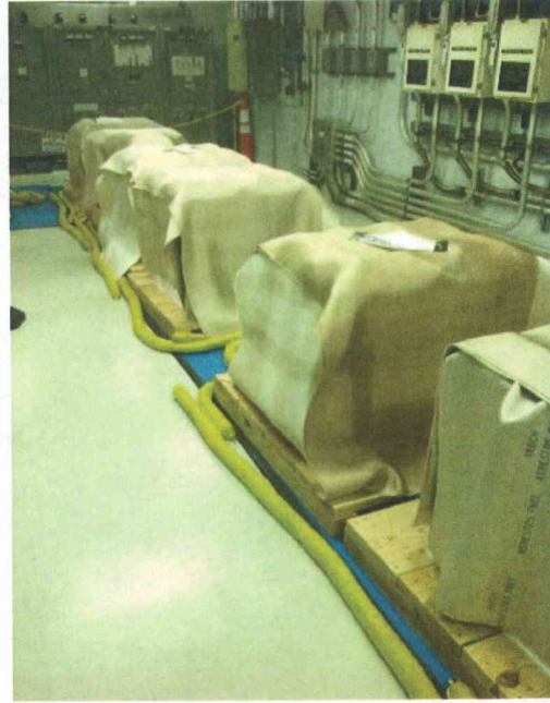
File Name: SWGR_DF(1).jpg Description: General view of electrical equipment in the area
