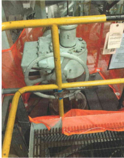
File Name: 1-65-2-3-27.jpeg Description: Scaffold identified in the area
