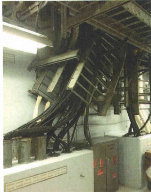
File Name: SWGR_DF(3).jpg Description: View of cable trays above electrical cabinets
