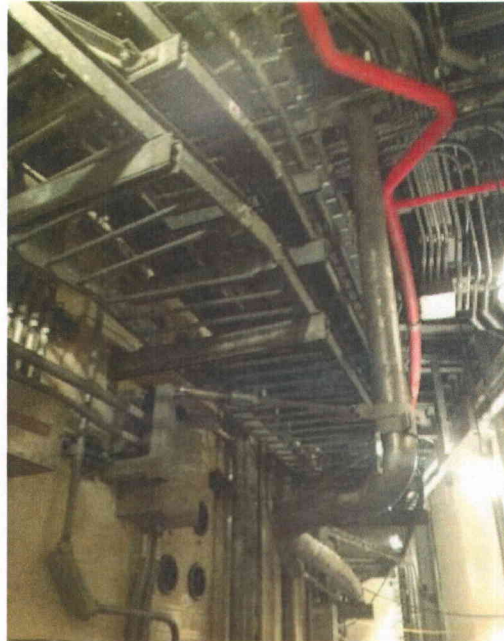
File Name: 1-59-5-3-19.jpeg Description: General view of cable trays and fire line in the area
