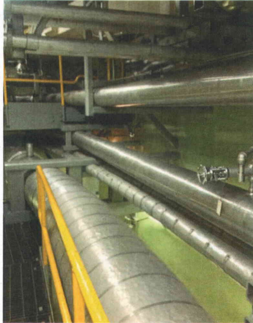
File Name: 1-59-7-3-23.jpeg Description: View of supports for piping in the area
