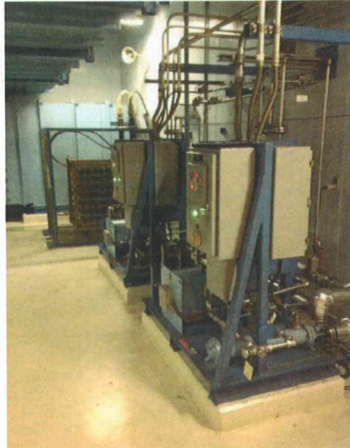
File Name: EDG2-1_Up(1).jpg Description: View of electrical equipment properly braced in the area
