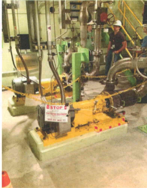
File Name: 1-59-3-3-29.jpeg Description: Overall view of pumps in the area
