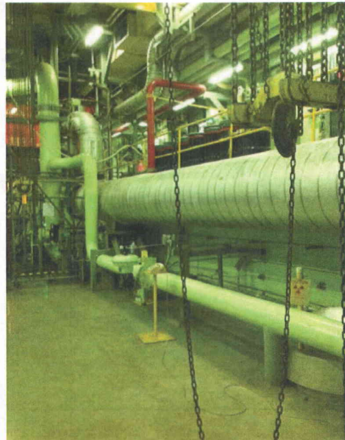
File Name: 1-66-4-3-01.jpeg Description: General view of Heat Exchanger
