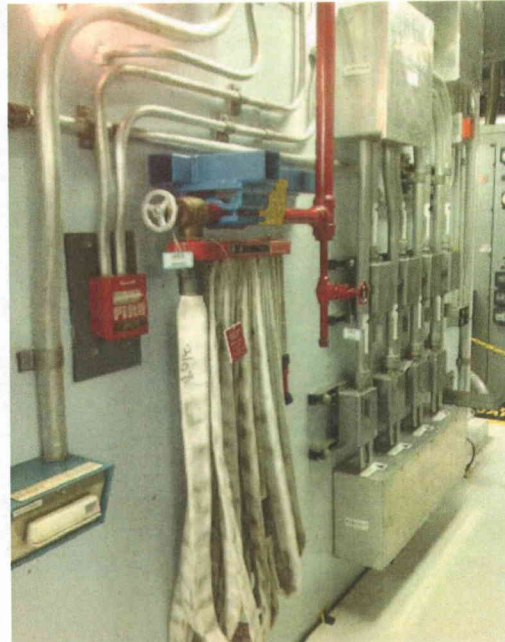
File Name: SWGR_DF(5).jpg Description: Fire hose located in the area
