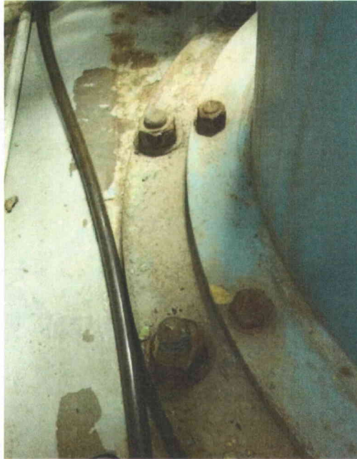
File Name: INTK_CUB_C(5).jpg Description: Surface rust identified on bolts for Pump 2SWS-P21B.
