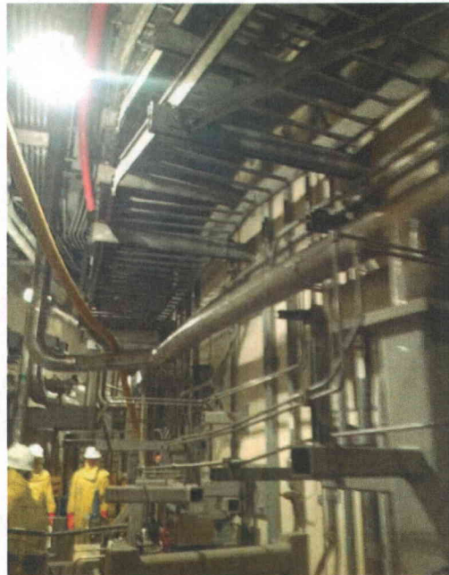
File Name: 1-66-5-3-19.jpeg Description: View of wall mounted supports for piping and cable trays.
