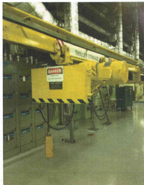
File Name: 1-66-5-3-03.jpeg Description: Trolley identified in the area to be securely restrained
