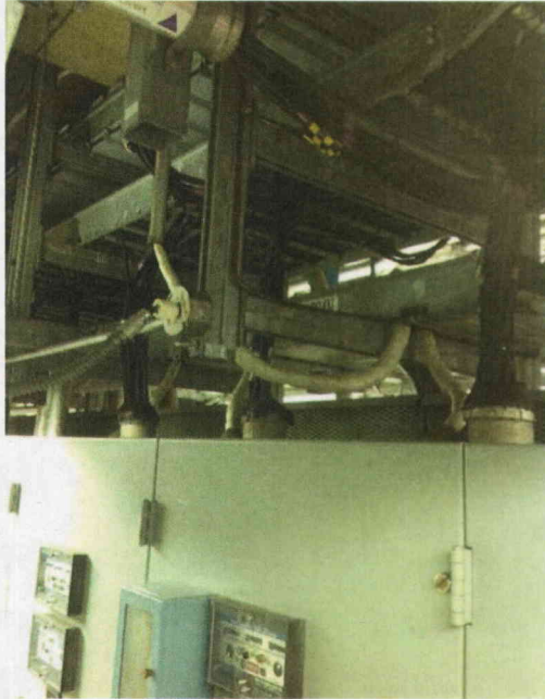
File Name: 4KVS-2-DF(3).jpg Description: View of Flexible Top Conduit
