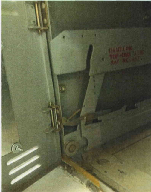
File Name: 2-62-9-2-26.jpeg Description: Adjacent Cabinets Bolted Together
