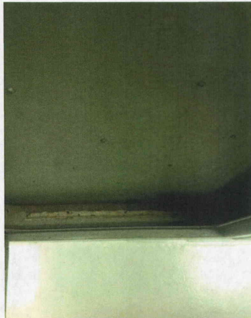
File Name: 2-62-14-2-26.jpeg Description: View of Internal Welding in Front of Cabinet
