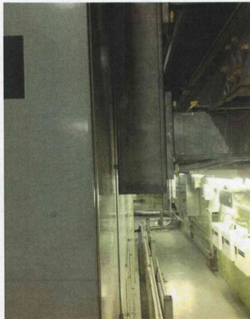
File Name: 2-94-1-2-13.jpeg Description: Space Between MCC and Cable Tray Support
