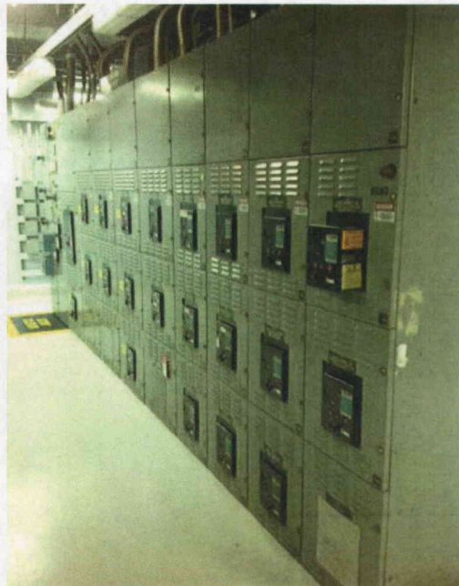
File Name: 480VUS-2-8(2).jpg Description: General View of Component
