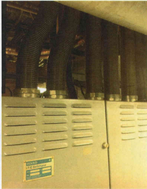
File Name: 480VUS-2-9(3).jpg Description: View of Flexible Top Conduit
