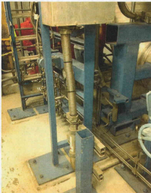
File Name: 2SWS-PT-117A(6).jpg Description: General View of Rack
