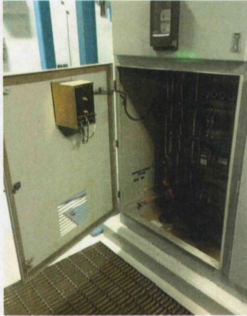
File Name: 2-62-8-2-08.jpeg Description: View of Open Cubicle
