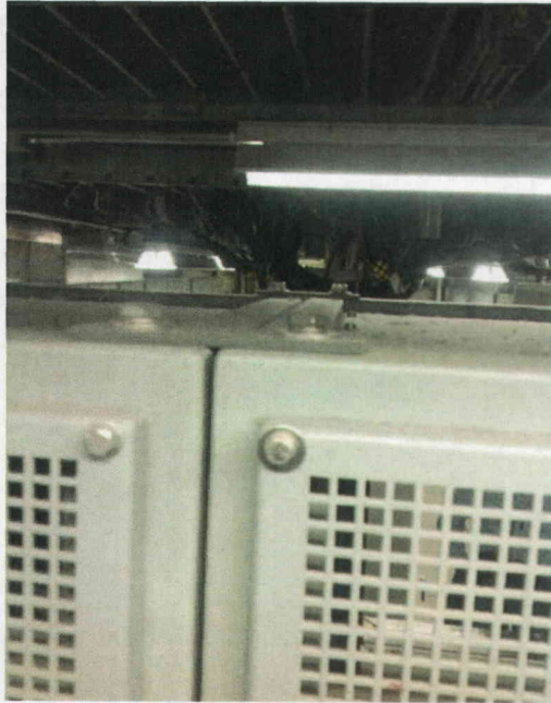
File Name: 2-95-4-2-06.jpeg Description: Adjacent Cabinets are Bolted Together
