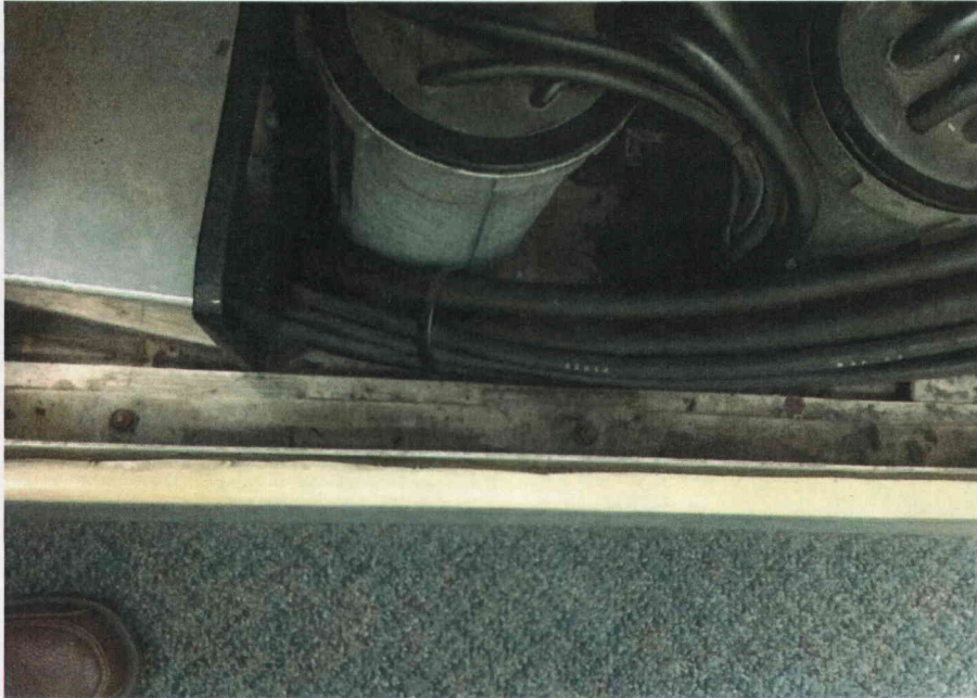
File Name: 2HVR-TI228(1).jpg Description: View of Cabinet Anchorage
