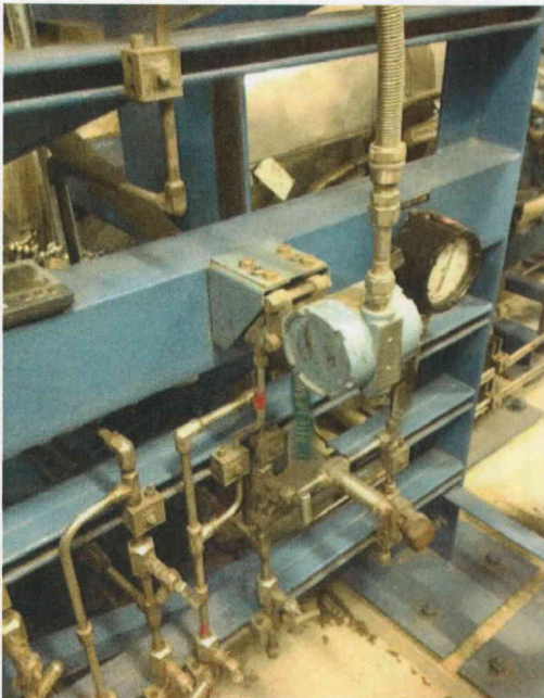
File Name: 2SWS-PT-117A(2).jpg Description: General View of Component on Rack
