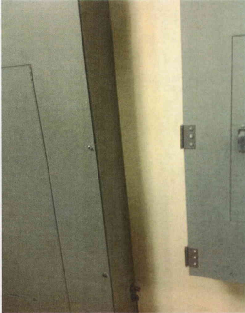
File Name: 2-63-2-2-06.jpeg Description: Anchorage Inaccessible
