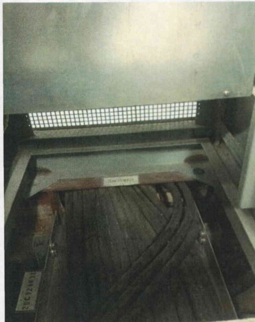
File Name: 2-62-3-2-06.jpeg Description: View of Interior at Cabinet Base
