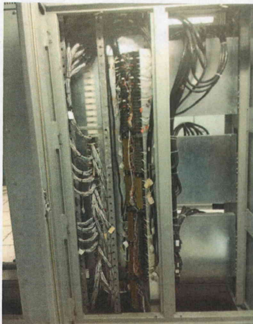
File Name: 2-94-4-2-06.jpeg Description: View of Opened Cabinet
