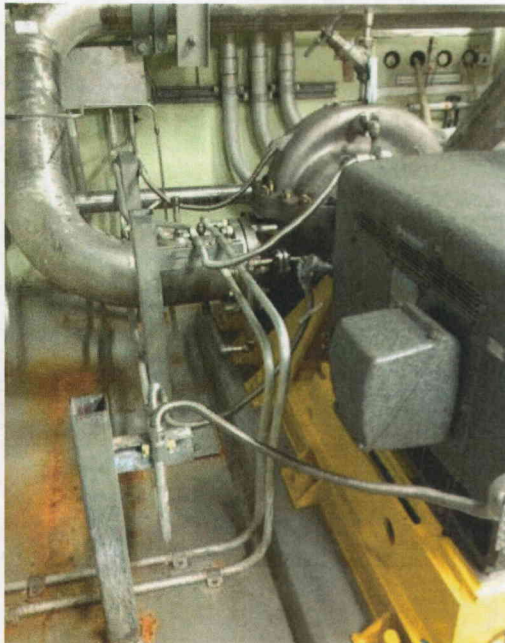
File Name: 2-64-5-2-23.jpeg Description: View of Attached Lines
