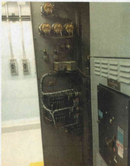
File Name: 2-94-9-2-26.jpeg Description: View of Components Mounted on Door
