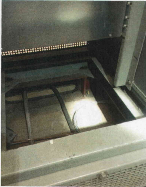
File Name: 2-73-4-2-06.jpeg Description: View of Interior at Cabinet Base
