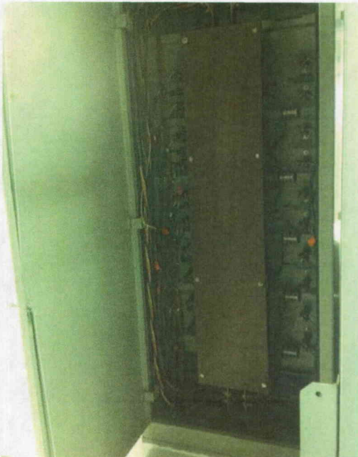
File Name: 2-63-10-2-26.jpeg Description: View of Opened Cabinet
