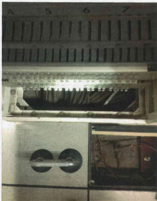
File Name: 2-64-7-2-06.jpeg Description: View of Interior at Cabinet Base
