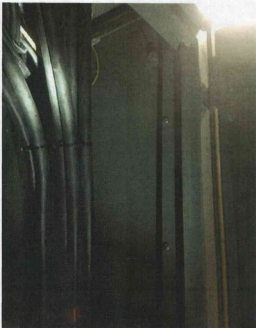
File Name: 2-62-5-2-06.jpeg Description: Adjacent Cabinets are Bolted Together
