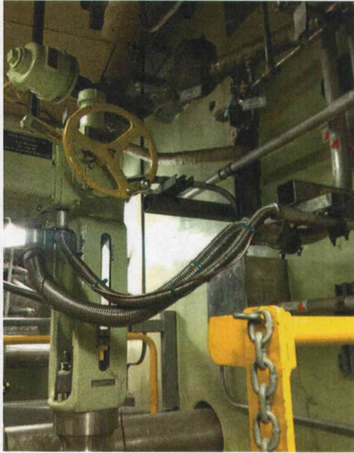
File Name: 2-63-8-2-23.jpeg Description: View of Attached Lines
