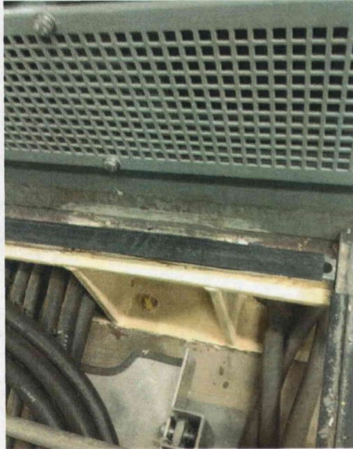
File Name: 2-95-3-2-06.jpeg Description: View of Anchor Weld and Wide Flange Anchor Bolt
