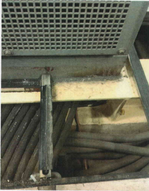
File Name: 2-97-4-2-06.jpeg Description: View of Base Weld
