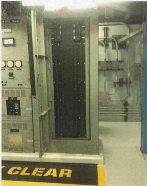
File Name: 2-64-17-2-26.jpeg Description: View of Opened Cabinet
