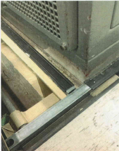
File Name: 2-95-5-2-06.jpeg Description: View of Base Weld
