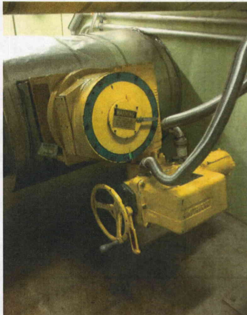
File Name: 2SWS-MOV106A(2).jpg Description: General View of Component
