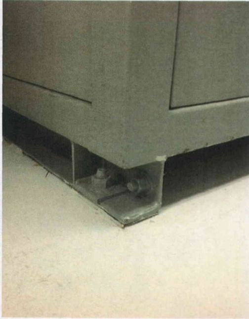
File Name: BAT-CHG2-1(1).jpg Description: View of Anchor Bolts in Rear of Component
