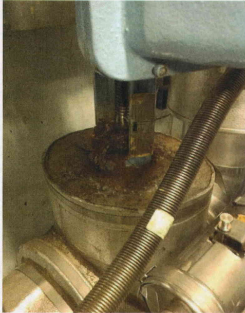
File Name: 2SWS-MOV113A(3).jpg Description: View of Corroded Packer Nuts
