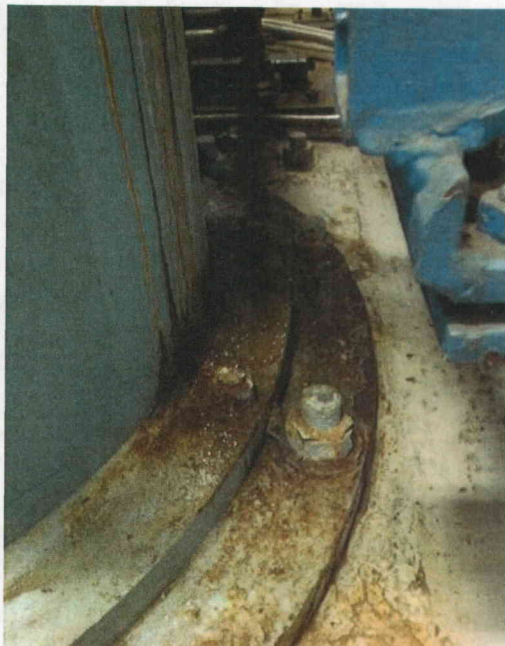
File Name: 2SWS-P21A(4).jpg Description: View of Corroded Anchorage
