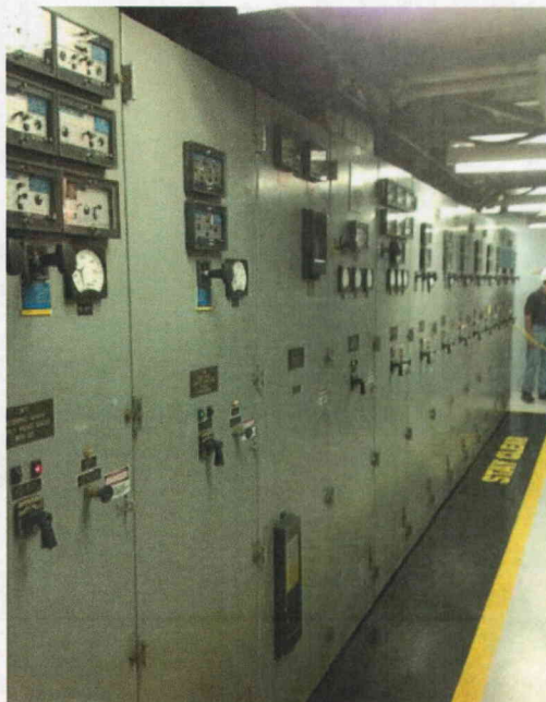
File Name: 4KVS-2-DF(2).jpg Description: General View of Component
