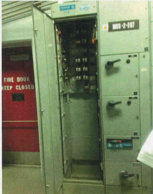
File Name: 2-61-6-2-08.jpeg Description: View of Open Cubicle
