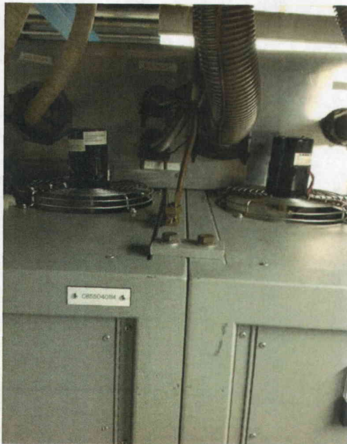
File Name: UPS-VITBS2-1-REG(1).jpg Description: View of Top Bolting of Cabinets
