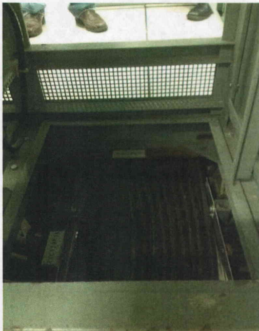
File Name: 2-64-4-2-06.jpeg Description: View of Interior at Cabinet Base
