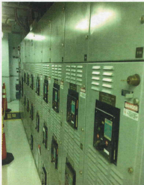
File Name: 480VUS-2-9(2).jpg Description: General View of Component
