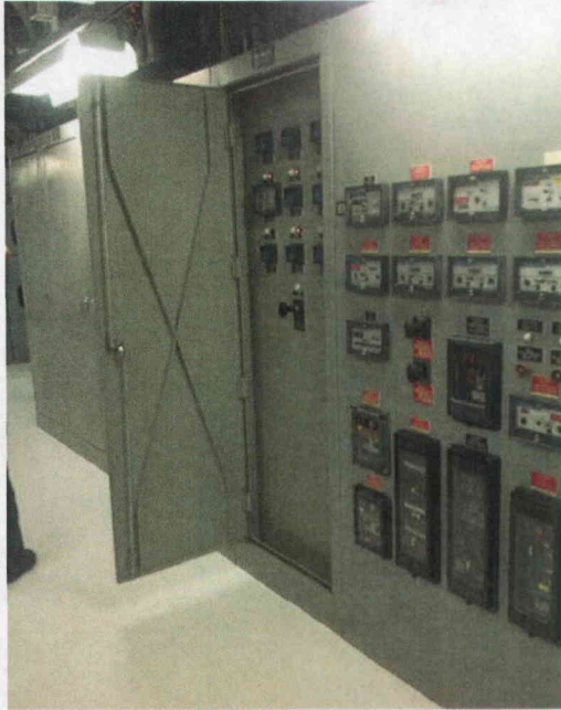
File Name: 2-61-14-2-26.jpeg Description: View of Opened Cabinet
