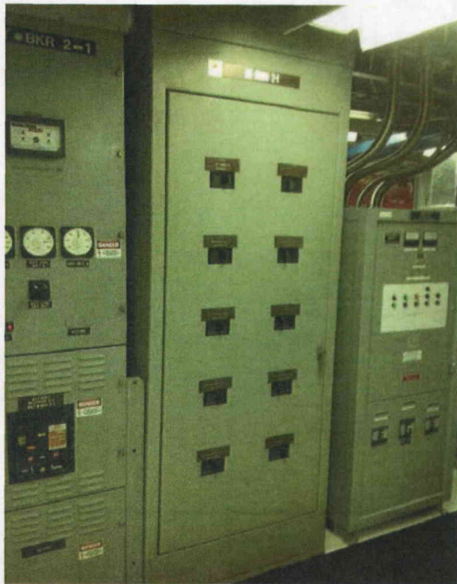
File Name: DC-SWBD2-1(2).jpg Description: General View of Component
