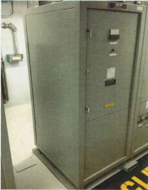
File Name: UPS-VITBS2-1-REG(3).jpg Description: General View of Component
