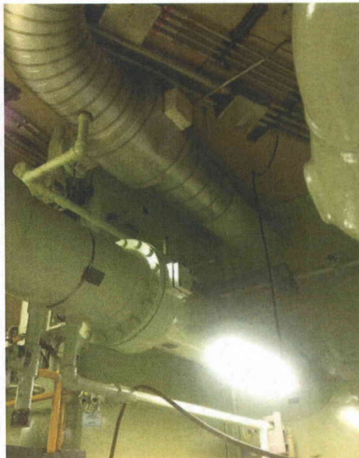
File Name: 2-94-1-2-12.jpeg Description: View of Penetration Support and Branch Line with Adequate Flexibility
