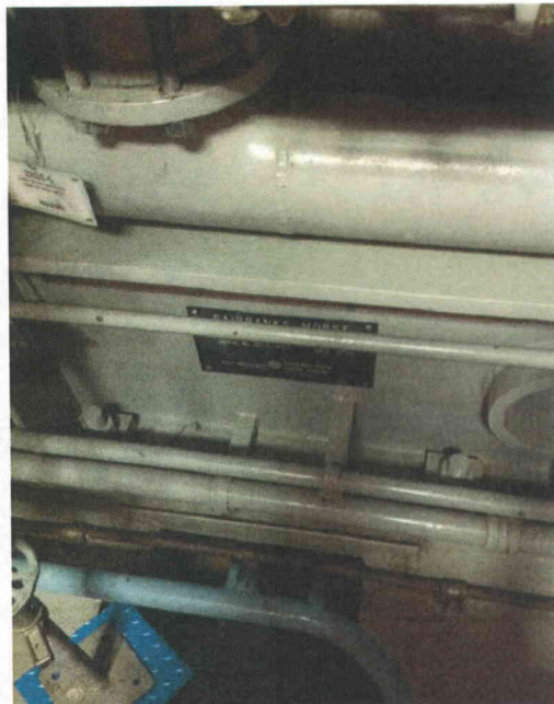
File Name: 2EGS-EG2-1(4).jpg Description: View of Typical Anchor Bolts
