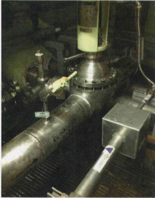
File Name: 2-63-7-2-23.jpeg Description: View of Main Line
