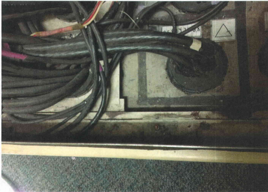
File Name: 2HVR-TI228-1(3).jpg Description: View of Cabinet Anchorage
