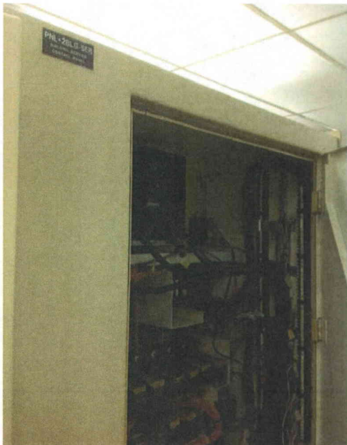
File Name: 2HVR-TI228(4).jpg Description: General View of Inside Cabinet
