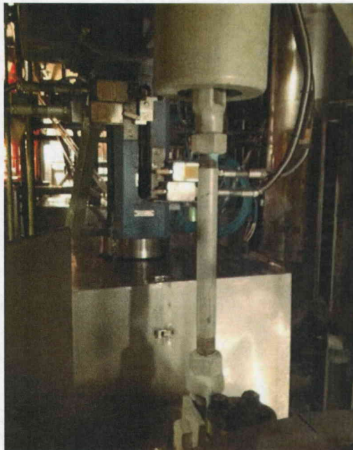
File Name: 2-62-2-2-19.jpeg Description: View of Insulated Main Line
