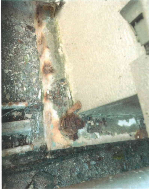
File Name: 2-73-10-2-29.jpeg Description: Corrosion Observed on Anchorage
