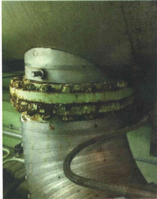
File Name: 2-98-4-2-01.jpeg Description: View of Corrosion on Flange
