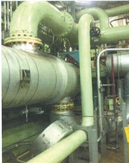
File Name: 2-95-4-2-01.jpeg Description: View of Attached Piping
