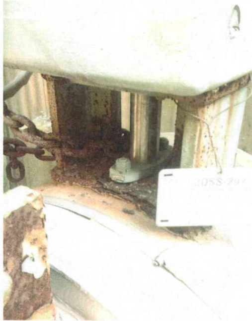
File Name: 2-63-9-2-29.jpeg Description: Corrosion at Valve Base
