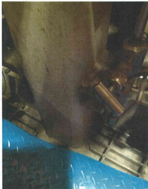
File Name: 2-64-7-2-19.jpeg Description: View of Base Weld
