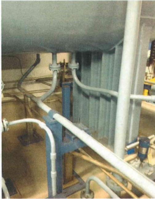
File Name: 2EGF-TK22A(5).jpg Description: View of Attached Lines
