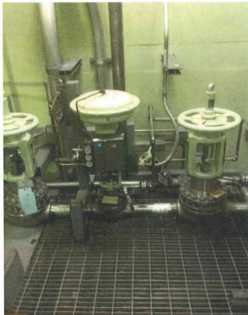
File Name: 2-62-3-2-02.jpeg Description: General View of Component (Center Valve)
