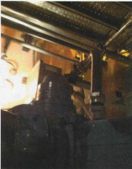
File Name: 2-62-5-2-19.jpeg Description: View of Attached Lines
