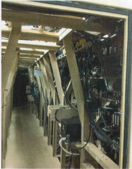
File Name: 2RSS-TI150A(5).jpg Description: General View of Inside Cabinet
