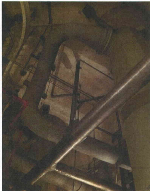
File Name: 2-64-3-2-18.jpeg Description: View of Attached Piping
