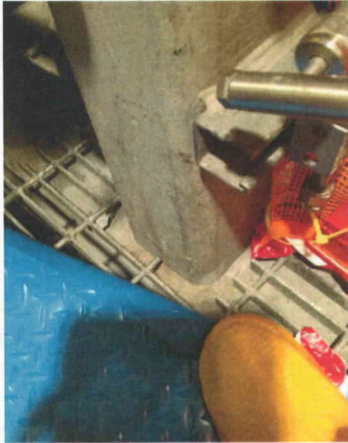
File Name: 2-64-8-2-19.jpeg Description: View of Base Weld
