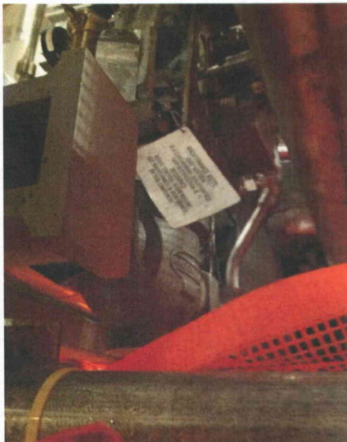
File Name: 2-63-10-2-19.jpeg Description: View of Main Line
