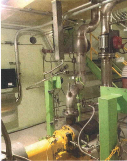
File Name: 2-73-7-2-29.jpeg Description: View of Attached Lines
