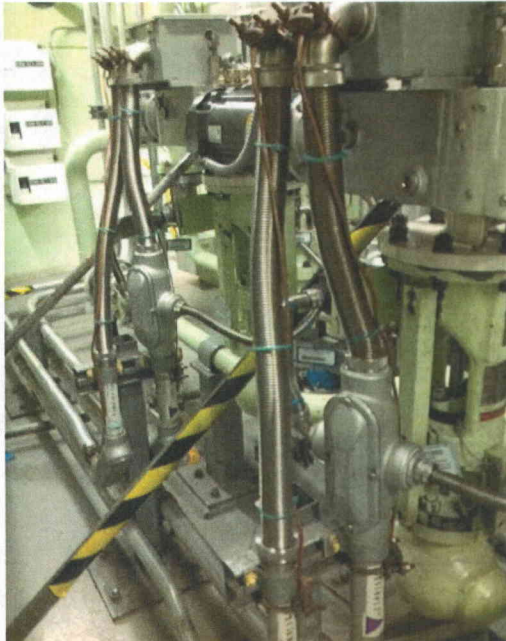
File Name: 2-64-1-2-25.jpeg Description: View of Attached Lines
