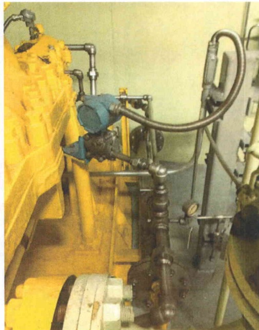
File Name: 2-64-4-2-23.jpeg Description: View of Attached Lines
