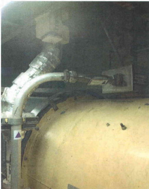
File Name: 2-64-10-2-16.jpeg Description: View of Attached Lines
