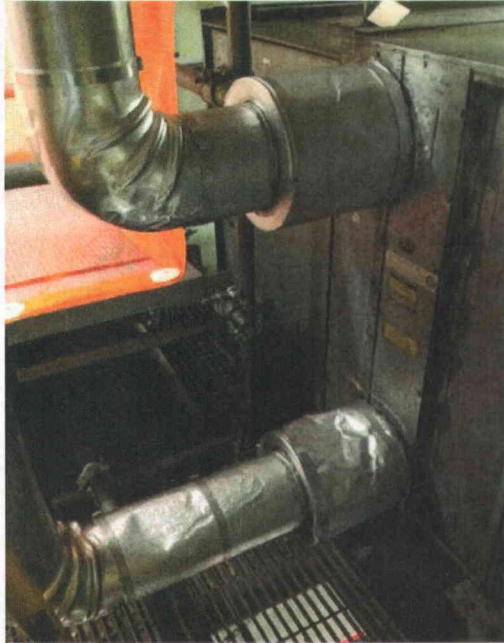
File Name: 2-63-2-2-25.jpeg Description: View of Attached Piping
