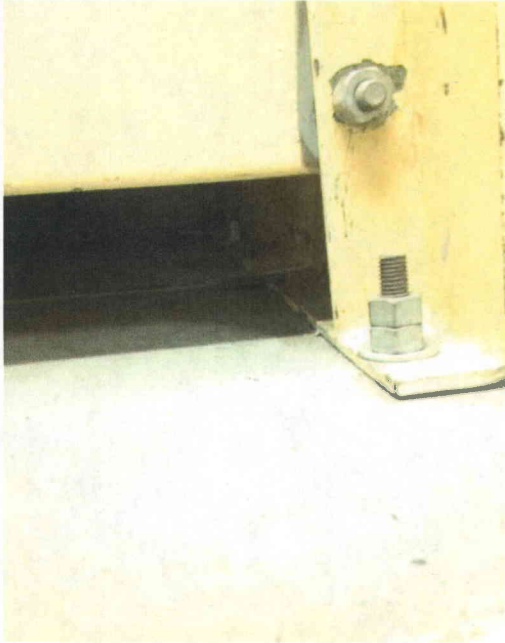
File Name: 2-63-10-2-16.jpeg Description: View of Fan Support Bolts
