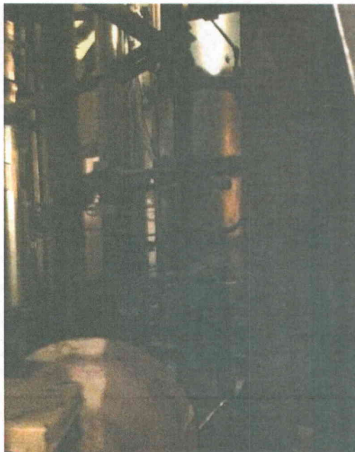
File Name: 2-62-6-2-19.jpeg Description: View of Piping Support
