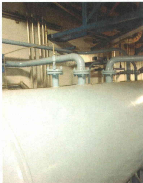
File Name: 2EGF-TK22A(4).jpg Description: View of Attached Lines
