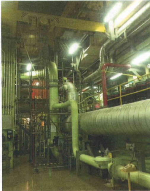
File Name: 2-94-4-2-01.jpeg Description: View of Monorail Crane in Area
