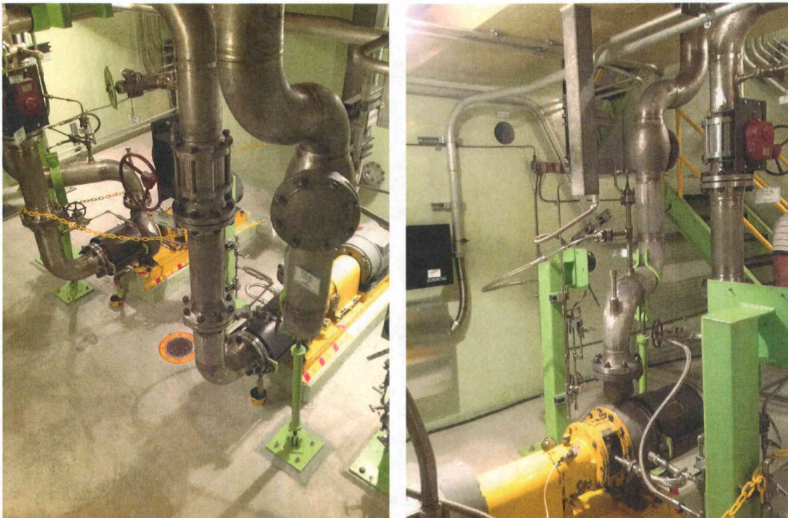
Figure 6-3: View of piping system between Heat Exchangers and Pumps in the SFP area.
