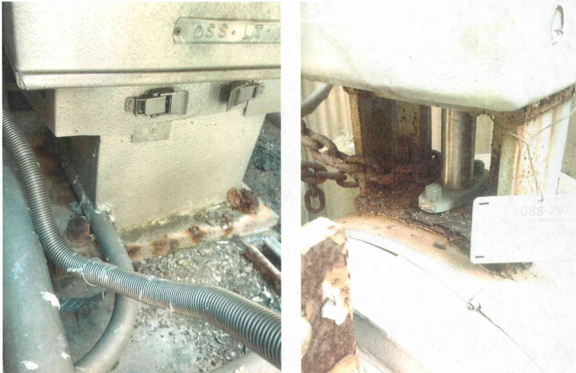
Figure 6-2: Corrosive condition found for Yard components
