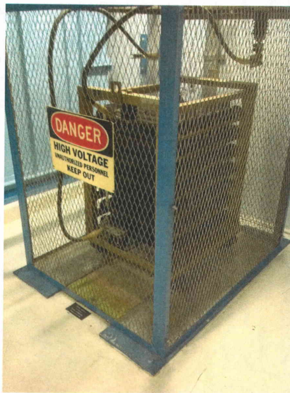
Figure 6-5: Emergency Diesel Generator Ground Resistor 2EGS-GR2-1
