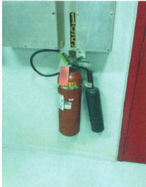
File Name: 1-67-1-4-22.jpeg Description: View of nearby fire extinguisher
