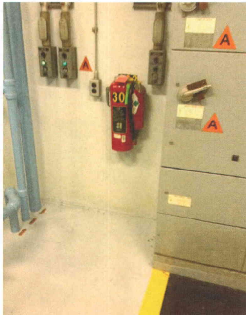
File Name: 1-66-1-4-20.jpeg Description: View of nearby fire extinguisher
