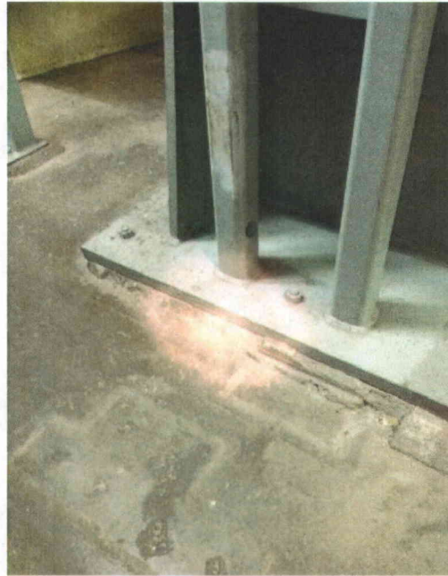
File Name: 1-69-1-4-32.jpeg Description: Spalled grout on main steam support, not significant
