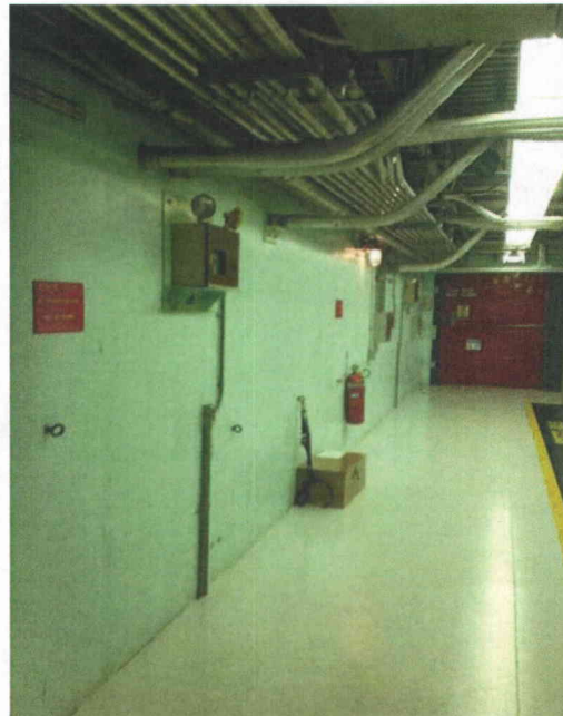
File Name: 1-69-1-4-26.jpeg Description: View of unrestrained fire extinguisher, and properly secured box.
