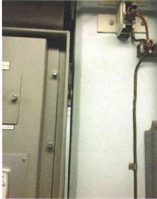
File Name: 1-67-1-4-25.jpeg Description: Gap of 1" between VITBUS 1 and wall judged adequate
