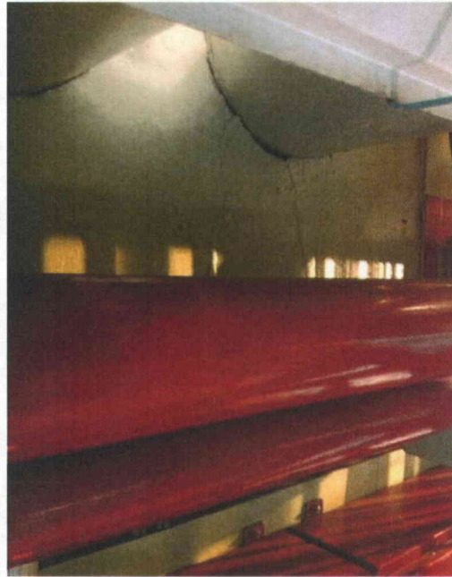
File Name: 1-75-1-4-38.jpeg Description: Wall with potential cracking, east wall, judged not significant
