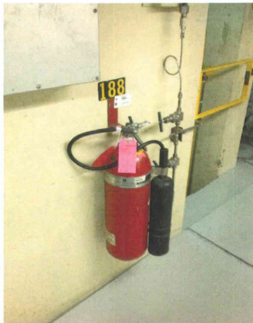
File Name: 1-66-1-4-58.jpeg Description: Fire extinguisher
