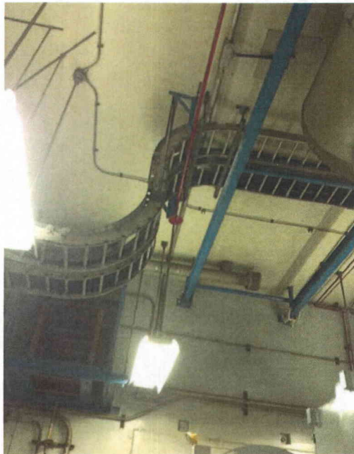
File Name: 1-70-1-4-22.jpeg Description: Fire pipe in proximity of cable tray, is a co2 line
