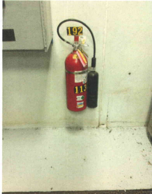
File Name: 1-67-1-4-20.jpeg Description: View of nearby fire extinguisher
