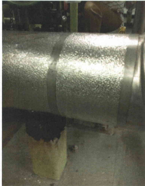
File Name: 1-65-1-4-38.jpeg Description: Noted minor corrosion in area
