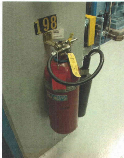
File Name: 1-68-1-4-22.jpeg Description: View of nearby fire extinguisher
