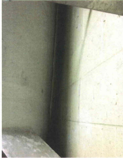
File Name: 1-65-1-4-42.jpeg Description: SI TK 2 approximately 3 inches from block wall. Judged not a concern.
