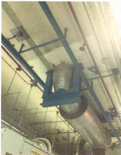
File Name: 1-68-1-4-20.jpeg Description: Soot on ceiling indicates possible exhaust leak inside building
