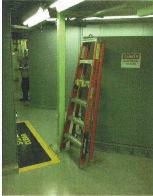
File Name: 1-65-1-4-60.jpeg Description: Poorly secured ladder at ladder station 34
