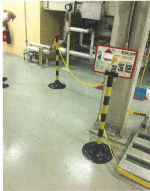
File Name: 1-65-4-4-60.jpeg Description: Unsecured poles, not heavy significant
