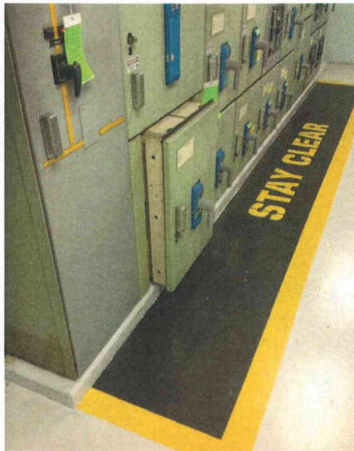
File Name: 1-66-1-4-26.jpeg Description: SUB STA 1-9 BUS 1P, with un-racked breaker
