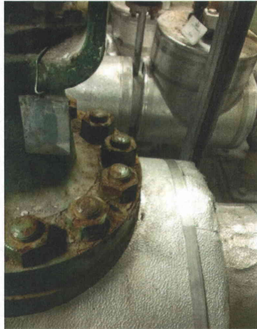
File Name: 1-71-1-4-38.jpeg Description: Noted corrosion in area, CR-2012-13970 initiated
