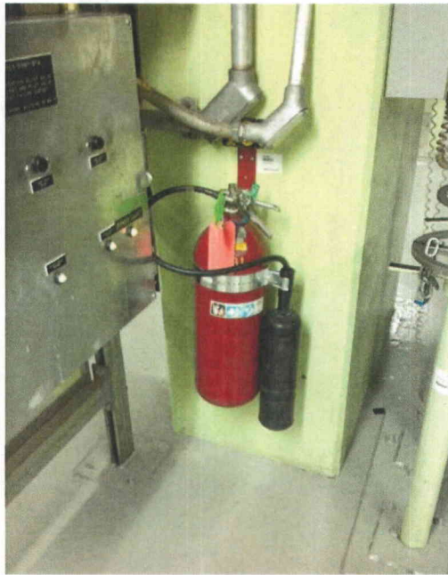
File Name: 1-66-1-4-60.jpeg Description: Fire extinguisher unsecured in area
