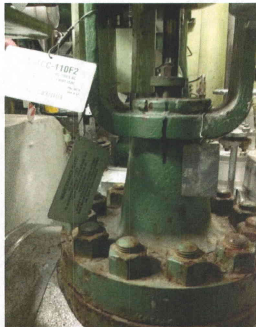
File Name: 1-70-1-4-38.jpeg Description: Noted corrosion in area, CR-2012-13970 initiated
