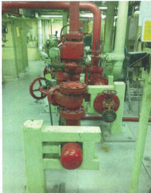
File Name: 1-60-1-4-45.jpeg Description: Fire system identified to be adequately supported.
