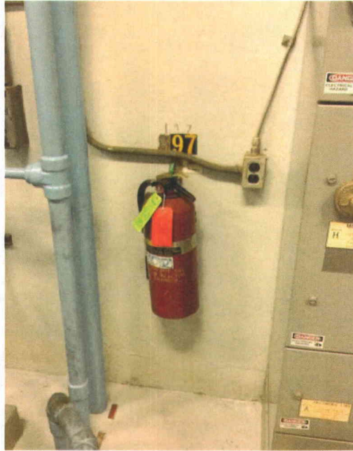
File Name: 1-65-1-4-22.jpeg Description: View of nearby fire extinguisher
