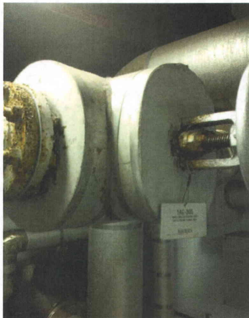
File Name: 1-66-1-4-50.jpeg Description: Corroded valve identified. CR-2012-13972 issued to address this condition.
