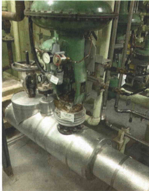
File Name: 1-67-1-4-38.jpeg Description: Noted minor corrosion in area
