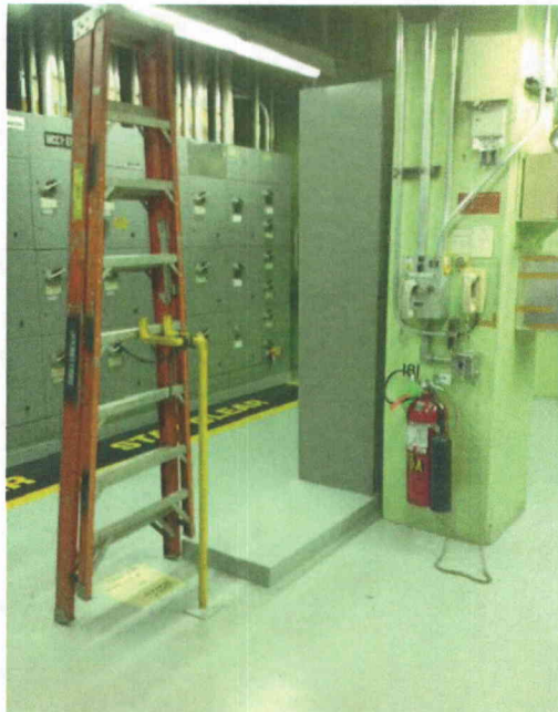
File Name: 1-67-1-4-23.jpeg Description: Fire extinguisher and loose ladder in area
