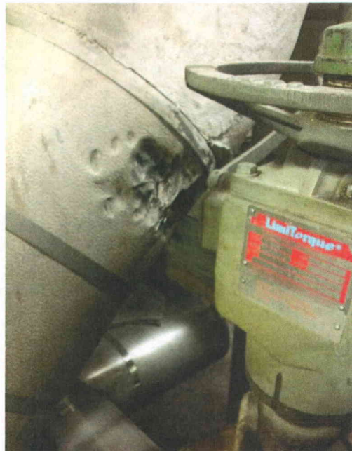
File Name: 1-70-1-4-32.jpeg Description: Insulation damage believed to be due to valve servicing MOV 1 MS 105
