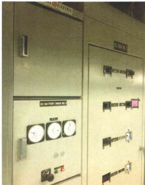
File Name: 1-70-1-4-25.jpeg Description: DC-SWGR-3 and DC-SWBD-3 are bolted together,
