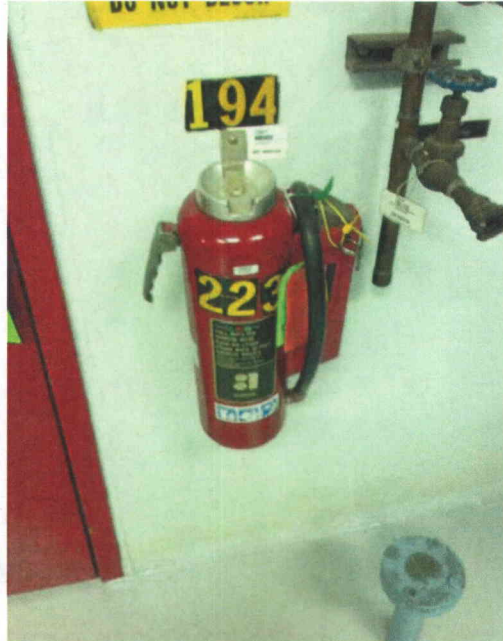
File Name: 1-65-1-4-20.jpeg Description: View of nearby fire extinguisher
