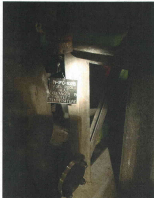
File Name: 1-70-3-4-60.jpeg Description: Temperature gage near HVAC supports judged acceptable
