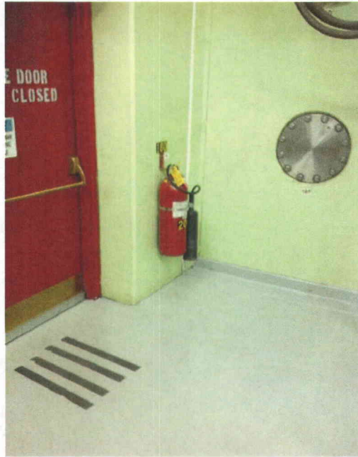
File Name: 1-68-1-4-23.jpeg Description: Fire extinguisher in area
