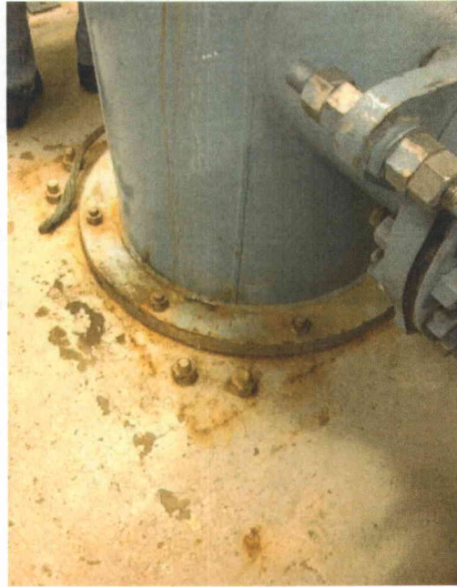
File Name: 1-65-1-4-28.jpeg Description: Surface rust on pump 1WR P 1B not an issue
