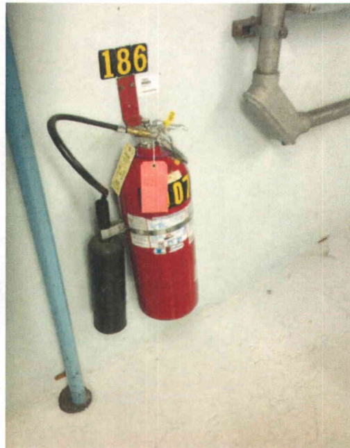
File Name: 1-65-1-4-50.jpeg Description: View of fire extinguisher located in the area
