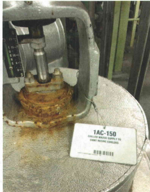
File Name: 1-69-1-4-38.jpeg Description: Noted corrosion in area, CR-2012-13971 initiated
