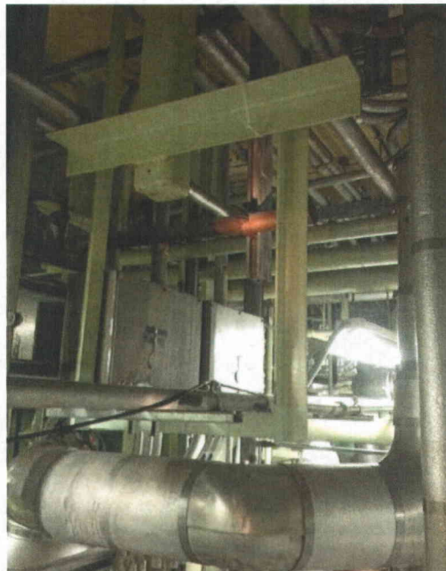
File Name: 1-68-1-4-38.jpeg Description: Noted minor corrosion in area
