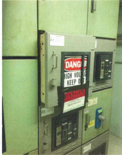
File Name: 1-67-1-4-26.jpeg Description: SUB STA 1-9 BUS 1P, with un-racked breaker
