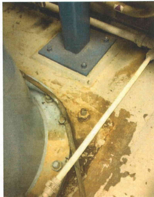
File Name: 1-68-1-4-29.jpeg Description: Corroded bolt near pump. Bolt hold nothing
