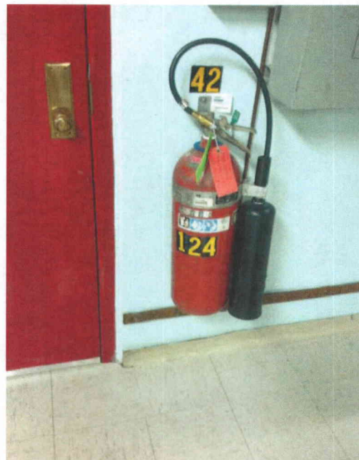
File Name: 1-66-5-4-60.jpeg Description: Fire extinguisher
