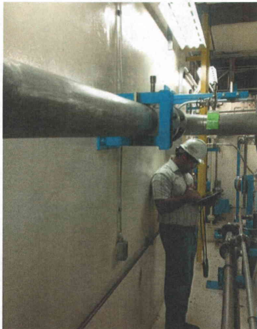
File Name: 1-60-1-4-17.jpeg Description: Pipe is not restrained in the longitudinal direction
