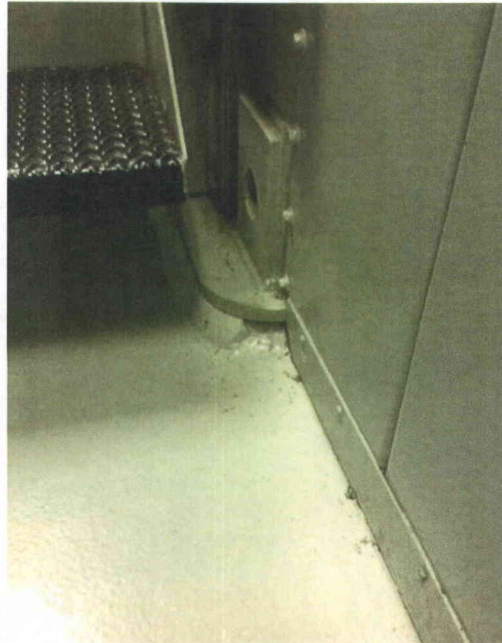
File Name: 1-69-1-4-22.jpeg Description: Minor spalling underneath diesel generator
