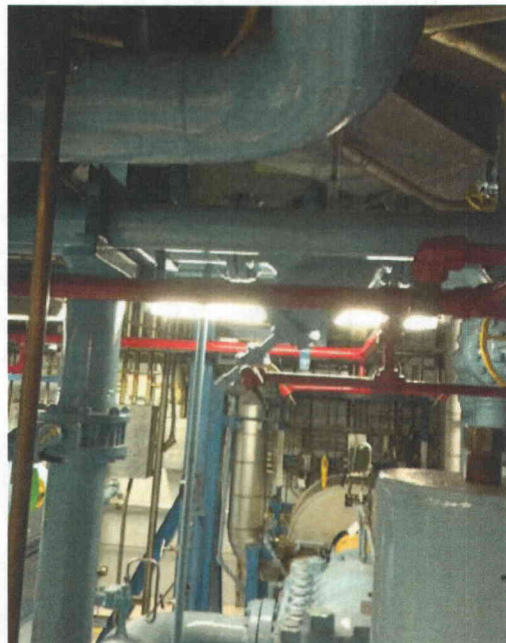
File Name: 1-72-1-4-50.jpeg Description: Fire pipe system appears secure, no risk identified.
