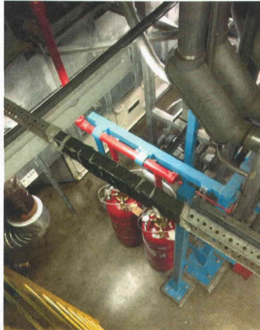
File Name: 1-65-1-4-06.jpeg Description: Fire suppression system rugged
