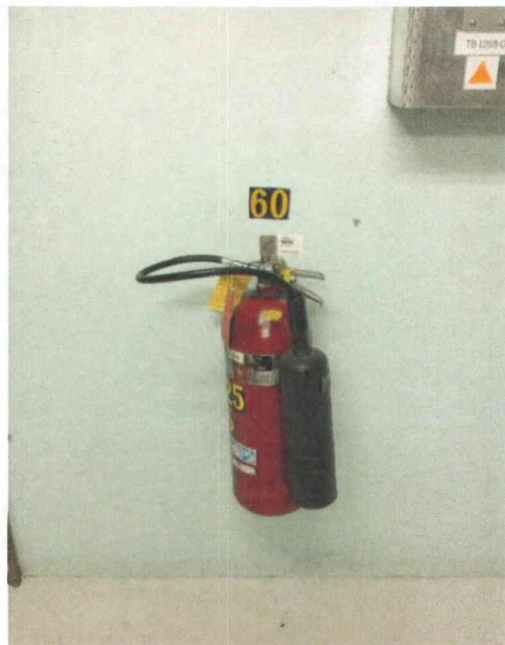
File Name: 1-72-1-4-25.jpeg Description: View of nearby fire extinguisher
