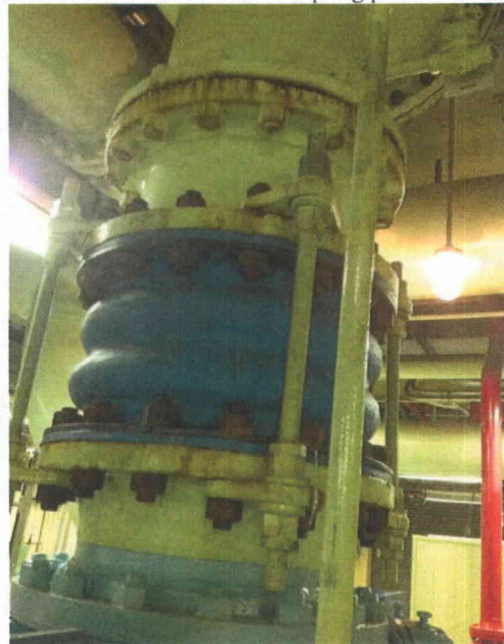
File Name: 1-68-1-4-46.jpeg Description: Surface corrosion, judged a non issue
