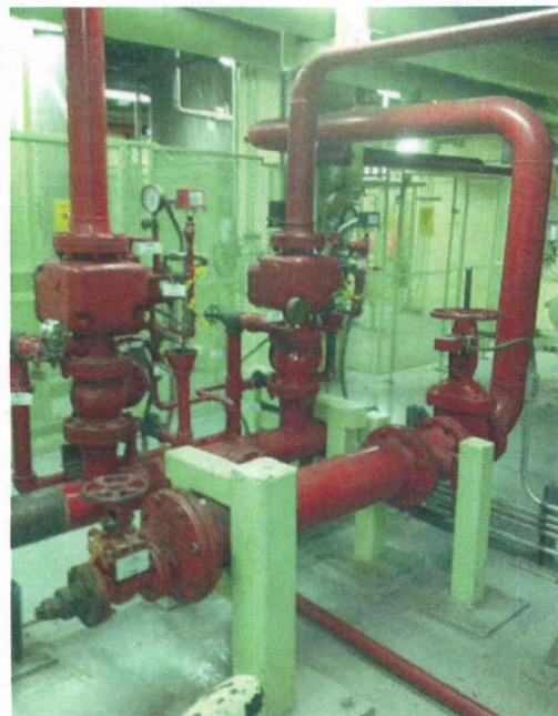
File Name: 1-60-1-4-46.jpeg Description: Fire system is rugged.
