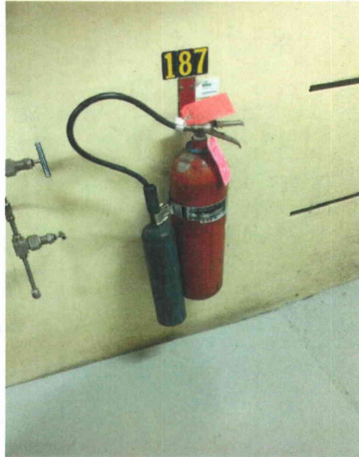
File Name: 1-67-1-4-58.jpeg Description: Fire extinguisher
