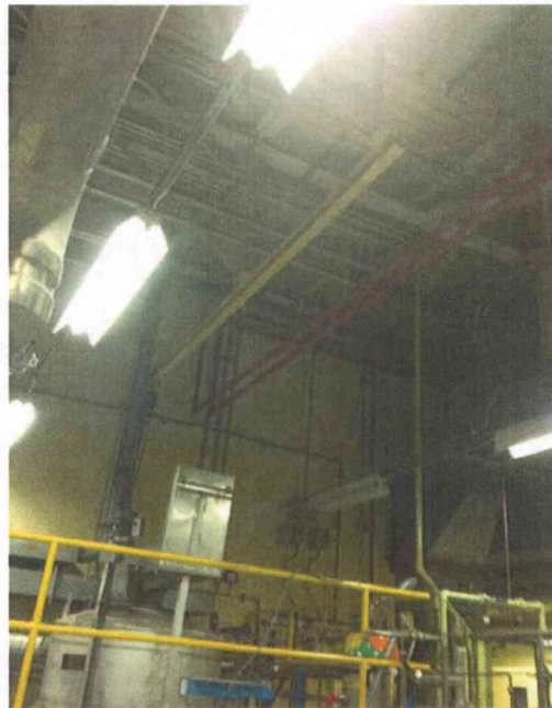
File Name: 1-60-4-4-60.jpeg Description: Fire pipe looks secured judged a non issue
