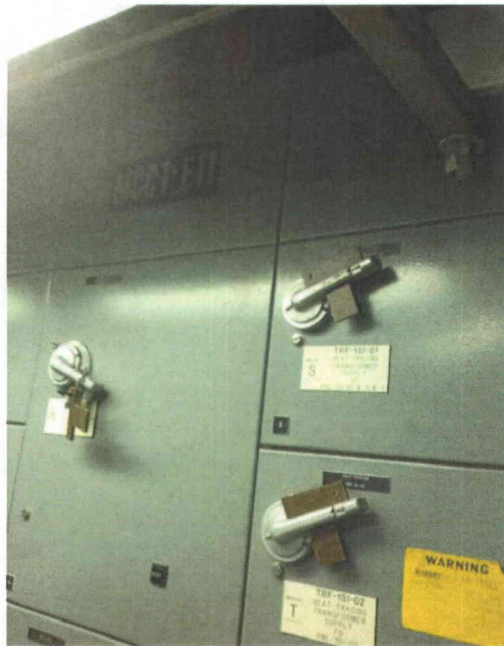
File Name: 1-68-1-4-60.jpeg Description: MCC-E11 and nearby cable tray
