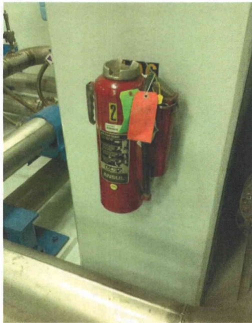
File Name: 1-66-1-4-22.jpeg Description: View of nearby fire extinguisher
