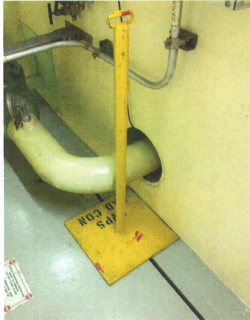
File Name: 1-65-1-4-41.jpeg Description: Loose pole could impact
