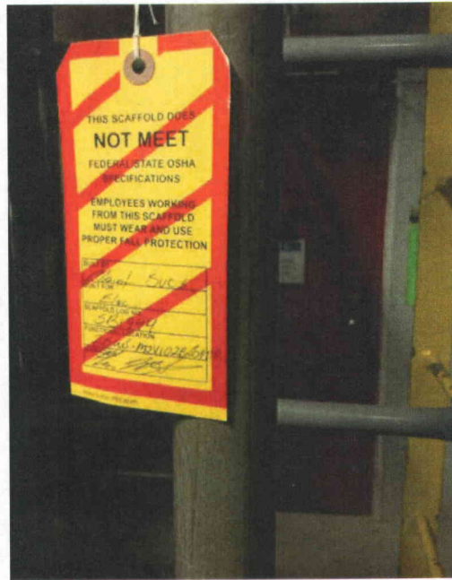
File Name: 1-67-1-4-29.jpeg Description: Scaffold deficient tag
