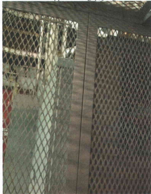
File Name: 1-67-1-4-34.jpeg Description: No connection between cage and transformer, approx 2 in gap, judged a non issue.
