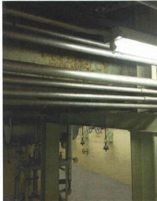
File Name: 1-71-1-4-43.jpeg Description: Surface corrosion identified on large pipes. Judged not a concern.
