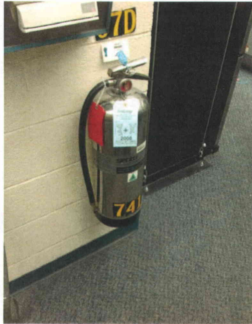
File Name: 1-65-1-4-18.jpeg Description: Fire extinguisher near computer room
