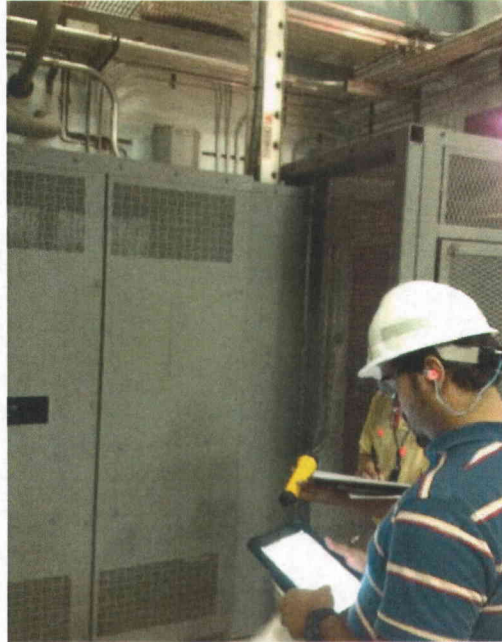
File Name: 1-66-1-4-34.jpeg Description: No connection between cage and transformer, approx 2 in gap, judged a non issue.
