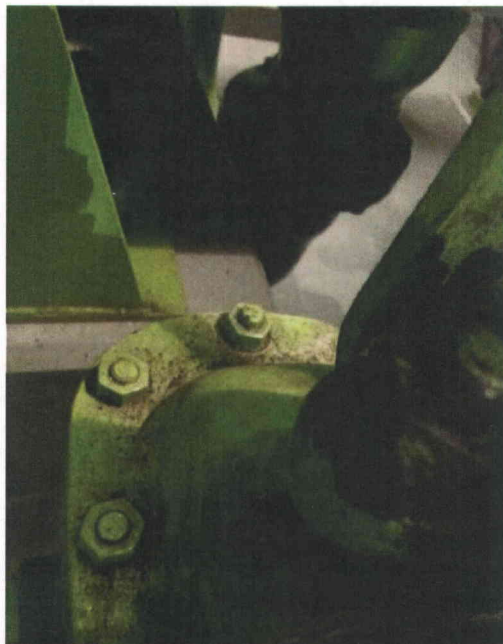
File Name: 1-65-3-4-60.jpeg Description: Nut at 12 o'clock not engaged on underside. Judged acceptable.
