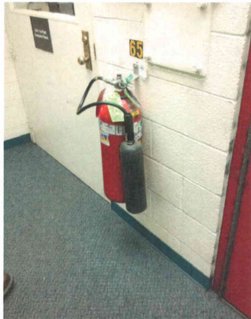
File Name: 1-60-1-4-18.jpeg Description: Fire extinguisher near computer room
