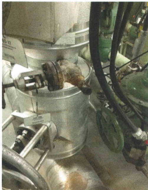
File Name: 1-66-1-4-38.jpeg Description: Noted minor corrosion in area
