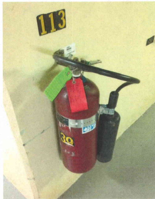
File Name: 1-60-1-4-41.jpeg Description: Fire extinguisher in area
