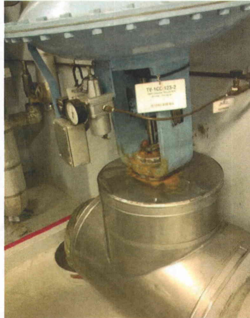
File Name: 1-67-1-4-50.jpeg Description: Corroded valve identified. CR-2012-13972 issued to address this condition.
