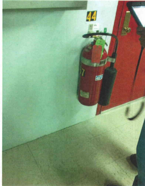
File Name: 1-65-5-4-60.jpeg Description: Fire extinguisher
