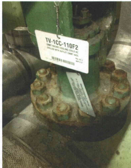
File Name: 1-72-1-4-38.jpeg Description: Noted corrosion in area, CR-2012-13970 initiated
