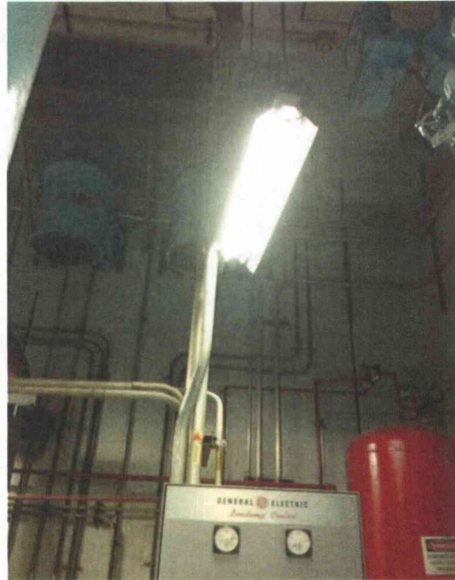
File Name: 1-65-1-4-27.jpeg Description: Light above Cabinet PNL 1FP1. Judged non-damaging.
