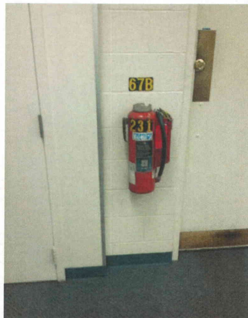
File Name: 1-68-1-4-18.jpeg Description: Fire extinguisher near computer room
