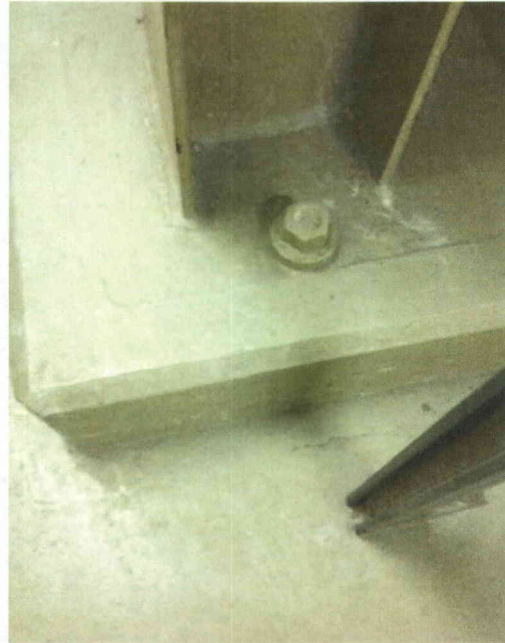
File Name: 1-65-1-4-14.jpeg Description: One anchor bolt not fully engaged on north post by half a thread.
