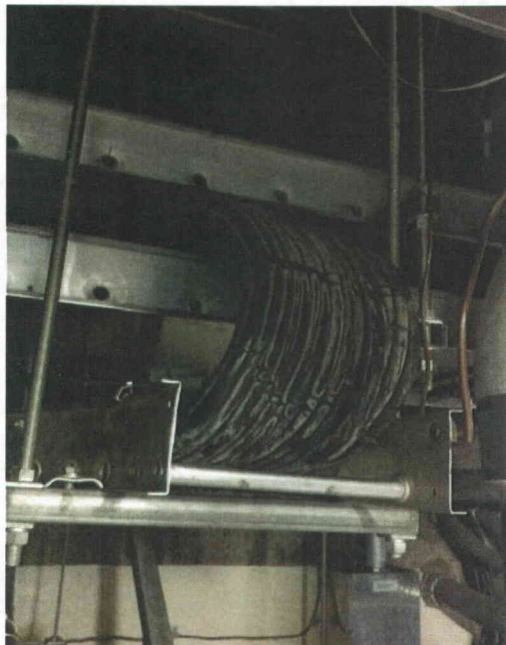
File Name: 1-66-1-4-06.jpeg Description: Cable trays in area full, but not overflowing
