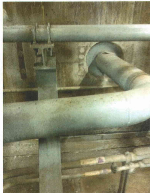
File Name: 1-75-1-4-32.jpeg Description: View of pipe going into containment building with nearby knee brace located on the floor of Safeguards Building. Interaction due to differential motion judged not a concern.
