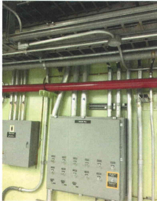
File Name: 1-65-1-4-23.jpeg Description: Fire pipe over panel is rigidly supported
