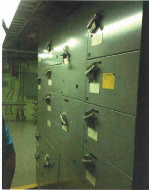
File Name: 1-69-1-4-60.jpeg Description: MCC-E11 and nearby cable tray
