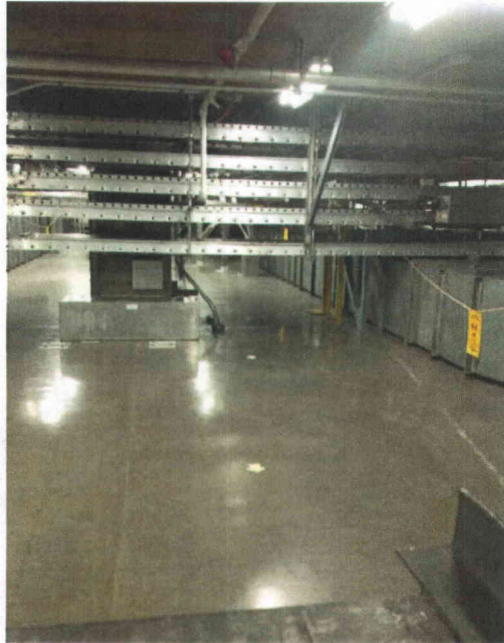
File Name: 1-65-1-4-56.jpeg Description: General view of cable trays in the area
