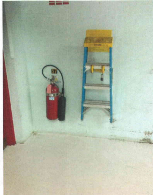
File Name: 1-70-1-4-26.jpeg Description: View of unrestrained fire ext, ladder is properly secured.
