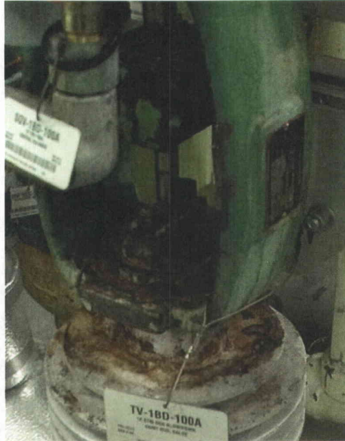
File Name: 2-63-1-1-38.jpeg Description: Slight corrosion identified on valve
