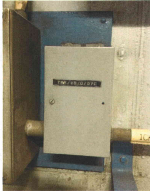
File Name: 2-73-1-1-29.jpeg Description: View of tag ID for related instrumentation panel
