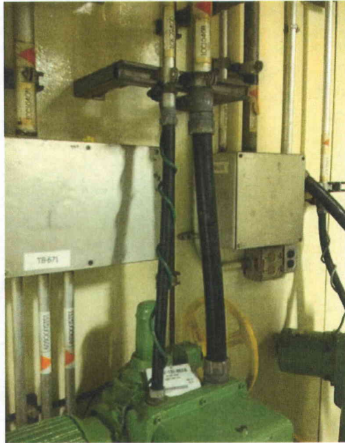
File Name: 2-63-2-1-58.jpeg Description: View of flexible attached lines
