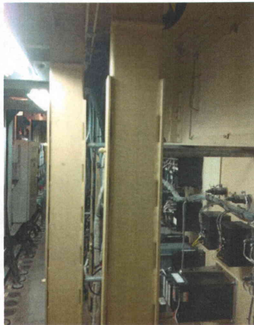
File Name: 2-64-6-1-18.jpeg Description: View of mid posts inside panel providing support to front mounting panel
