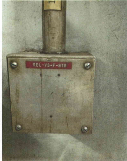
File Name: 2-63-4-1-28.jpeg Description: View of tag ID for related instrumentation panel
