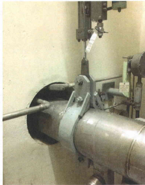
File Name: 2-63-1-1-10.jpeg Description: View of hung support for attached pipe line
