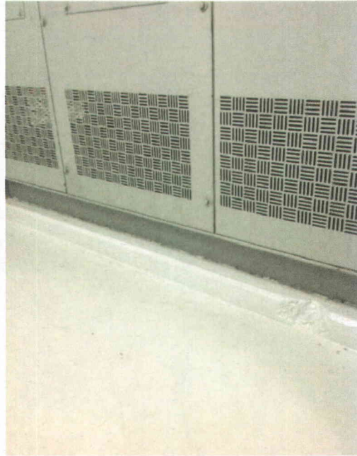
File Name: 2-63-7-1-26.jpeg Description: General view of base mounting frame
