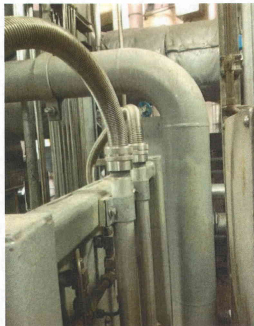
File Name: 2-64-7-1-32.jpeg Description: View of flexible attached lines
