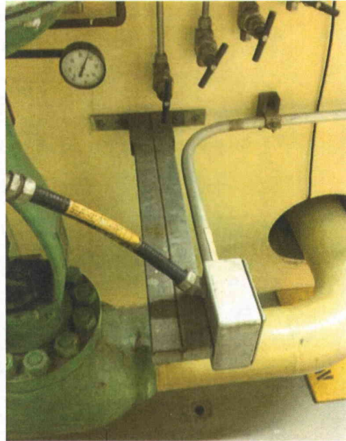
File Name: 2-63-1-1-41.jpeg Description: View of flexible attached lines
