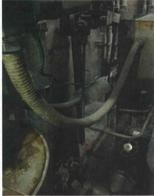
File Name: 2-63-1-1-32.jpeg Description: View of flexible attached lines
