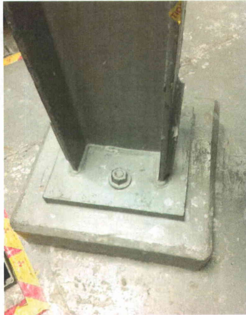
File Name: 2-63-1-1-42.jpeg Description: Typical view of base anchorage configuration for each leg support
