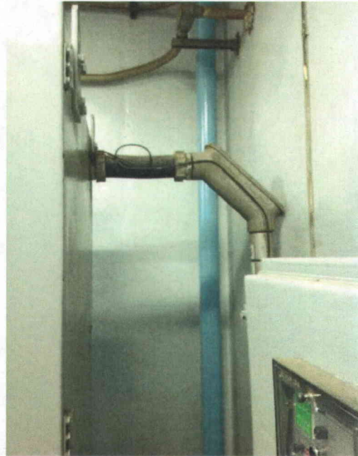
File Name: 2-63-2-1-21.jpeg Description: View of flexible attached line
