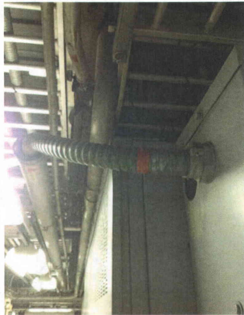
File Name: 2-64-12-1-25.jpeg Description: View of flexible attached line
