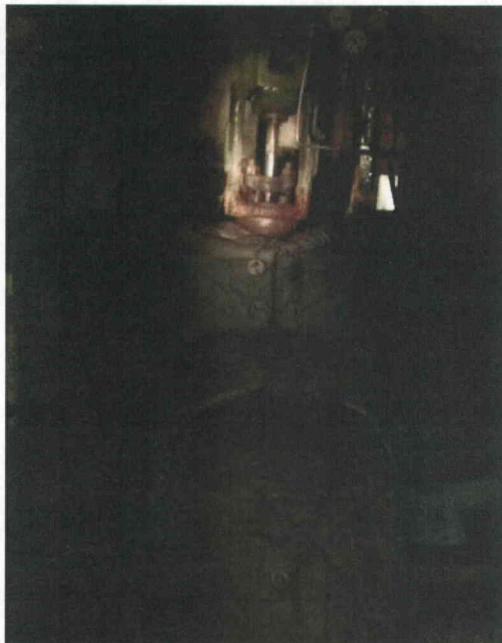
File Name: 2-62-3-1-32.jpeg Description: View of valve on main pipe line
