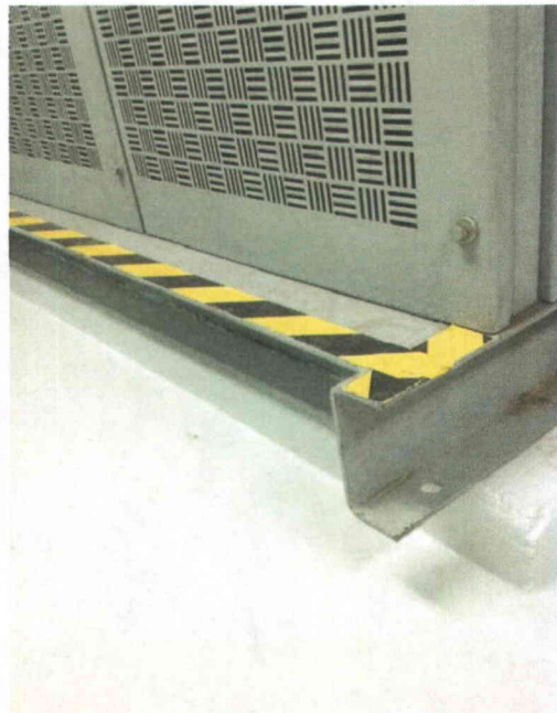
File Name: 2-64-7-1-26.jpeg Description: General view of base mounting frame
