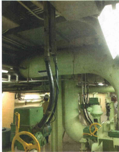
File Name: 2-63-2-1-43.jpeg Description: View of flexible attached lines
