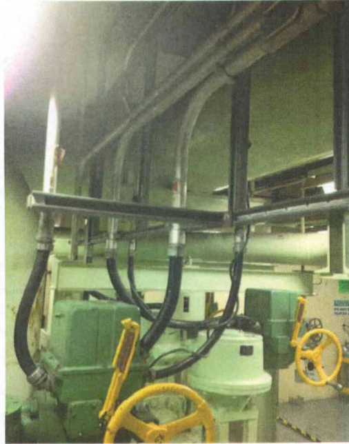
File Name: 2-63-3-1-43.jpeg Description: View of flexible attached lines
