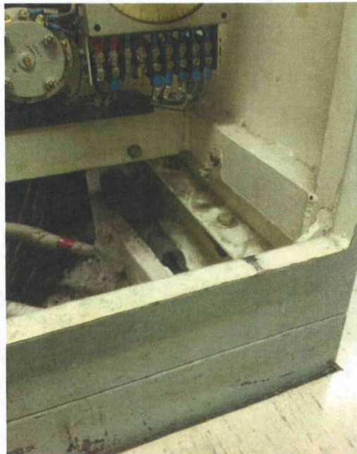
File Name: 2-64-3-1-49.jpeg Description: View of anchorage between cabinet housing and base frame
