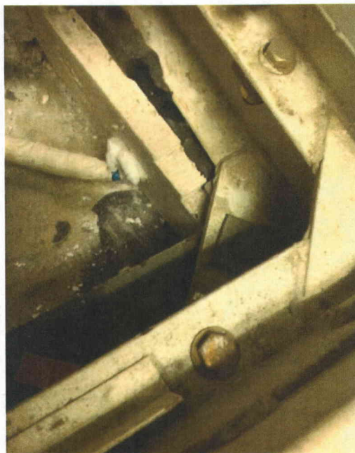
File Name: 2-73-3-1-49.jpeg Description: View of anchorage between base frame and floor beam
