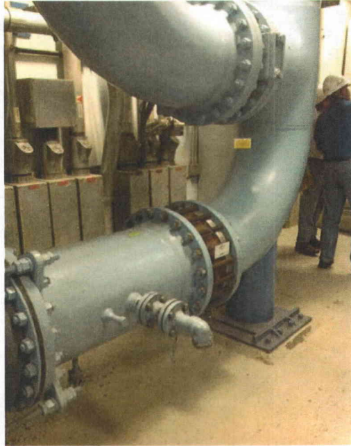
File Name: 2-63-4-1-27.jpeg Description: View of valve location on main line
