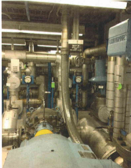
File Name: 2-63-7-1-50.jpeg Description: View of flexible attached lines
