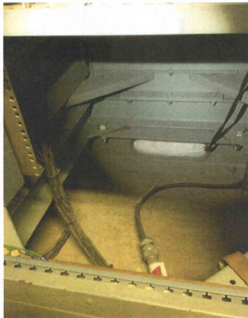
File Name: 2-64-1-1-49.jpeg Description: View of base frame connection to floor wide flange beams
