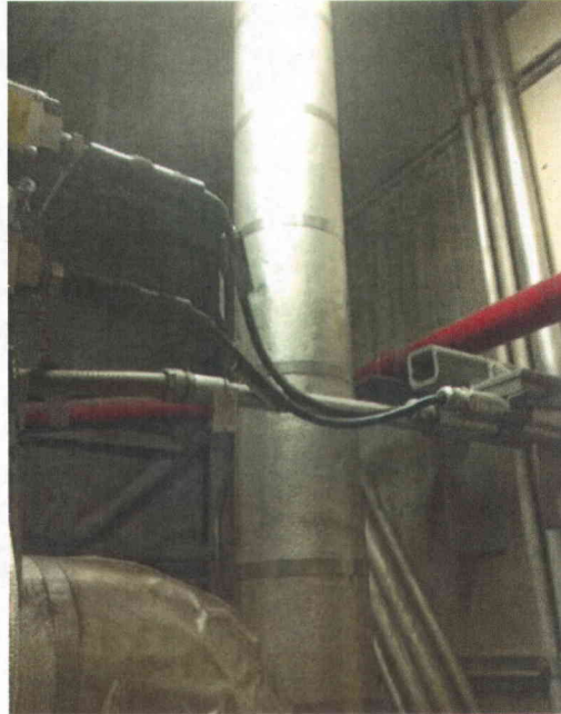
File Name: 2-63-6-1-32.jpeg Description: View of flexible attached lines
