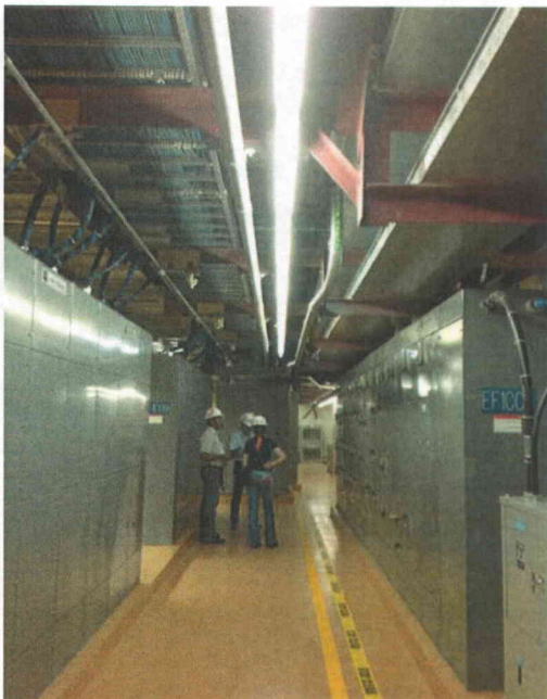
File Name: 1-75-1-1-06.jpeg Description: View of single row of fluorescent lights
