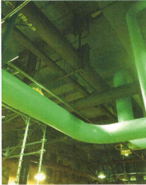
File Name: 1-76-3-1-20.jpeg Description: View of overhead piping restraints
