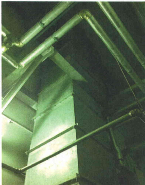
File Name: 1-60-2-1-15.jpeg Description: View of HVAC support
