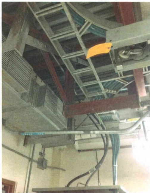
File Name: 1-60-1-1-02.jpeg Description: Rigid support cable tray and HVAC
