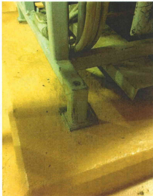
File Name: 1-74-1-1-01.jpeg Description: Air dryer rack (1P52-D003B) missing anchorage (similar issue 1P52-D003A)
