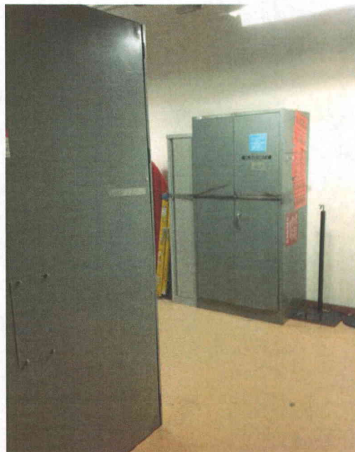
File Name: 1-69-1-1-06.jpeg Description: Tool locker not restrained behind bus/breakers
