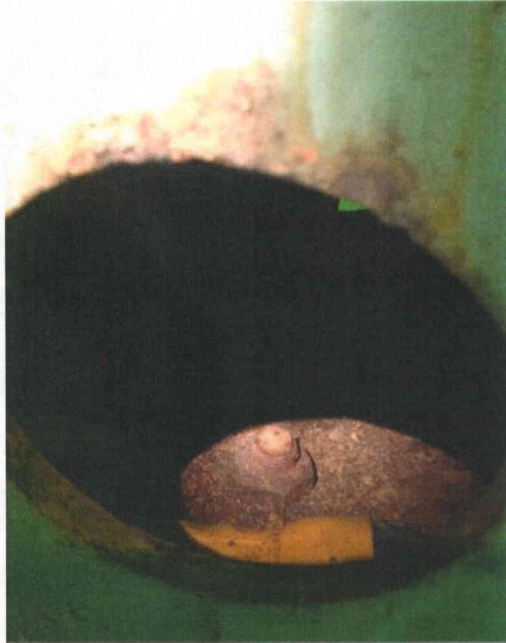
File Name: 1-71-3-1-20.jpeg Description: View of corroded bolt located north east end of 1P46B001B
