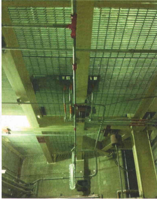
File Name: 1-65-2-1-16.jpeg Description: View of fire protection piping and overhead grating
