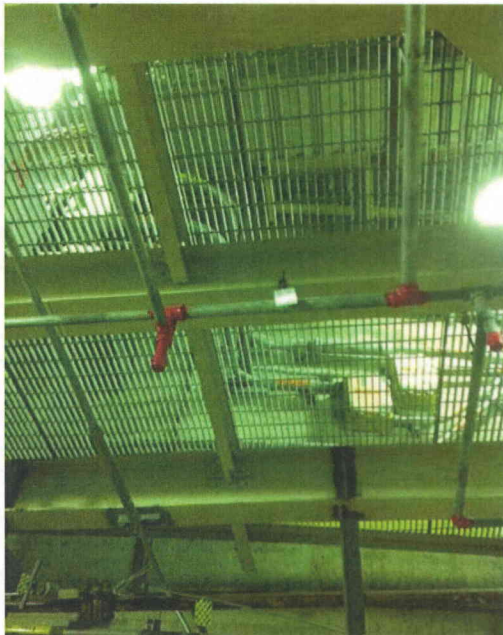
File Name: 1-60-2-1-16.jpeg Description: Friction clip on fire protection piping
