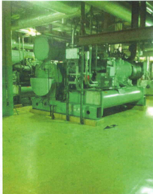
File Name: 1-77-3-1-20.jpeg Description: General view of chillers
