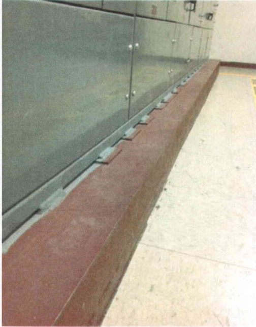
File Name: 1-65-2-1-06.jpeg Description: View of 1R24-S0029 welded shims
