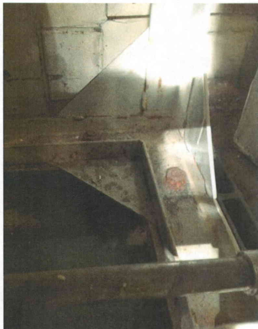
File Name: 1-71-1-1-13.jpeg Description: Mild corrosion identified in anchorage
