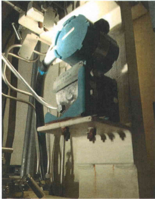
File Name: 1-68-1-1-12.jpeg Description: Surface corrosion identified
