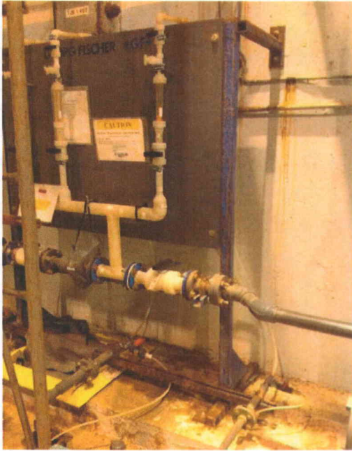
File Name: 1-70-1-1-05.jpeg Description: Surface corrosion identified
