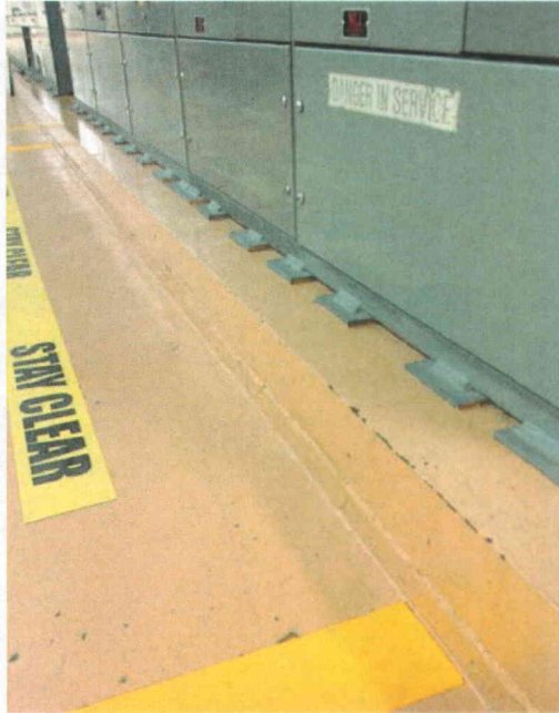
File Name: 1-69-3-1-06.jpeg Description: Welded shims for 1R21-S0019
