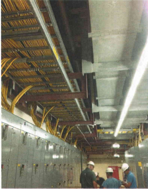
File Name: 1-65-3-1-06.jpeg Description: View of supports for cable trays
