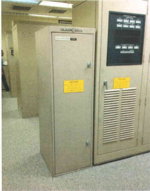
File Name: 1-67-1-1-03.jpeg Description: Cabinet not anchored
