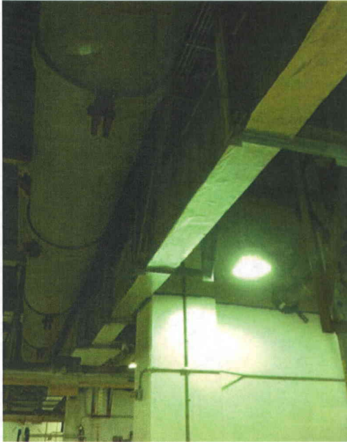
File Name: 1-65-1-1-01.jpeg Description: HVAC rigidly supported
