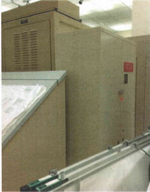
File Name: 1-59-1-1-03.jpeg Description: Supply locker not anchored
