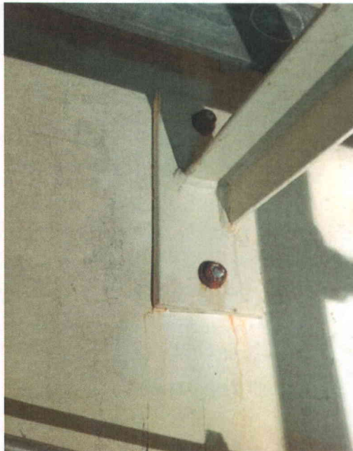
File Name: 1-60-1-1-12.jpeg Description: Surface corrosion identified
