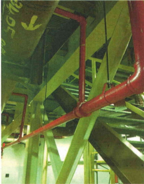
File Name: 1-67-1-1-01.jpeg Description: Rod hung fire protection piping
