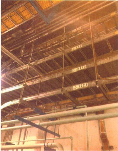
File Name: 1-65-2-1-14.jpeg Description: View of cable trays in the area
