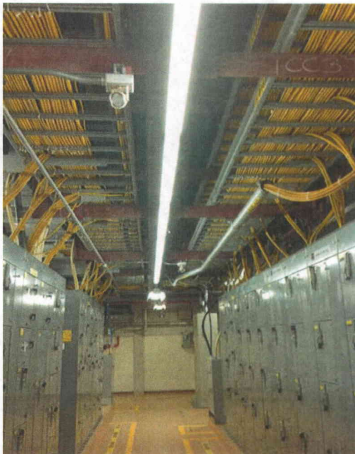
File Name: 1-72-3-1-06.jpeg Description: View of single row of fluorescent lights
