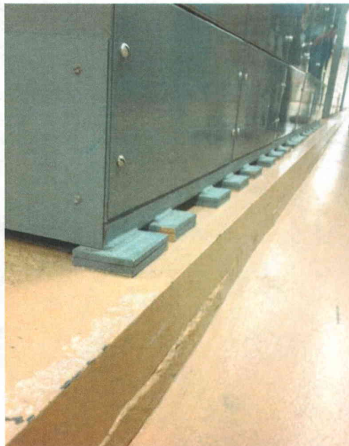
File Name: 1-70-3-1-06.jpeg Description: Welded shims for 0R24-S0035
