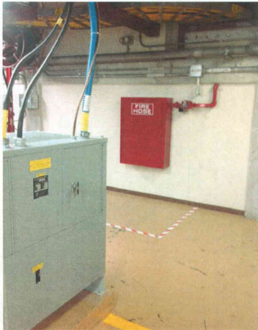
File Name: 1-67-3-1-06.jpeg Description: Fire protection valve near transformer judged to be adequately supported
