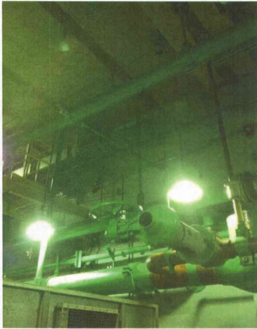
File Name: 1-65-5-1-18.jpeg Description: View of piping in the area
