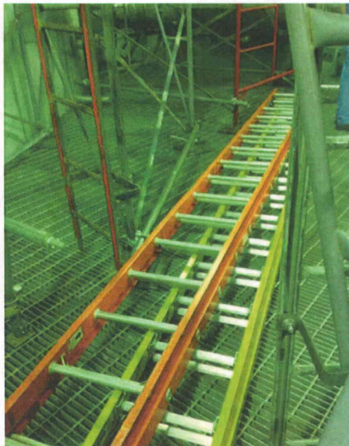
File Name: 1-60-1-1-19.jpeg Description: View of unrestrained ladders not likely to impact components
